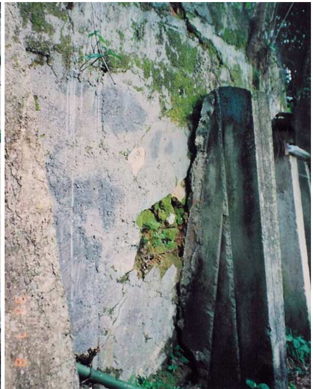
(4) 破裂表層及擋土牆
