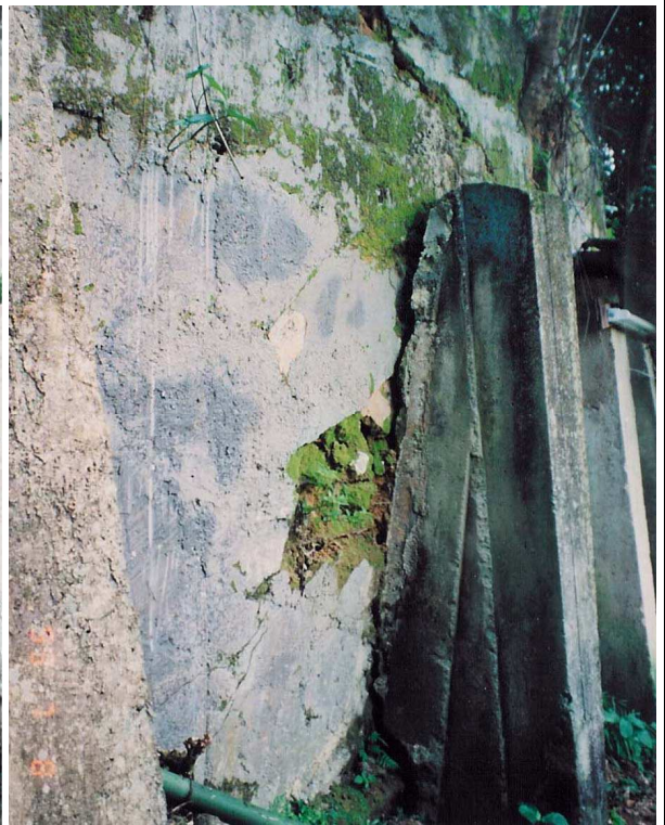
(4) 破裂表層及擋土牆
