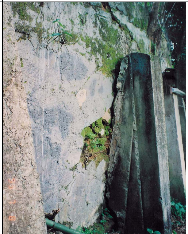
(4) 破裂表層及擋土牆
