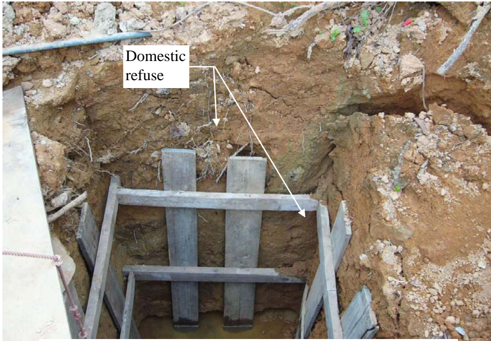
Plate 20 - Trial Pit TP4 Showing Landslide Debris Containing Deformed Domestic Refuse Layers (Photograph taken on 17 October 2005)
