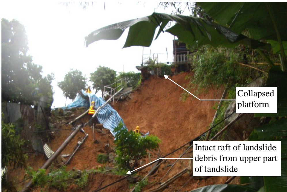
Plate 12 - The Main Scarp and the Southern Flank of the Landslide (Photograph taken on 21 August 2005)
