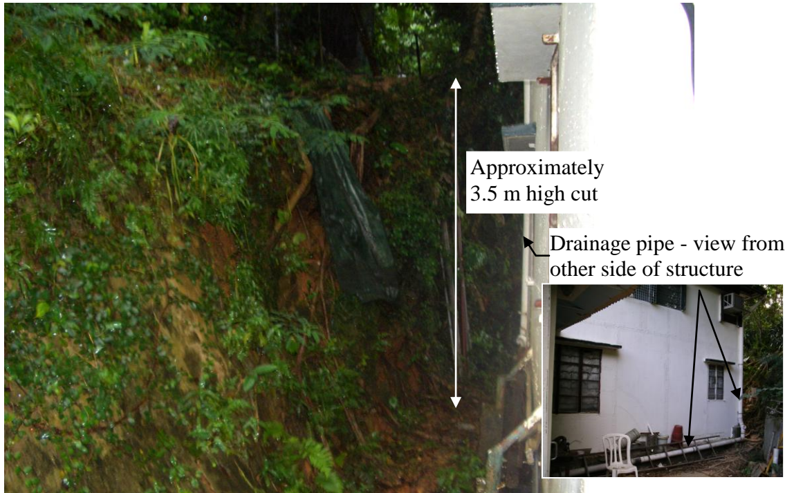
Plate 6 - Drainage Pipe and the Cut Slope behind Registered Squatter Structure No. RTW/4A/388 (Photograph taken on 21 August 2005)
