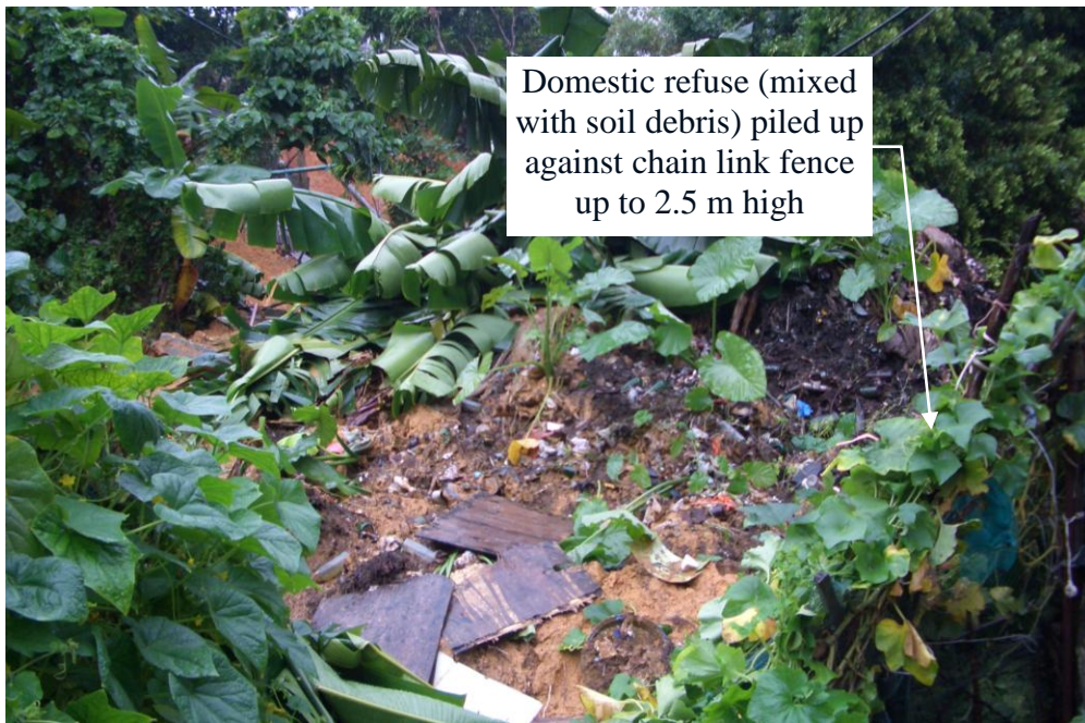
Plate 18 - Domestic Refuse Transported along with the Landslide Debris (Photograph taken on 21 August 2005)
