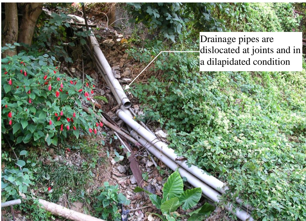
Plate 11 - PVC Drainage Pipes Leading from Squatter Structures Nos. RTW/4A/389, 391-393 (Photograph taken on 6 December 2005)
