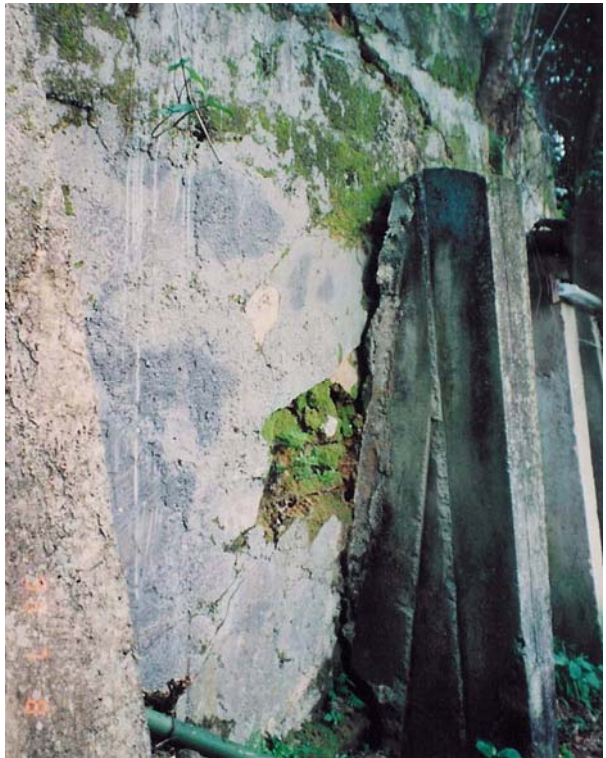
(4) 破裂表層及擋土牆
