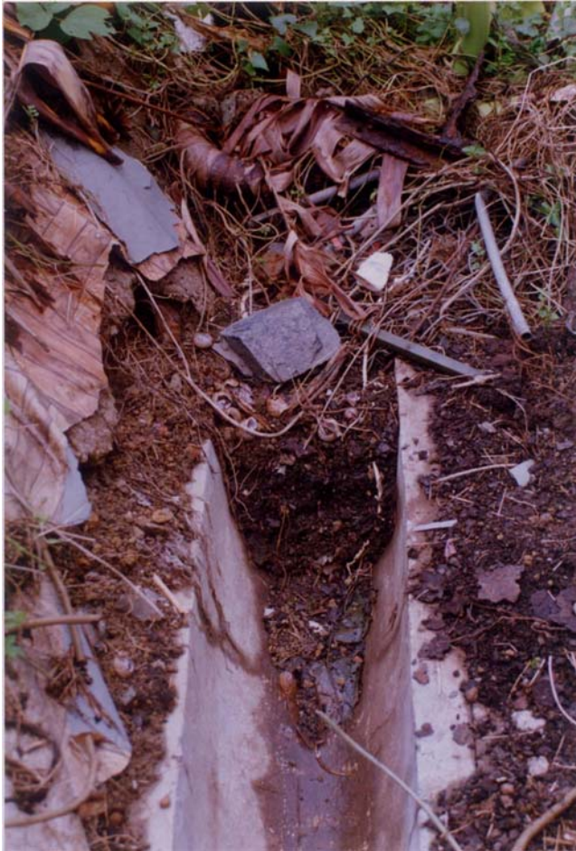
Plate 4 - Blocked Surface Drainage Channel on the Unfailed Section of the Cut Slope (Photograph Taken on 10 October 1995. See Figure 21 for Location)
