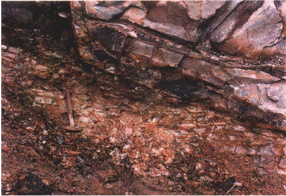
Plate 10 - Kaolinite-rich Altered Tuff at the Unfailed Portion of the Cut Slope to the East of the Landslide (Photograph Taken on 8 October 1995. See Figure 21 for Location)
