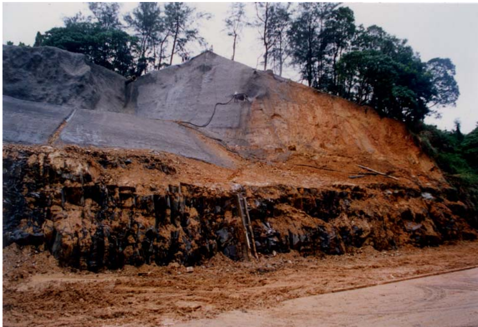
Plate 9 - Rock Face below the Base of the Landslide (Photograph Taken on 31 August 1995. See Figure 21 for Location)
