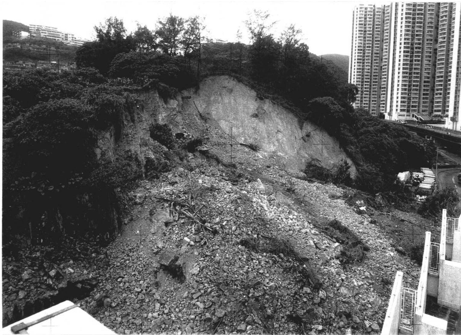
Plate 1 - Photograph of the Landslide Taken in the Morning of 13 August 1995 (See Figure 21 for Location)
