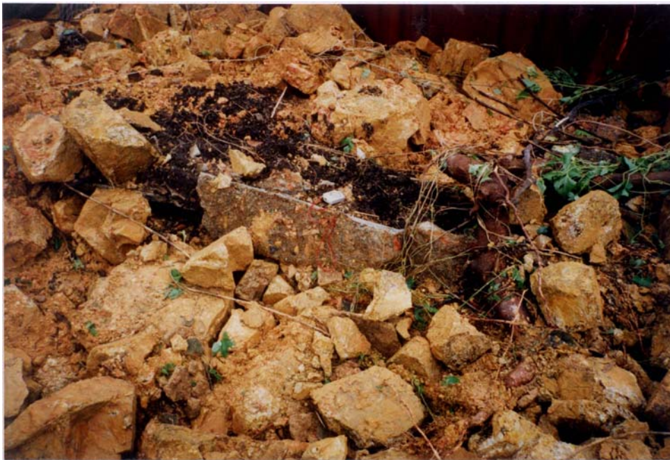
Plate 5 - Blocked Surface Drainage Channel in the Landslide Debris (Photograph Taken on 13 August 1995. See Figure 21 for Location)
