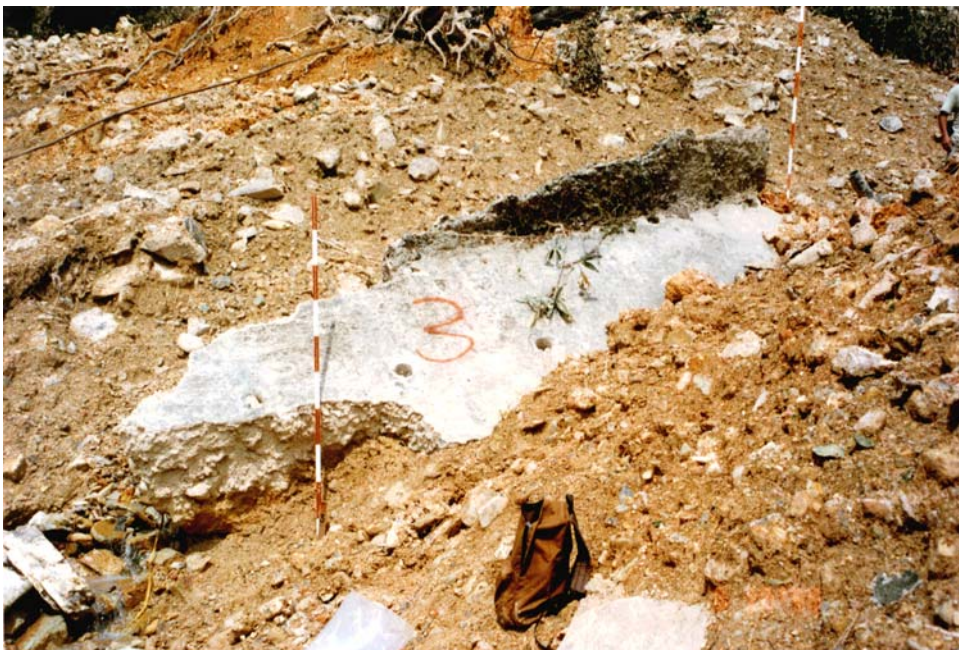
Plate 5 - Retaining Wall Fragment on Lower Part of Landslide Scar
