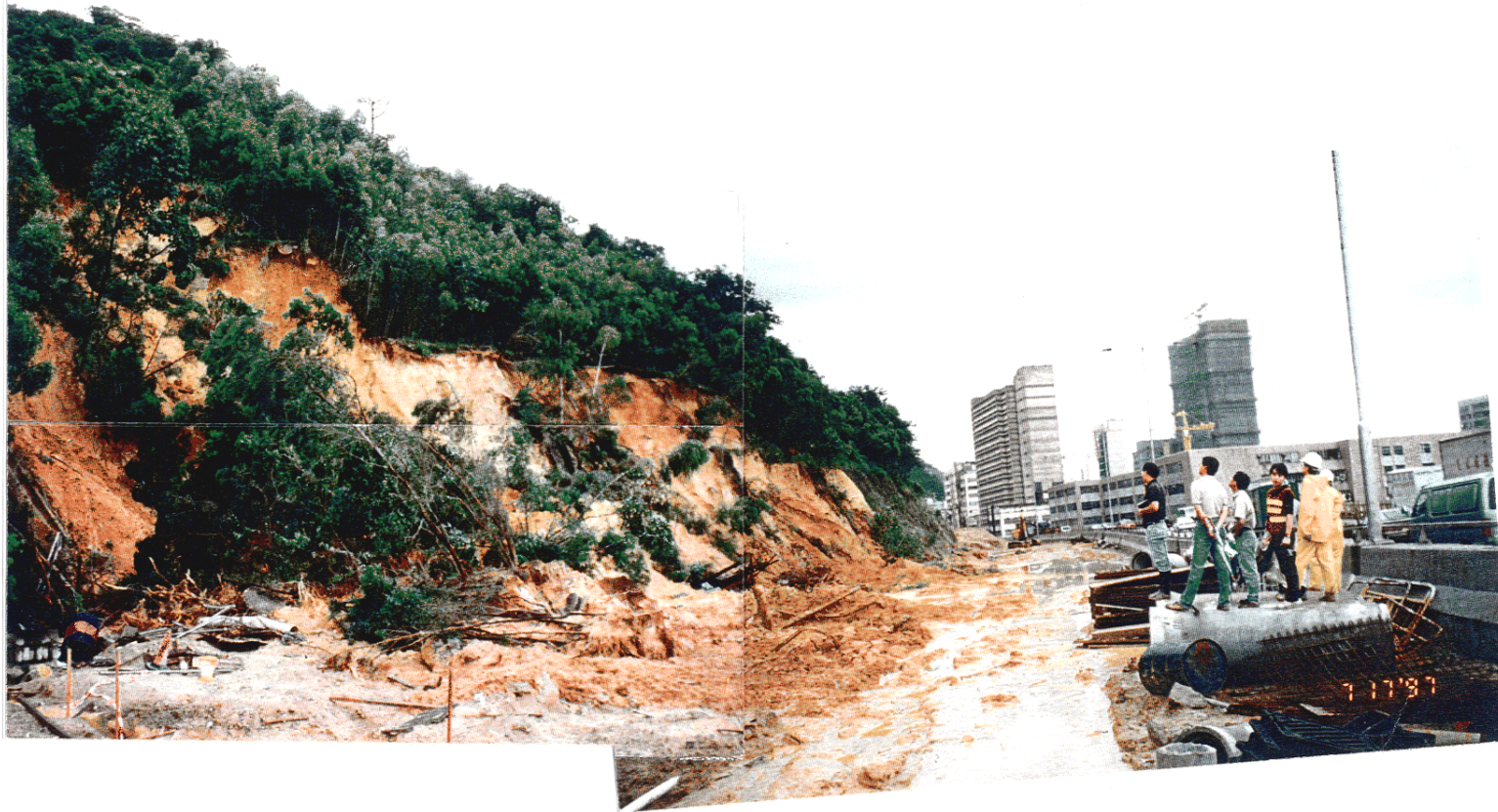
Plate 4 - Photograph of 17 July 1997 Failure (Photograph Taken on 17 July 1997)
