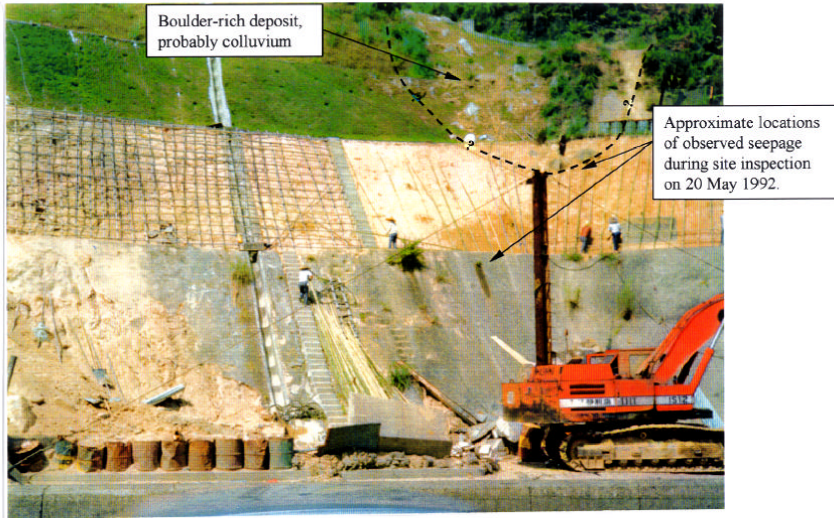
Plate 11 - Photograph of Central Section of Slope No. 11NW-A/C55 During LPM Works (Photograph Taken on 4 October 1991)
