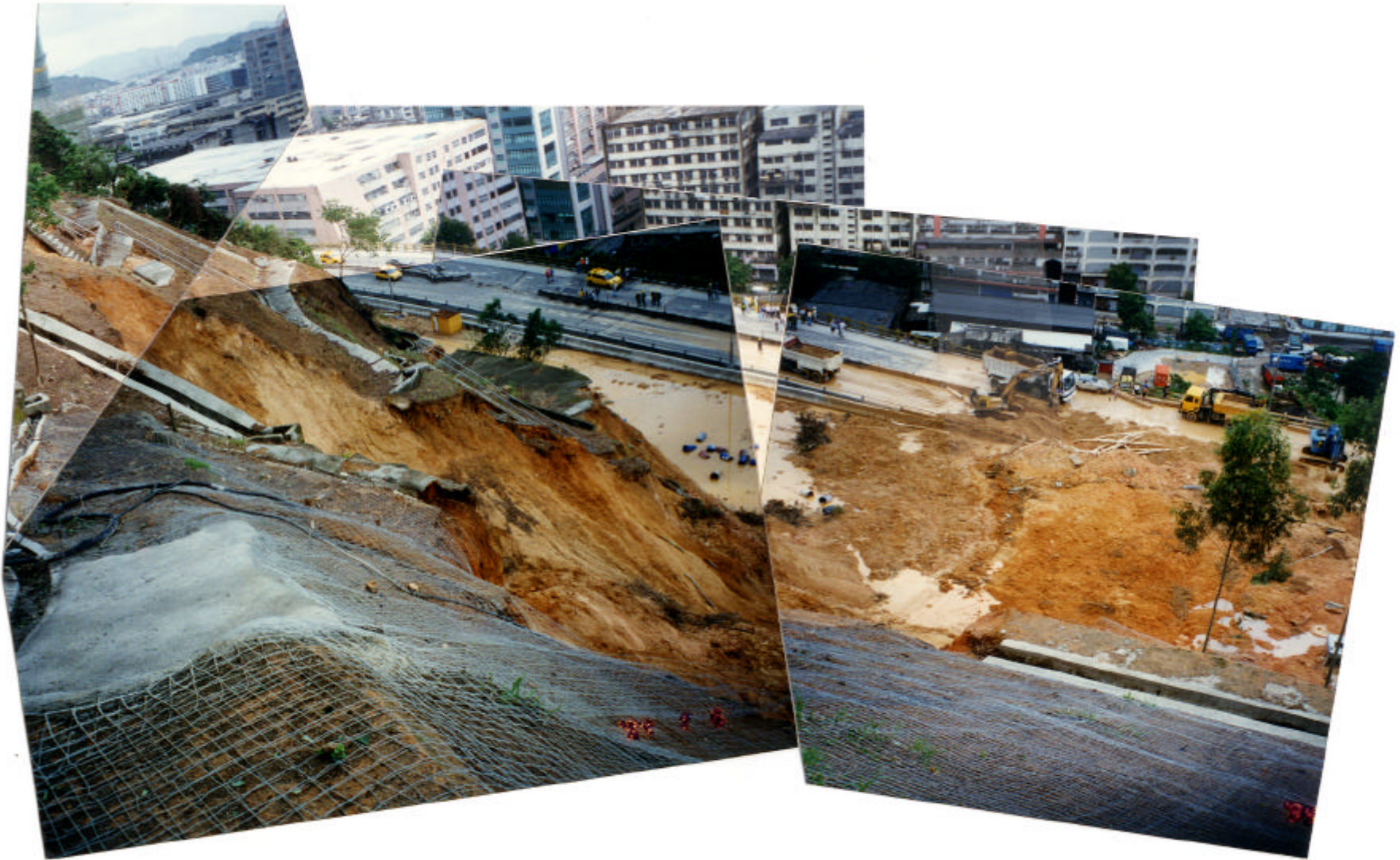
Plate 7 - View of 3 August 1997 Landslide from Cut Slope No. 11NW-A/C55 (Photograph Taken on 3 August 1997)
