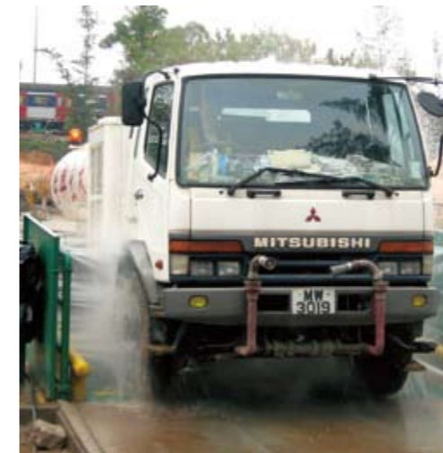
地盤出口的洗輪設施 Automated wheel-washing facility at site exits
