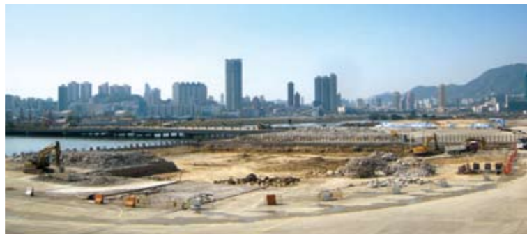
在南面停機坪挖掘污染的泥土 Excavation of contaminated soil at the south apron
