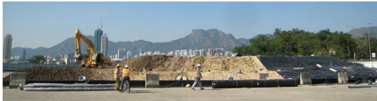
建造生物堆土及安裝通氣管道 Formation of biopile and installation of aeration pipes
