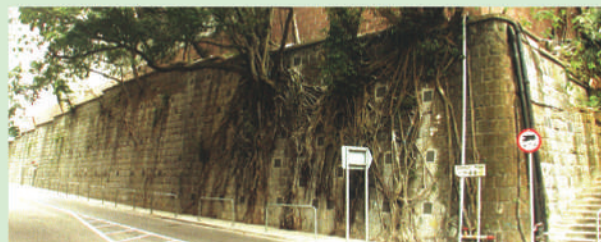
在擋土牆鞏固工程中採用泥釘可保留現存樹木 Existing trees are retained after upgrading works using soil nails
