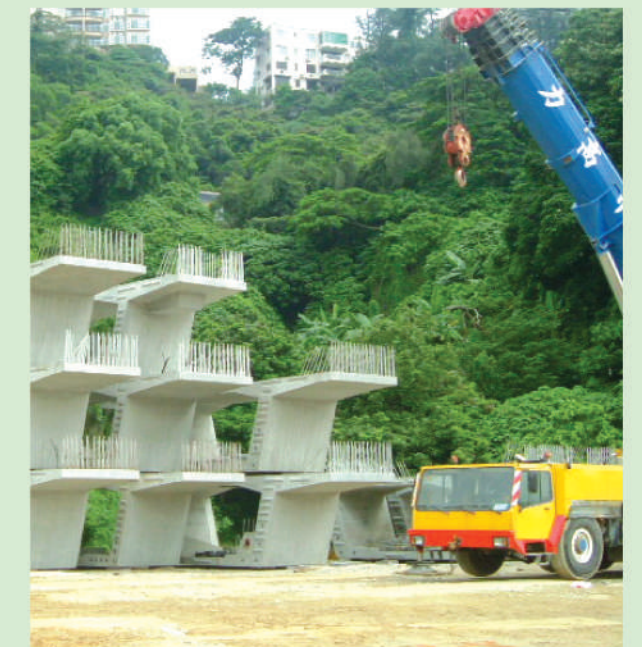
採用預製組件以減少建築廢料 Use of precast elements to reduce construction waste
