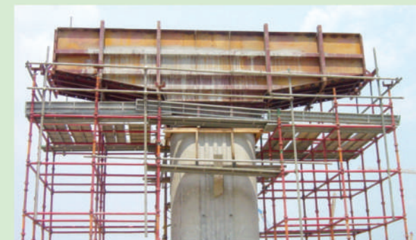
採用金屬模板以減少建築廢料 Use of metal formwork to reduce construction waste
