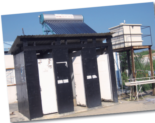
工地內設置的太陽能熱水系統 Solar powered water heating system on works site
