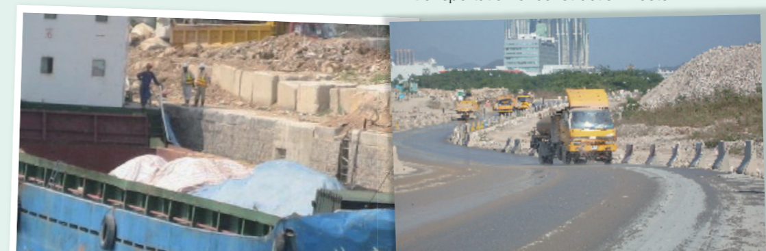
在躉船上以帆布覆蓋運送填料 Covering the material by tarpaulin on barge during delivery 經常於工地範圍灑水以控制泥塵散播 Regular water spraying on sites for dust control
