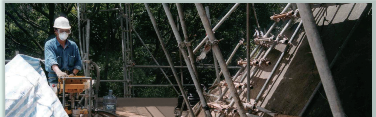
在斜坡工程中慣常使用的控制塵埃措施 (在鑽孔時使用帆布遮擋和灑水以減少塵埃散發) Typical dust-control measures employed in slope engineering works (use tarpaulin sheets and water spraying to suppress dust generated from drilling)
