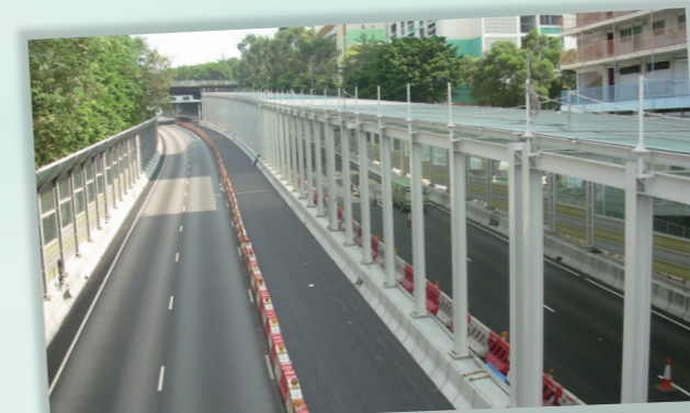
垂直式隔音屏障和半封閉式隔音罩 Noise barriers and semi-noise enclosures
