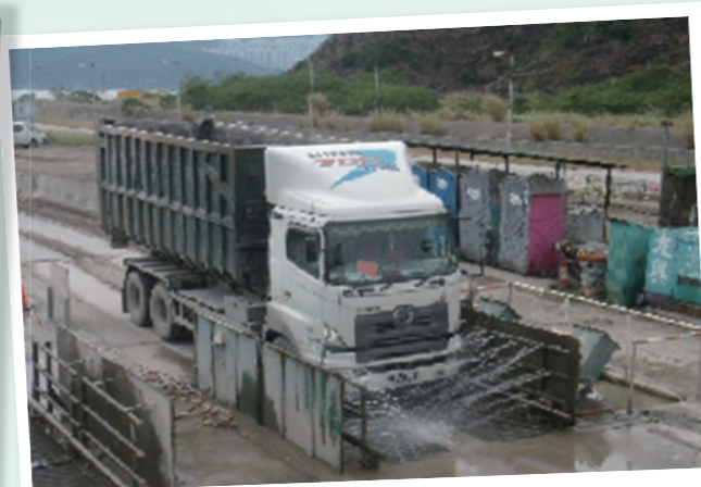
在工地出口處提供洗車設施，以便清洗車身及車輪上的塵埃 Wheel-washing facilities at site exits to wash away dusty material from vehicles
