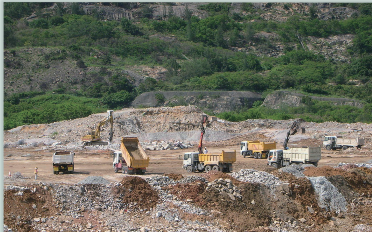
屯門公眾填料接收設施 The public fill reception facility at Tuen Mun
