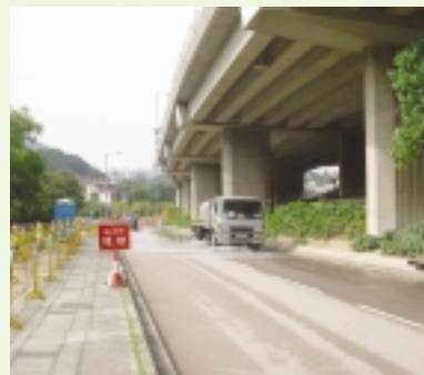
定期清洗工地旁的公用道路 Regular cleaning at public road adjacent to the work site
