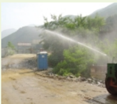
地盤運料路的灑水系統 Water spraying system at site haul road
