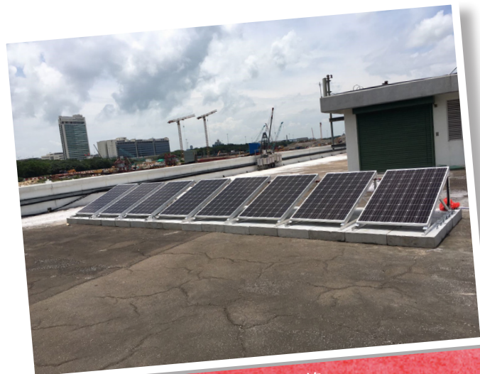
於東涌發展碼頭(公眾)的太陽能系統 Solar Energy System in Tung Chung Development Pier (Public)
