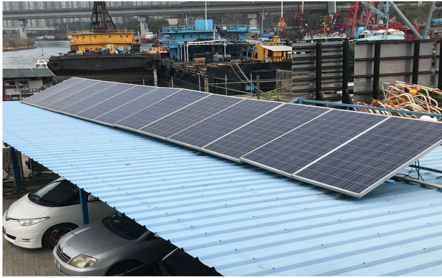
於地盤辦公室樓頂安裝太陽能電板作為照明電源 Installation of Solar Panels at Roof of the Site Accommodation for Lighting Purpose
