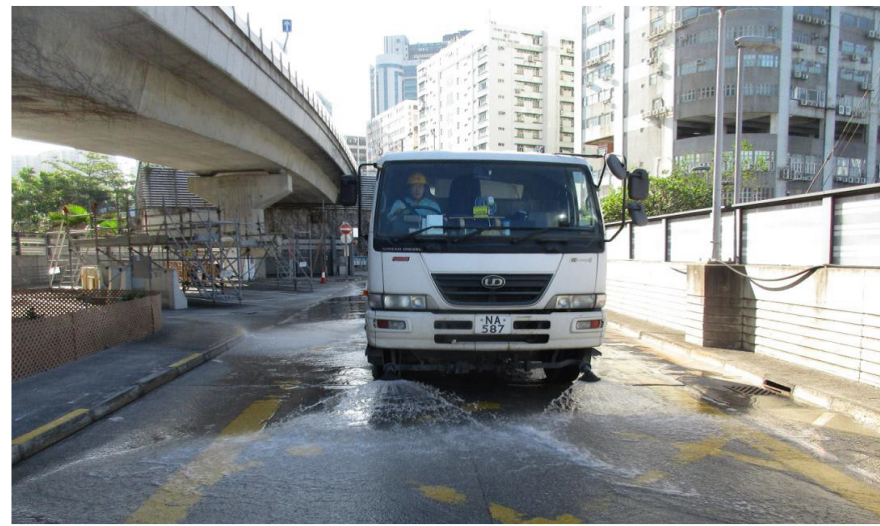
在地盤及鄰近公共道路上使用洗街車清理泥頭車遺下的泥塵 Use of Street Sweeper to Reduce Dusty Materials on Site and Neighboring Public Roads
