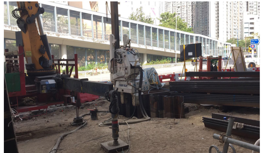
使用靜音式打樁機，降低工程期間製造的污染如噪音及振動，亦減少路面沉降 Use Silent Piler to Minimize the Construction Pollution Like Noise and Vibration, Contributing Less Ground Settlement as well
