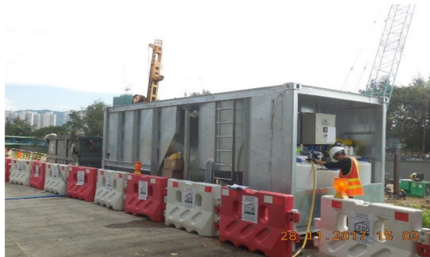
使用專用污水淨化設備加強污水處理效能 Use of Wetsep to Facilitate Sedimentation in Wastewater Treatment
