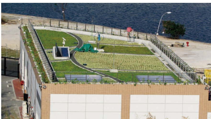
啟德發展計劃 — 前跑道南發展項目的前期基礎設施第一期工程 Kai Tak Development — Advance Infrastructure Works for Developments at the Southern Part of the Former Runways, Stage 1 污水泵房的屋頂綠化 Green roof of sewage pumping station
