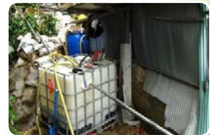
九龍及新界東(南)防治山泥傾瀉工程 Landslip Prevention and Mitigation Works in Mainland East (South) 回收及過濾泥釘工程的廢水循環再用 Flushing water used for coring of soil nails was collected, desilted and then reused
