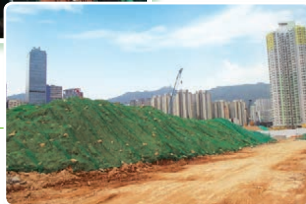
啟德發展計劃 Kai Tak Development 妥善覆蓋堆放的泥土以減少塵埃 Stockpile of soil properly covered up for dust control
