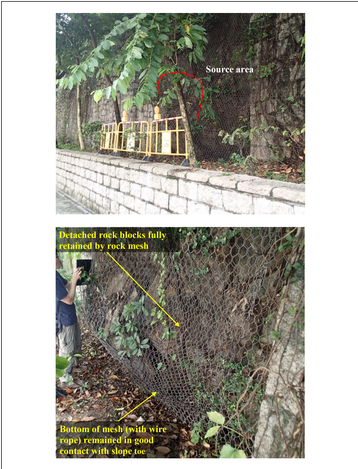
Figure 4.2 Incident at Castle Peak Road, Sham Tseng with Rockfall Debris Fully Retained by Rock Mesh (Incident No. 2019/08/2482)
