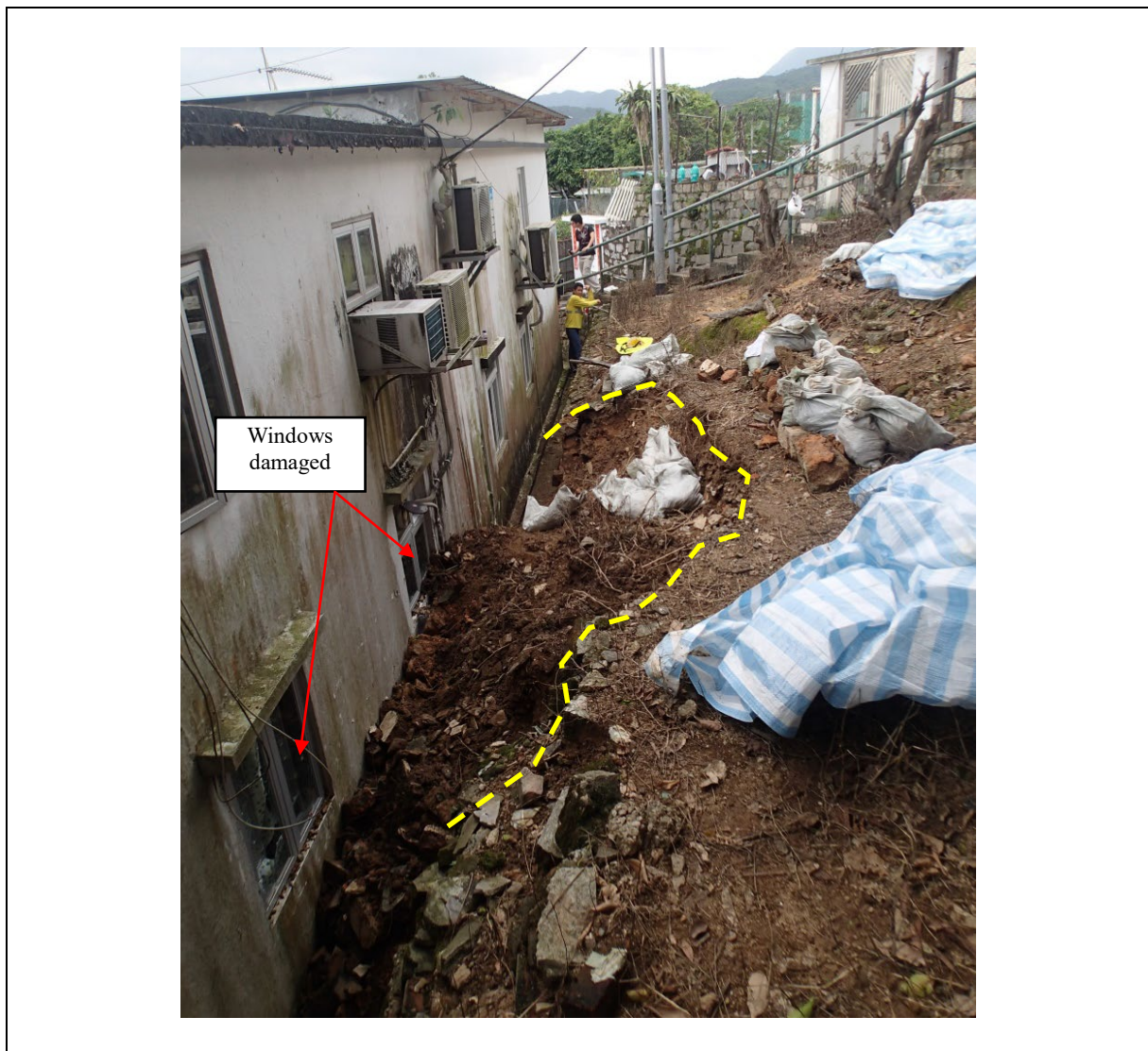
Figure 4.3 View of the 19 April 2019 Landslide on a Retaining Wall behind Nos. 24 and 25 O Long Village, Sai Kung (Incident No. 2019/04/2427)
