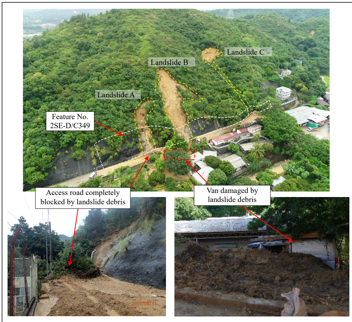
Figure 4.4 Views of the 29 August 2018 Landslides on the Natural Hillside at Ta Shek Wu Kiu Tau, Sheung Shui (Incident No. 2018/08/2231)
