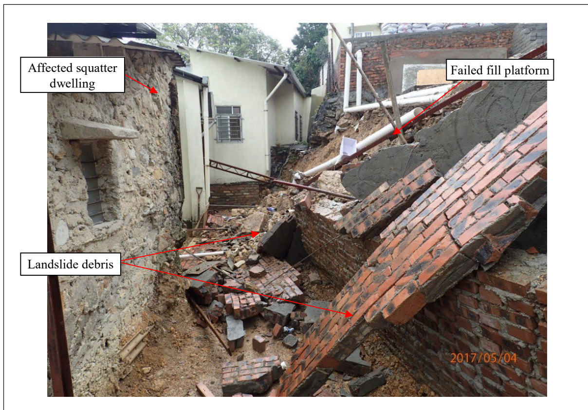
Figure 4.1 View of the 4 May 2017 Landslide at an Unregistered Fill Platform behind a Squatter Structure at Shung Him Tong Village, Fanling (Incident No. 2017/05/2009)
