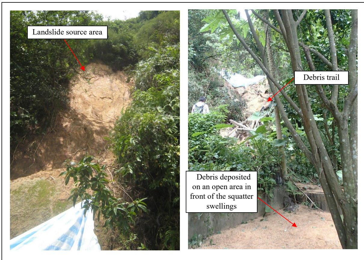
Figure 4.2 View of the 21 June 2017 Landslide on Slope No. 11SE-B/C635 behind Sam Ka Tsuen, Lei Yu Mun (Incident No. 2017/06/2052)
