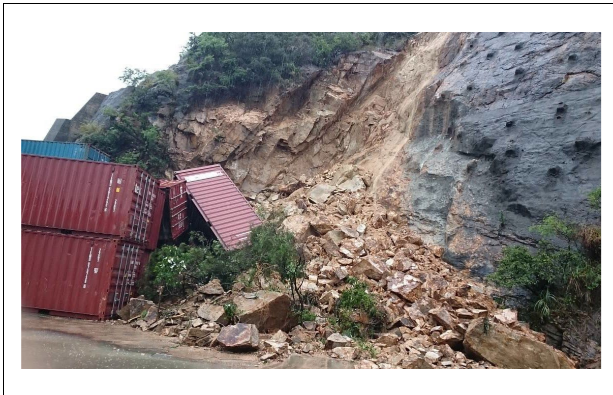
Figure 4.4 View of the 24 May 2017 Landslide on Slope No. 10NE-B/C57 below Tsing Yi Road, Tsing Yi (Incident No. 2017/05/2017)
