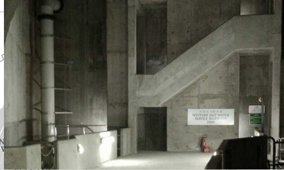
Western Salt Water Service Reservoirs at HKU (2009)
