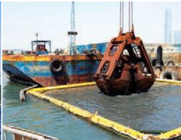
Silt curtain around the dredging area to confine the dispersion of marine deposits
