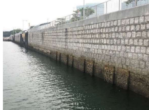
Eco-engineering such as blockwork seawall with eco panels / oyster basket to improve marine ecology and mitigate sediment transport. Existing defences can be integrated with eco-engineering to create hybrid infrastructure.
