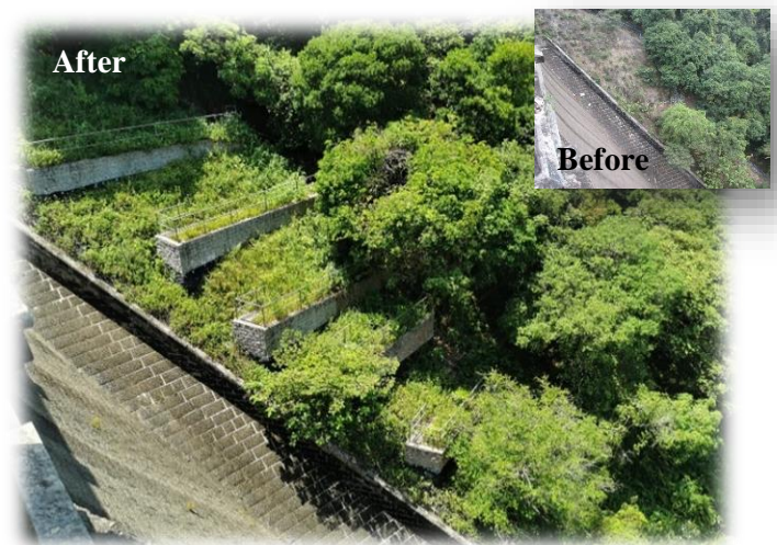
Champion of the Man-made Slope/Retaining Wall Category. Picture shows the changes of the slope next to the dam of Kowloon Byewash Reservoir before and after the works.
