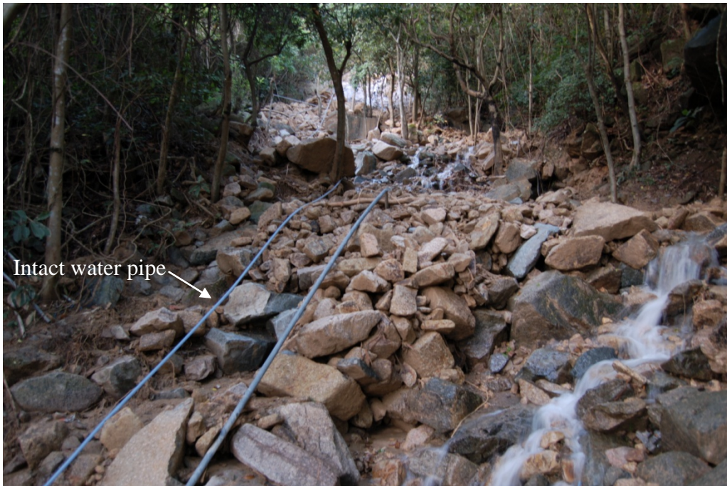
Plate 38 - Upstream View of Primary Drainage Line at about CH320 (Photograph taken on 11 June 2008)
