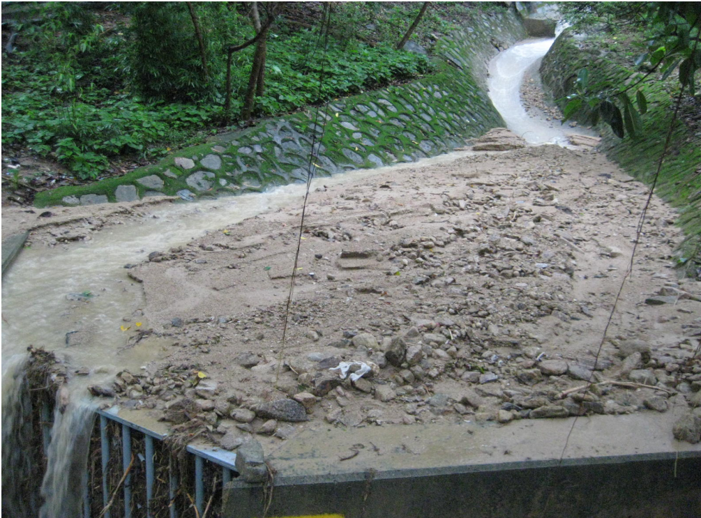
Plate 4 - Record Photograph from DSD Showing Blockage at the Rock Trap above Slope No. 11NE-A/C300 at Tsz Ching Estate (Photograph taken on 13 June 2008)
