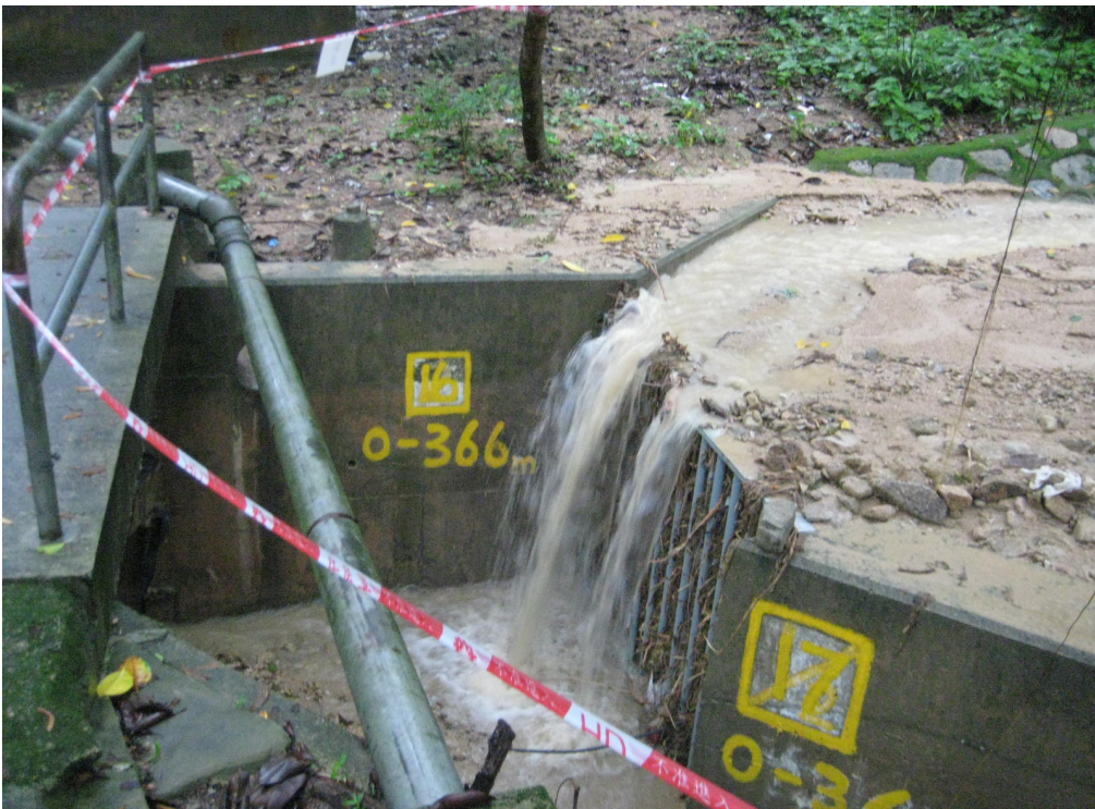
Plate 5 - Record Photograph from DSD Showing Overflow of the Rock Trap above Slope No. 11NE-A/C300 at Tsz Ching Estate (Photograph taken on 13 June 2008)
