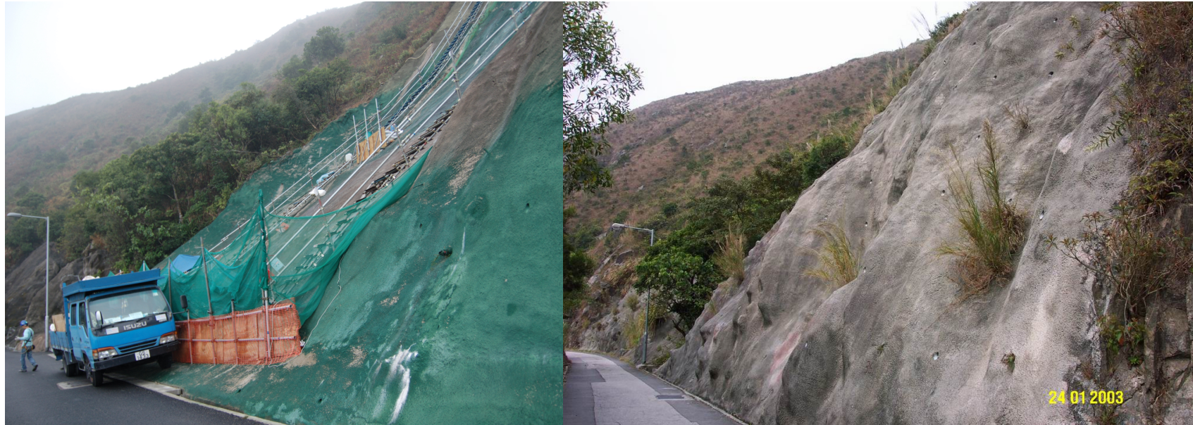
Plate 41 - Post-landslide Slope Profile in January 2010 when the Ground Investigation Works were Undertaking, and Contrasting with the Pre-failure Slope Profile in 2003
