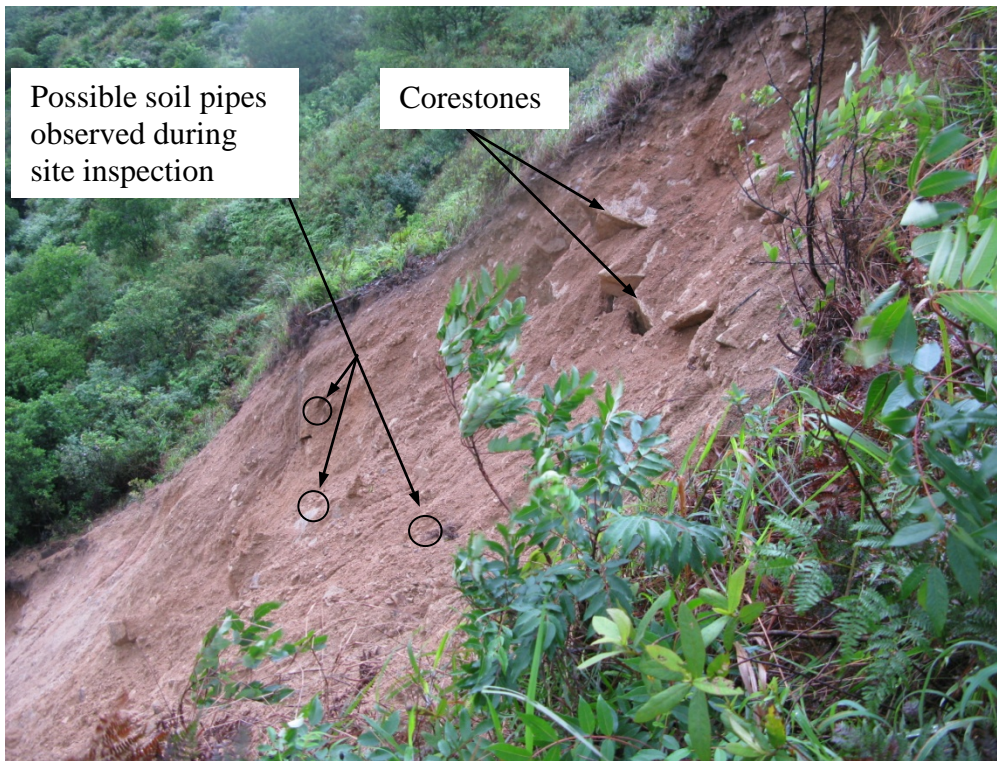
Plate 26 - Possible Soil Pipes and Presence of Corestones Exposed on Surface of Rupture (Photograph taken on 26 June 2008)
