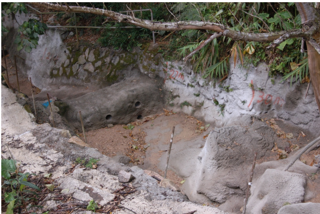
Plate 15 - View of Sedimentation Steps Constructed after 7 June 2008 Landslide Incident (Photograph taken on 6 January 2010)
