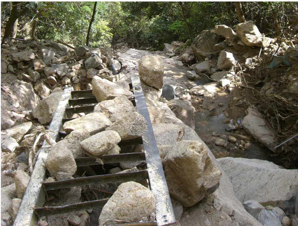
Plate 39 - View of Collapsed Section of Steel Maintenance Staircase of Slope No. 11NE-A/C351 at Primary Drainage Line at about CH250 (Photograph taken on 23 July 2008)
