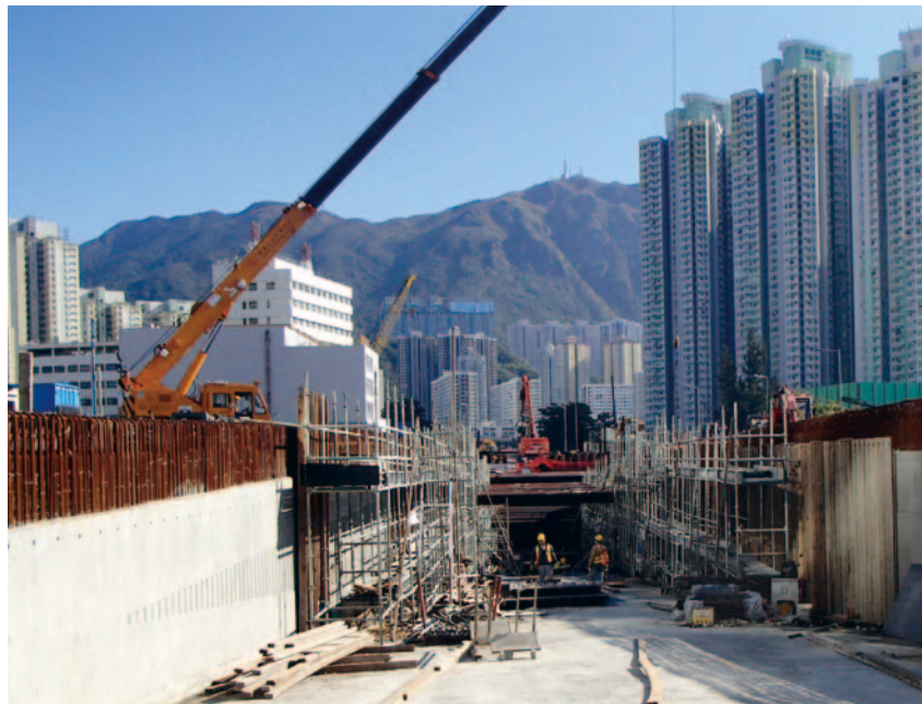
協調道行车隧道的澆灌混凝土工程 Concreting works of approaching ramp of vehicular underpass at Concorde Road
