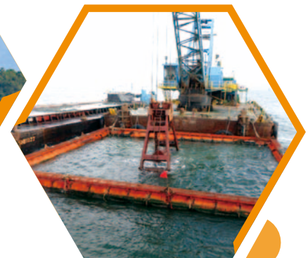
葵青貨櫃港池及其進港 航道的疏浚工程 Dredging works in Kwai Tsing Container Basin and its Approach Channel
