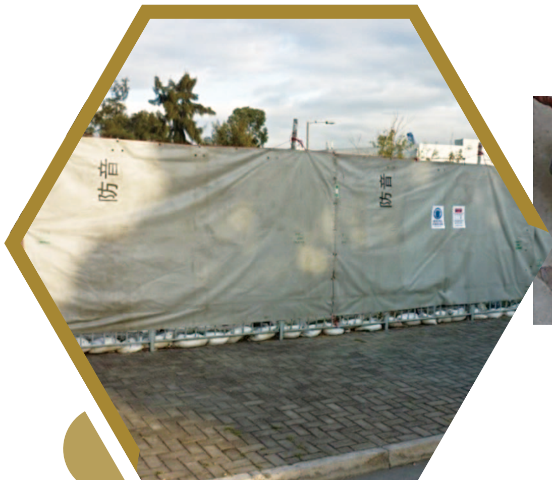
採用臨時隔音屏障以減低噪音 Provision of temporary noise barrier to reduce noise emission
