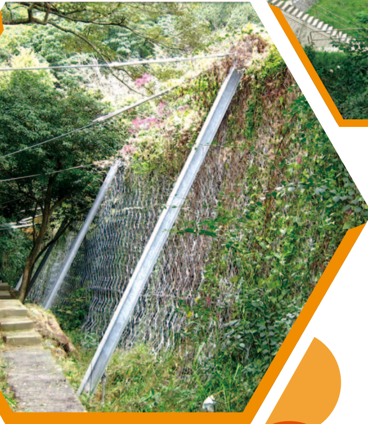
在灣仔堅尼地道天然山坡建造柔性防禦網以減低天然山坡塌滑風險 Construction of flexible barrier to mitigate open hillside failure in the natural hillside above Kennedy Road, Wan Chai
