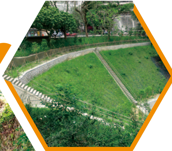
位於砲台山道及天后廟道交界處的防治山泥傾瀉工程 Landslip Prevention and Mitigation Works at the junction of Fortress Hill Road and Tin Hau Temple Road
