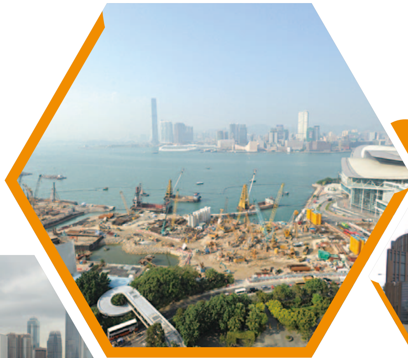
香港會議展覽中心西面正全速進行土地平整工程 Land formation works at the west of Hong Kong Convention and Exhibition Centre in full swing
