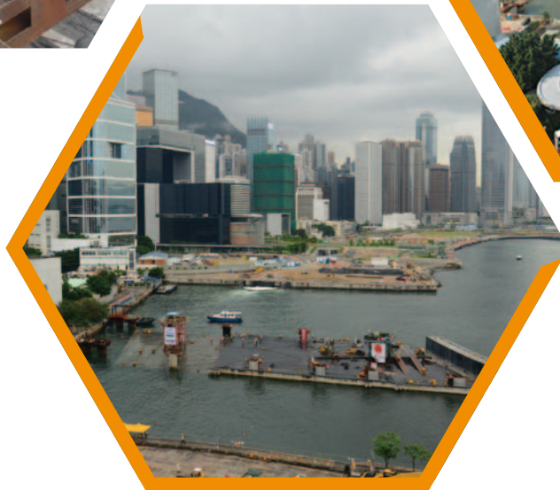
港鐵荃灣線過海隧道上方安裝巨型預製結構 Installation of gigantic precast structure above the MTR Tsuen Wan Line tunnel
