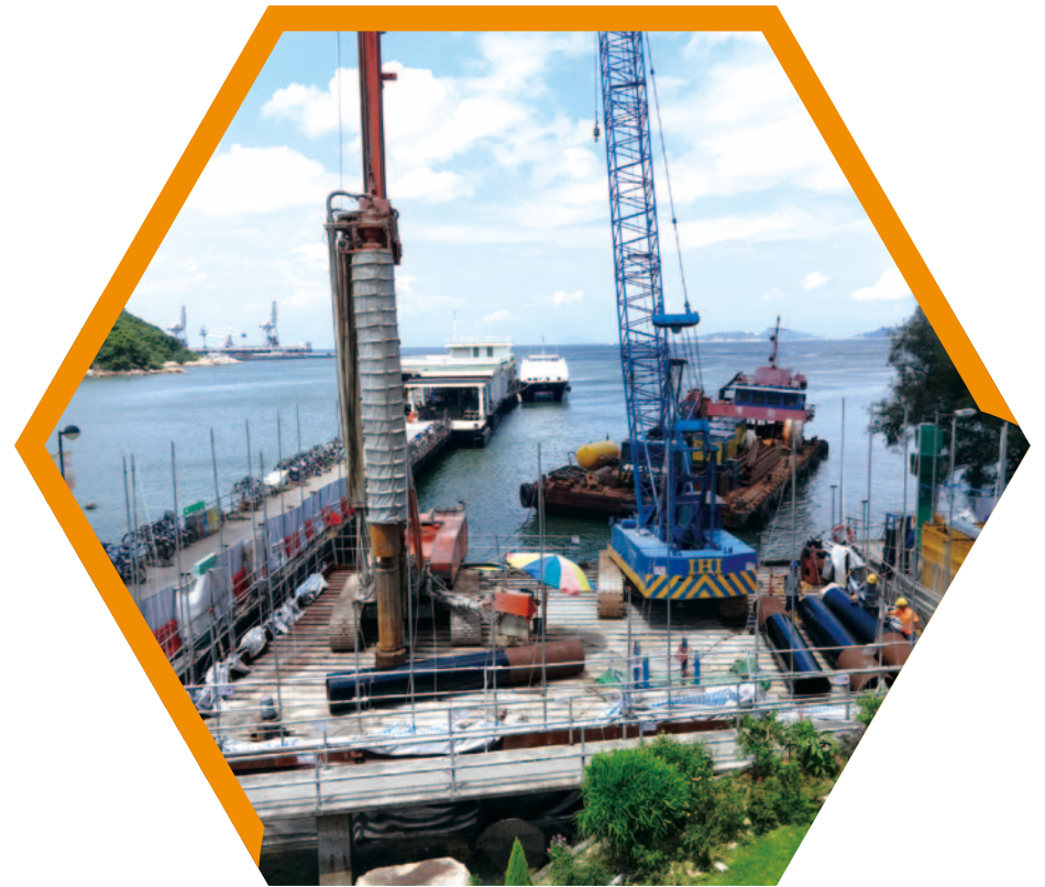
南丫島榕樹灣渡輪碼頭附近 興建單車停泊處 Construction of a cycle parking area near Yung Shue Wan Ferry Pier, Lamma Island
