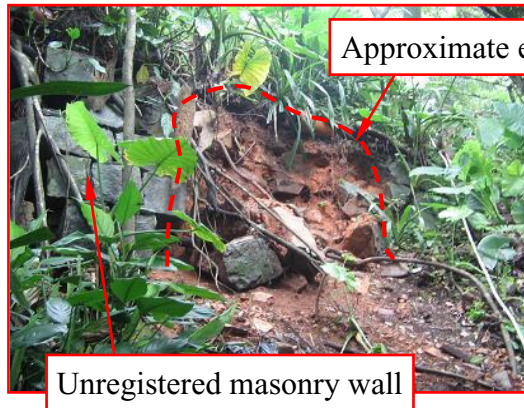
Close-up view of the failure scar
