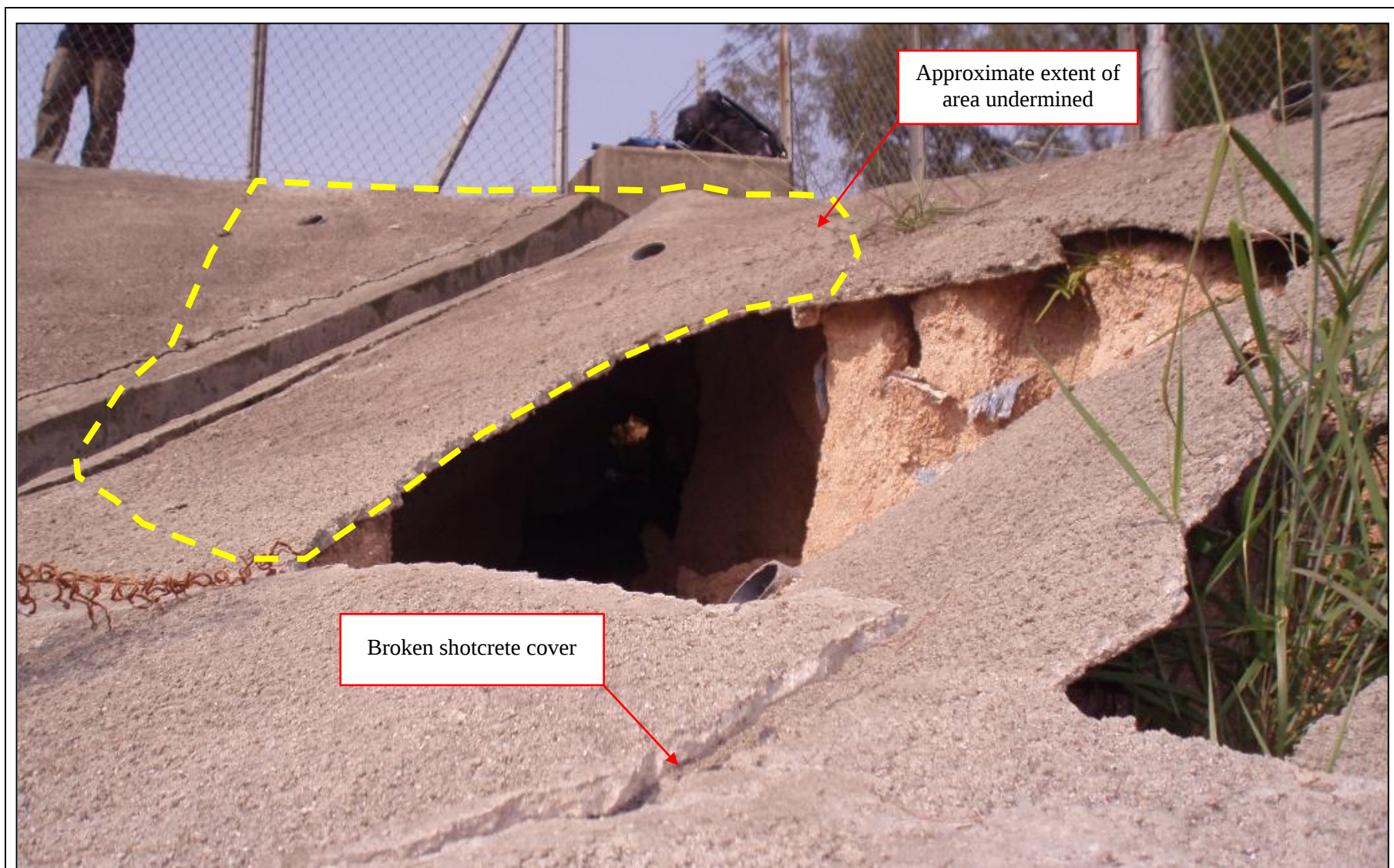
Plate 3 - The 14 November 2007 Landslide Incident at Pui Man Street
