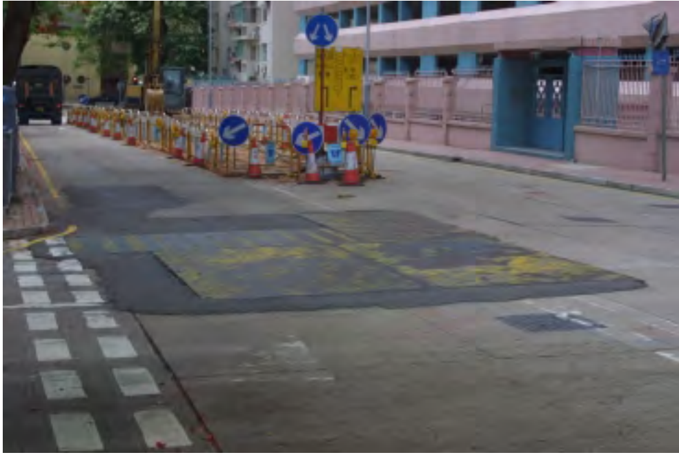
Plate B1 – Typical vehicle crossing over trench opening which is also effective for preventing surface runoff and infiltration of rainwater
