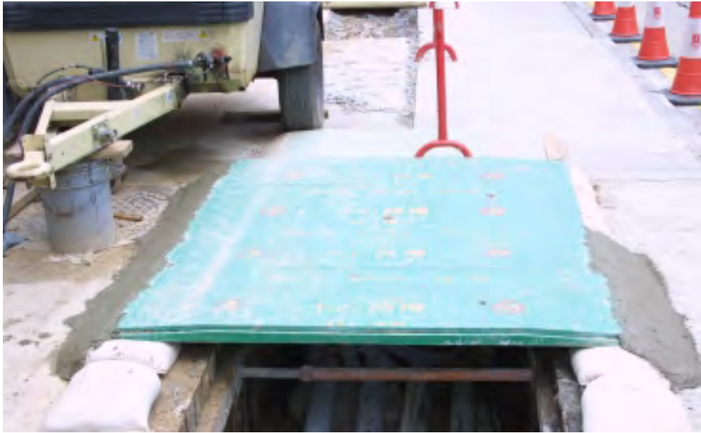
Plate B3 – Sandbag upstand with fibre-glass cover to prevent surface runoff and infiltration of rainwater
