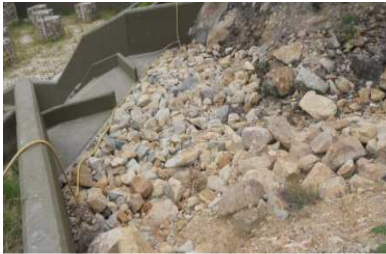
Plate 1 - Loose Surface Materials at Debris Approaching Zone
