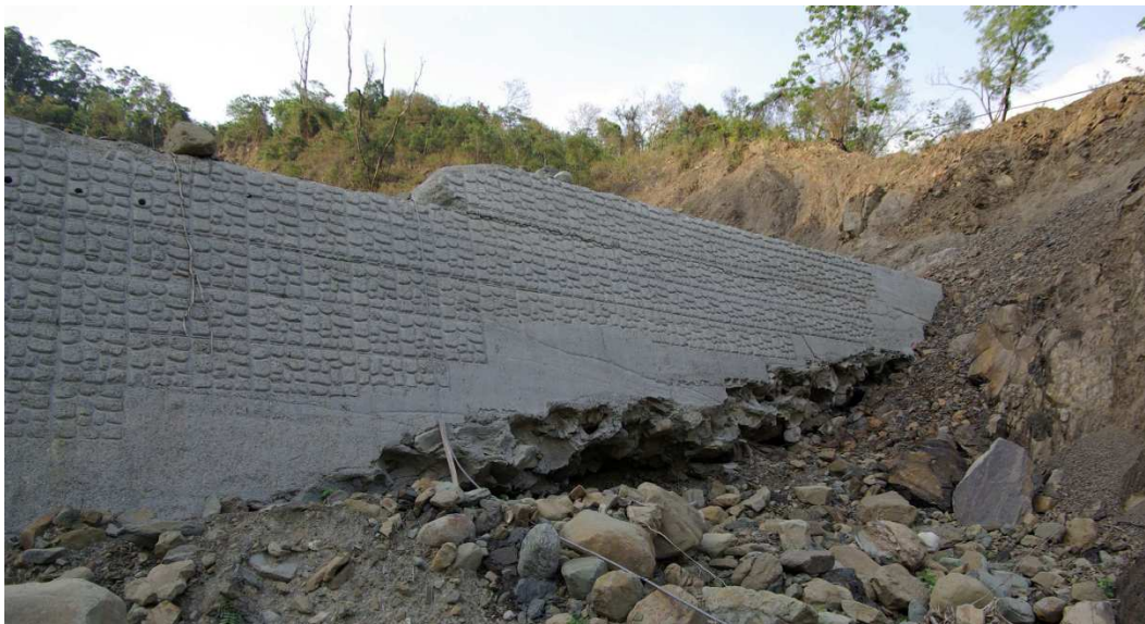
Plate 2 - Foundation of a Barrier Undermined after a Debris Flow Event
