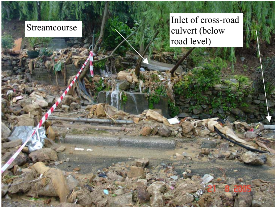
Plate 28 - Area in the Vicinity of Inlet of the Cross-road Culvert (Photograph taken by HyD on 21 August 2005)
