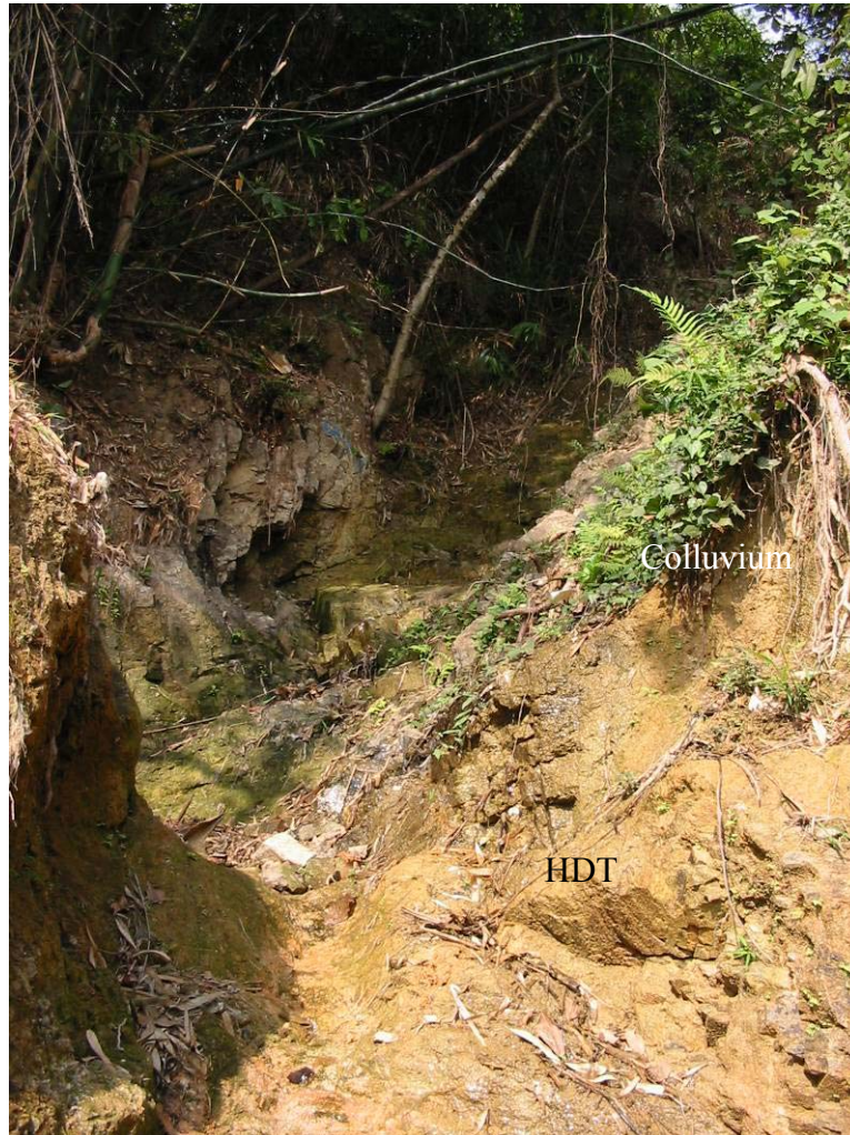
Plate 19 - View of Middle Portion of the Debris Flood Trail at CH 88 (Photograph taken on 22 February 2006)
