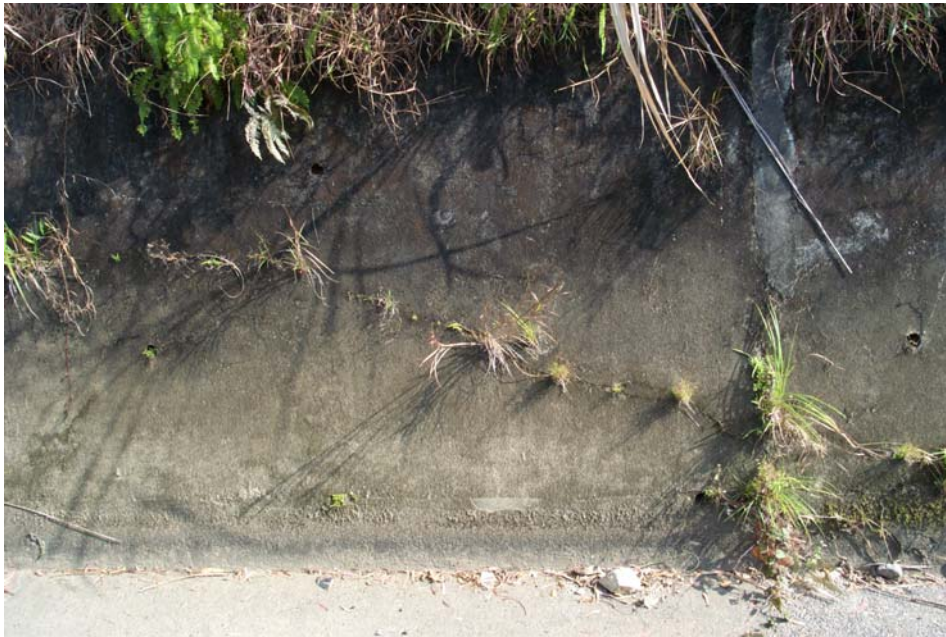
Plate 9 - Cracking of Catchwater Channel before the Landslide on Slope No. 6SE-B/CR249 (Photograph taken on 7 December 2000)
