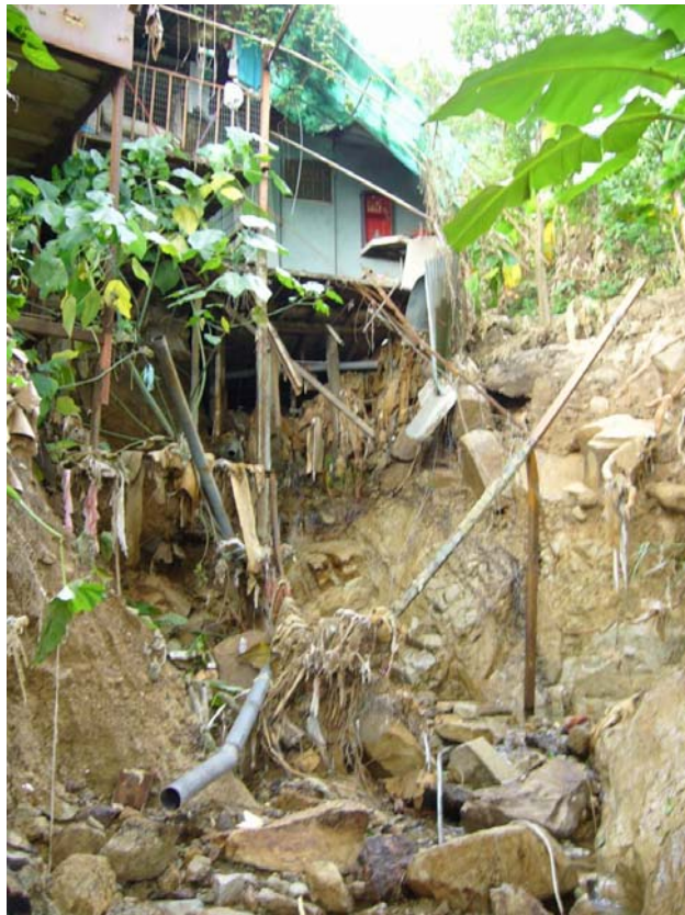
Plate 4 - View of Undermining of Registered Squatter Structure No. RTW/4D/296 along Streamcourse (Photograph taken on 26 August 2005)
