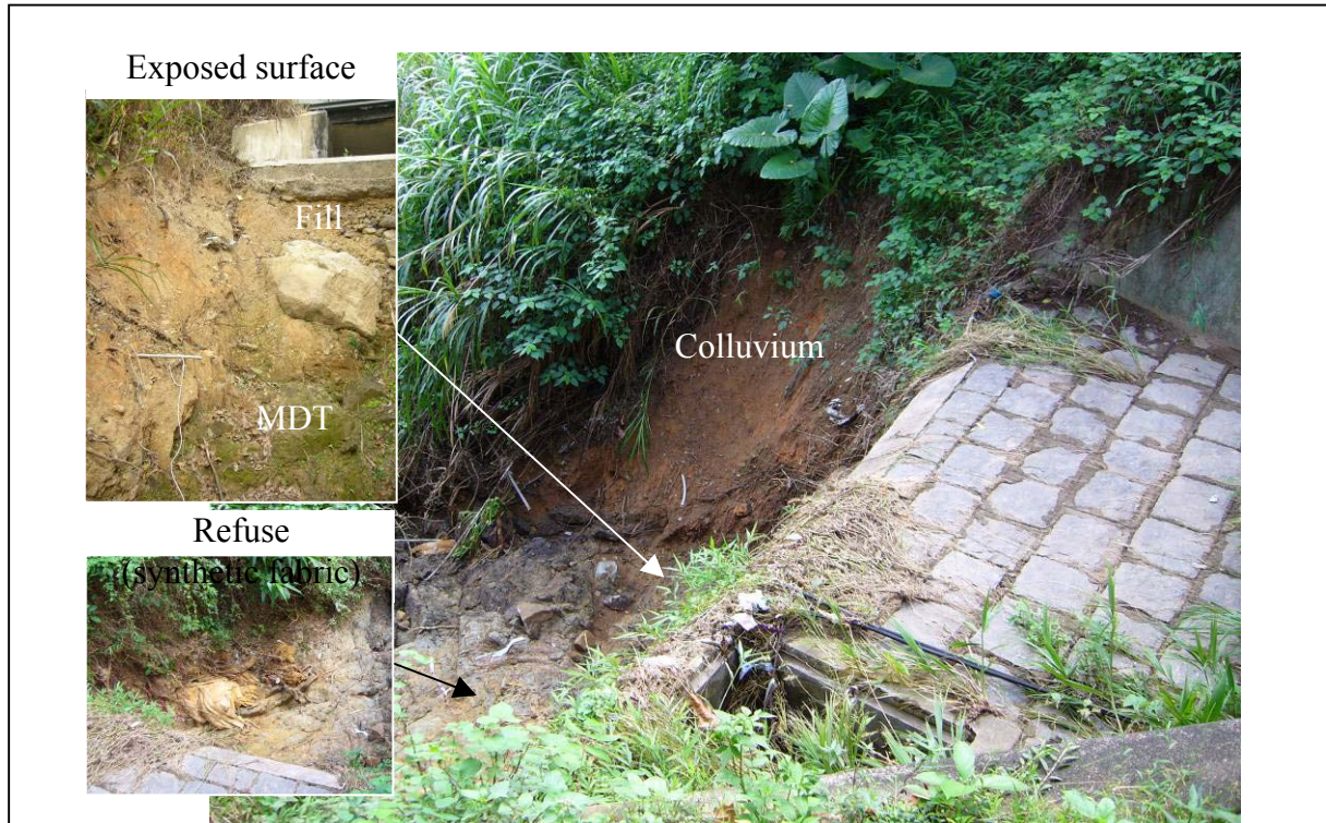
Plate 13 - Erosion below Overflow Weir SMOF-28 (Photograph taken on 26 August 2005)
