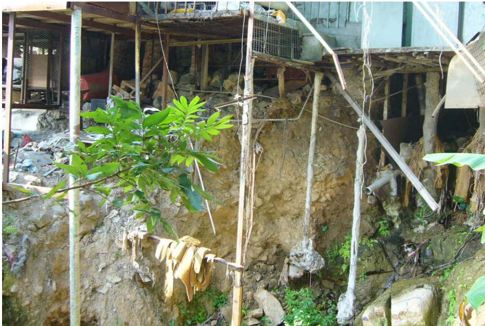
Plate 26 - Erosion underneath Registered Squatter Structure No. RTW/4D/296 (Photograph taken on 22 February 2006)
