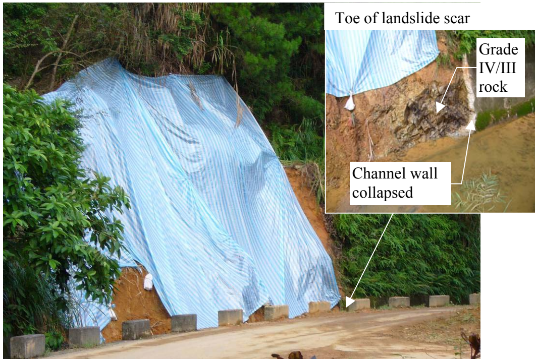
Plate 10 - General View of the Landslide on Slope No. 6SE-B/CR249 (Photograph taken on 26 August 2005)
