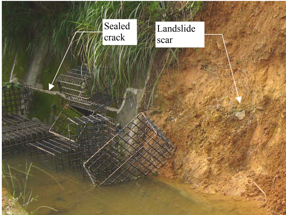
Plate 11 - Sealed Cracks on Catchwater Channel adjacent to Landslide Scar of Slope No. 6SE-B/CR249 (Photograph taken on 26 August 2005)
