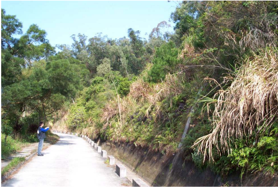
Plate 5 - General View of Slope No. 6SE-B/CR249 before the Landslide (Photograph taken on 7 December 2000)
