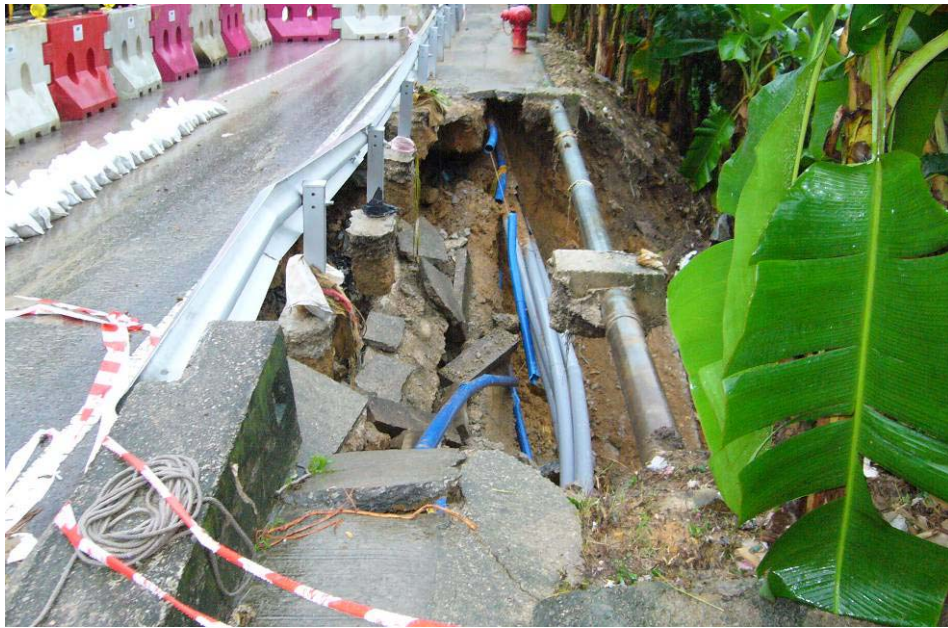
Plate 3 - View of Landslide at Slope No. 6SE-D/FR98 (Photograph taken on 21 August 2005)
