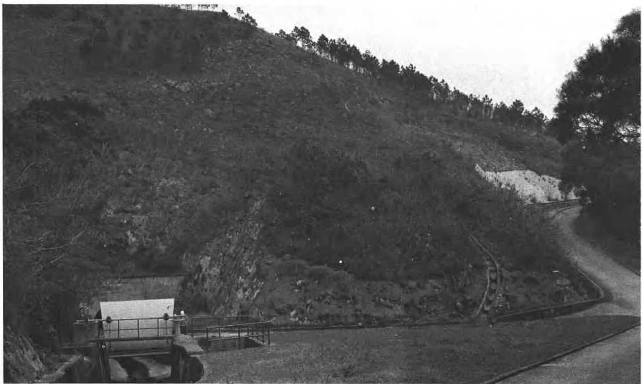
Plate 31. Chunam Surface Protection on a Cut Slope in Colluvium at the Catchwater Tunnel Portal to the Southwest of Shek Pik Dam. Numerous boulders project through the chunam which is protecting the cut slopes from erosion and infiltration.
