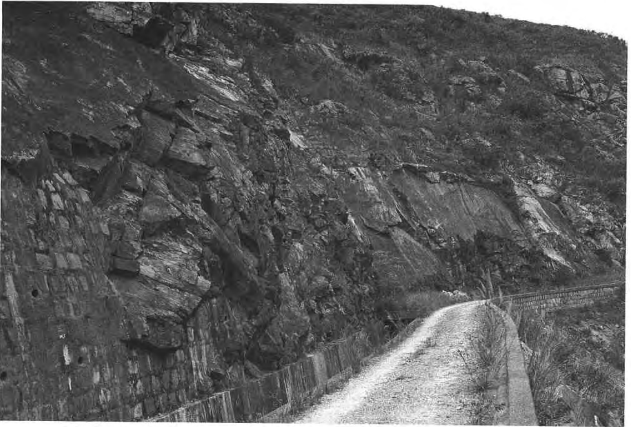
Plate 28. Adversely Jointed Volcanic Rocks in Cut Slopes Near the Western End of the Catchwater in the Keung Shan Valley. Steeply-dipping discontinuities in the bedrock have allowed blocks of rock to break away from the slope. (GCO/TP 1985/75-25).
