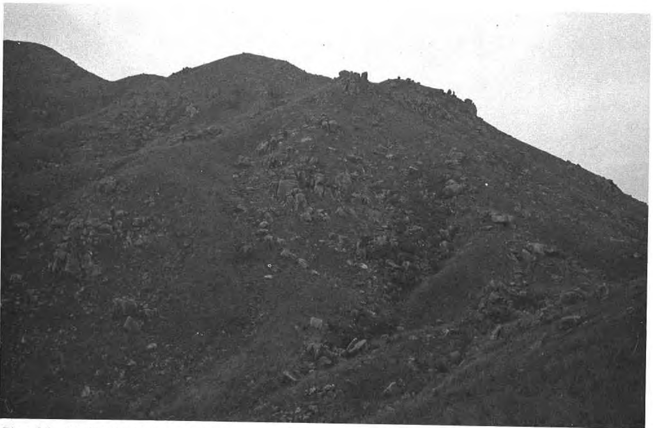
Plate 24. Mount Stenhouse on Lamma Island. Ridgecrests and sideslopes are littered with large blocks of Cheung Chau Granite which have spalled away from the insitu rock mass due to adverse jointing. (GCO/TP 1985/62-31).
