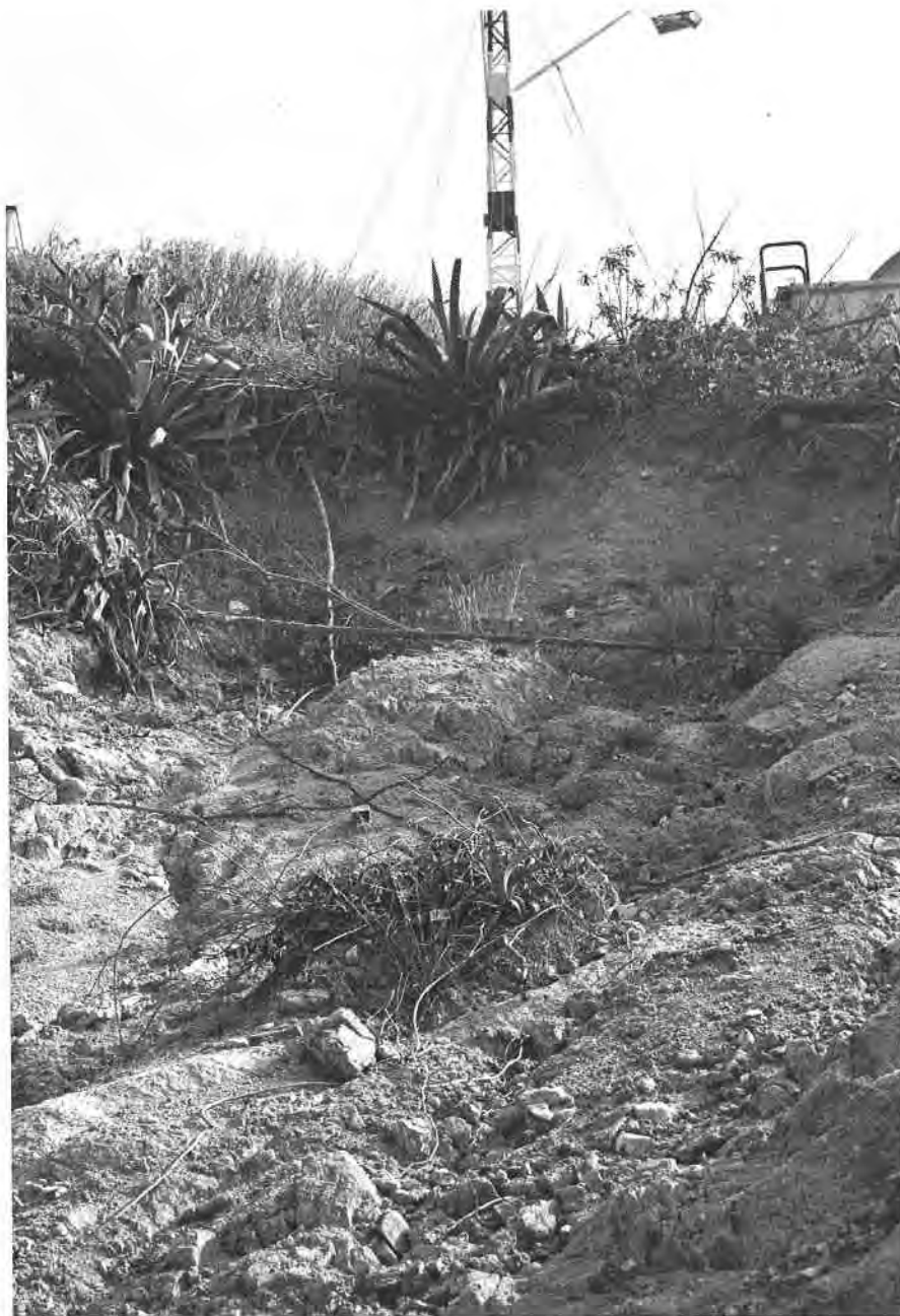
Plate 16. Landslip on the West Coast of Waglan Island.
