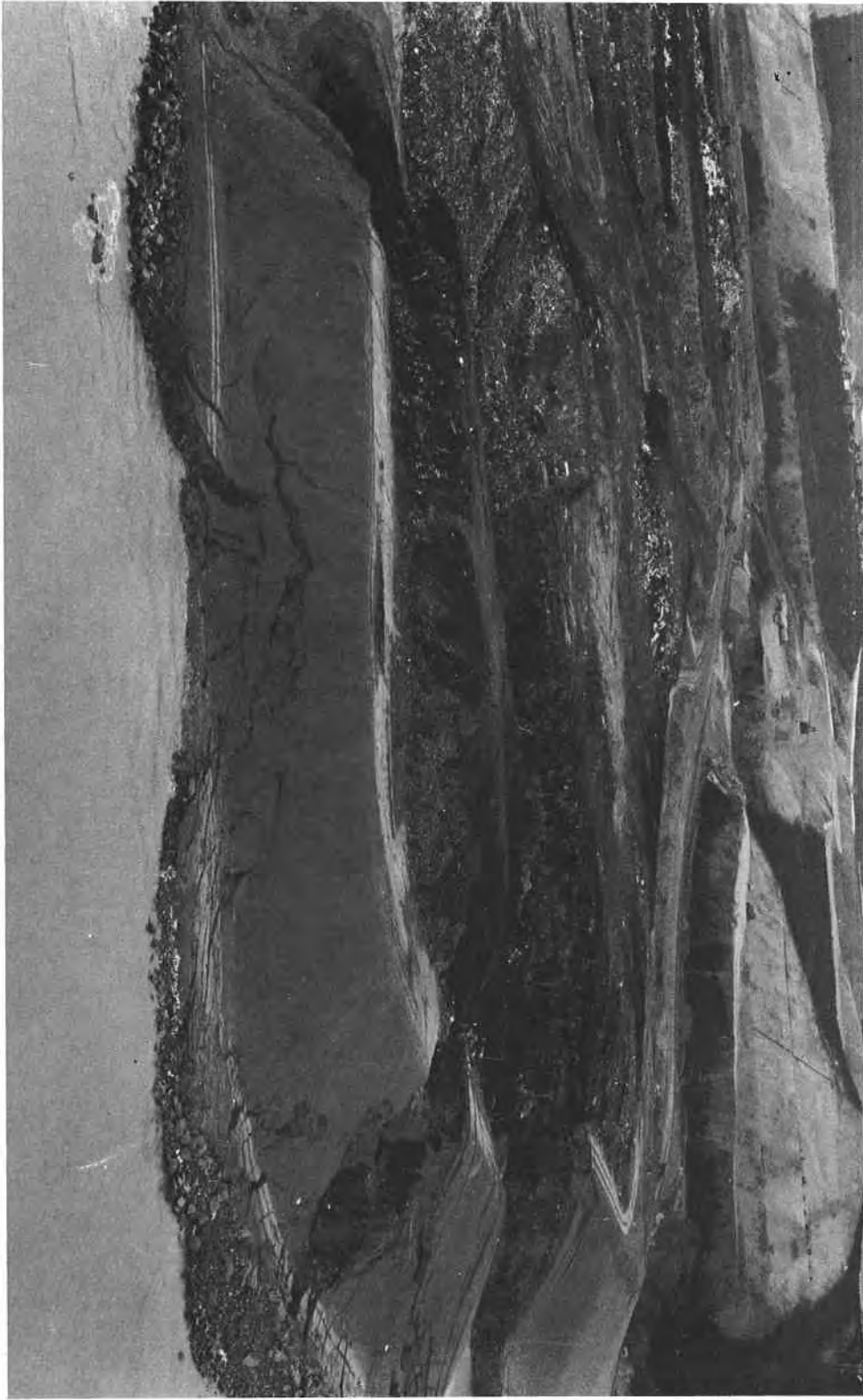
Plate 15. Failure of Landfill at the Junk Bay Controlled Tip. This Plate shows a failure of the southwestern corner of the Controlled Tip. Plant working on the site provide an indication of the scale of the failure.
