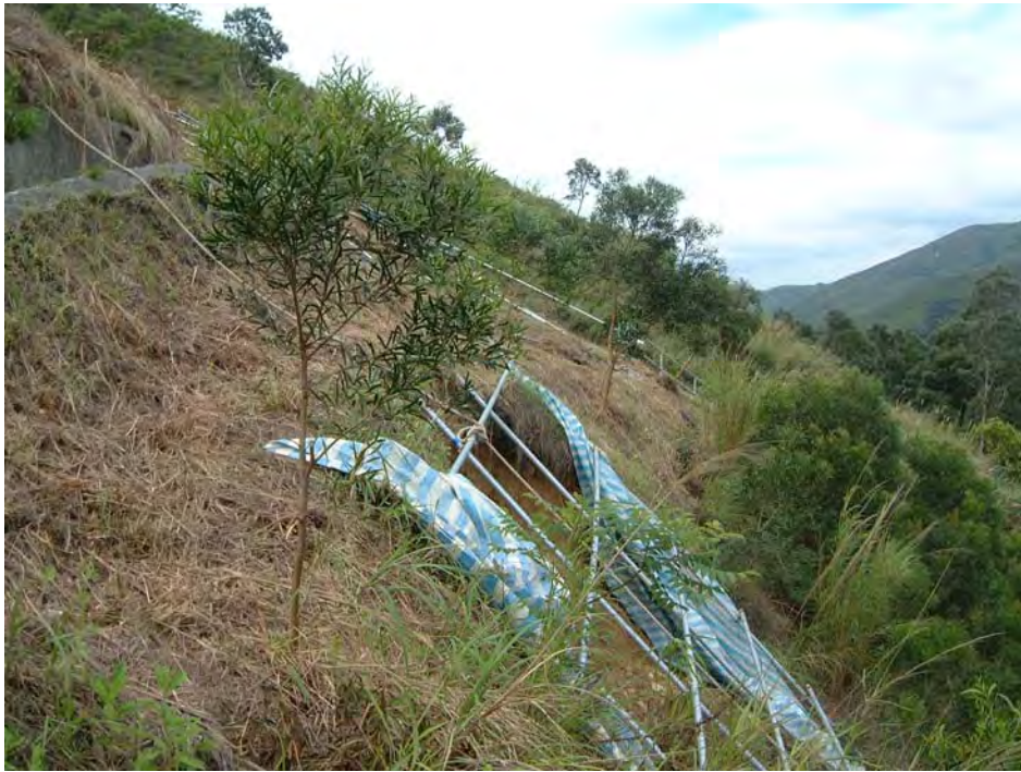
Plate 4 - Side View of the Area Immediately above the 5 May 2003 Landslide Site (Photograph taken on 16 May 2003)
