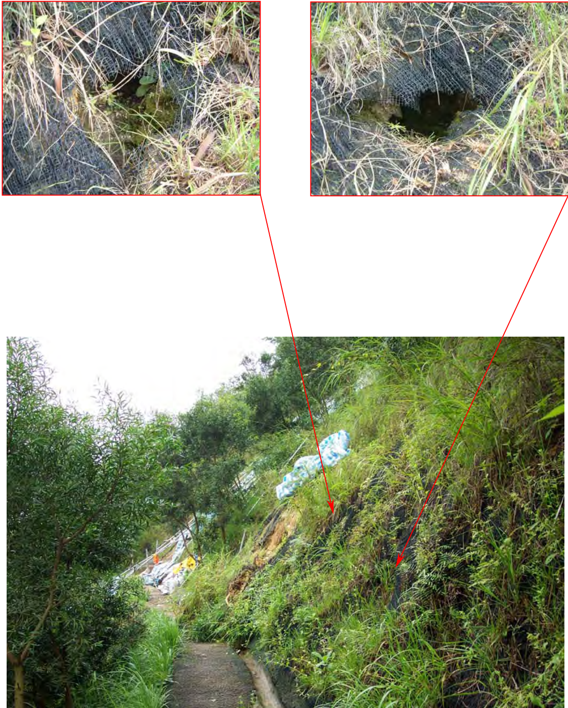
Plate 15 - View of the Erosion Scars on Slope No. 6NE-B/C8 above the Berm (Photograph taken on 14 June 2003)
