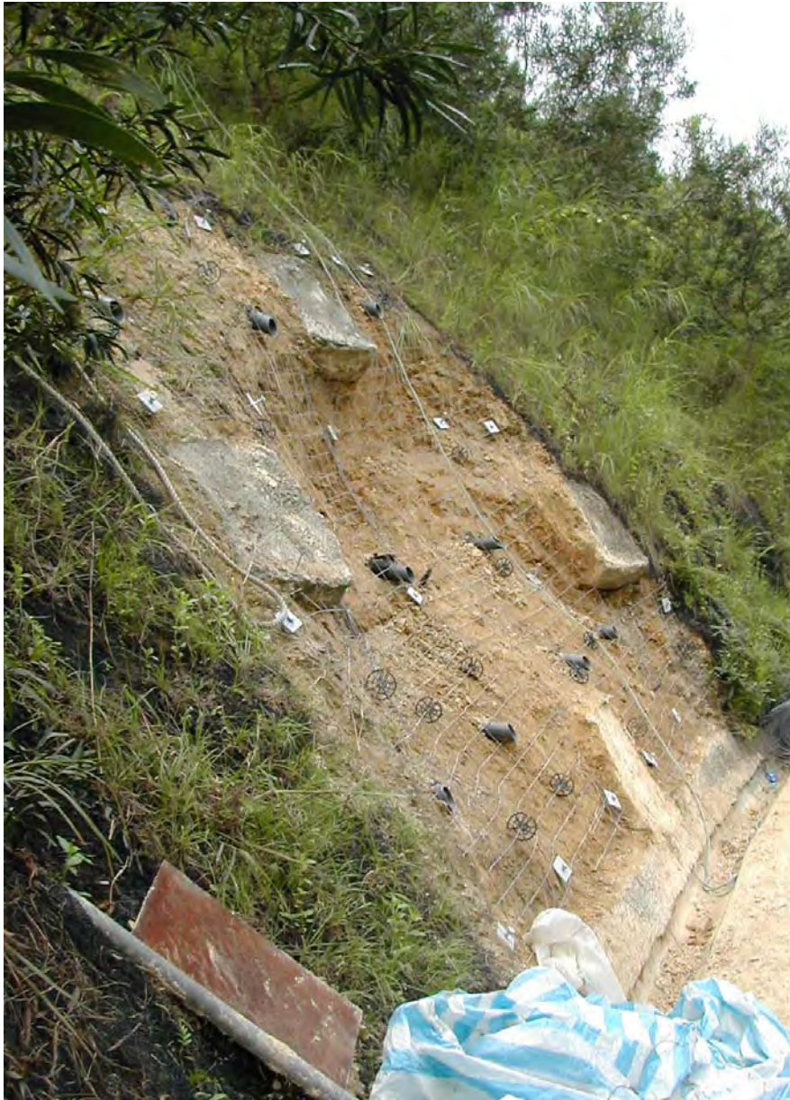
Plate 14 - View of the 13 June 2003 Landslide Following Surface Preparation for Urgent Repair Works (Photograph taken on 19 June 2003)
