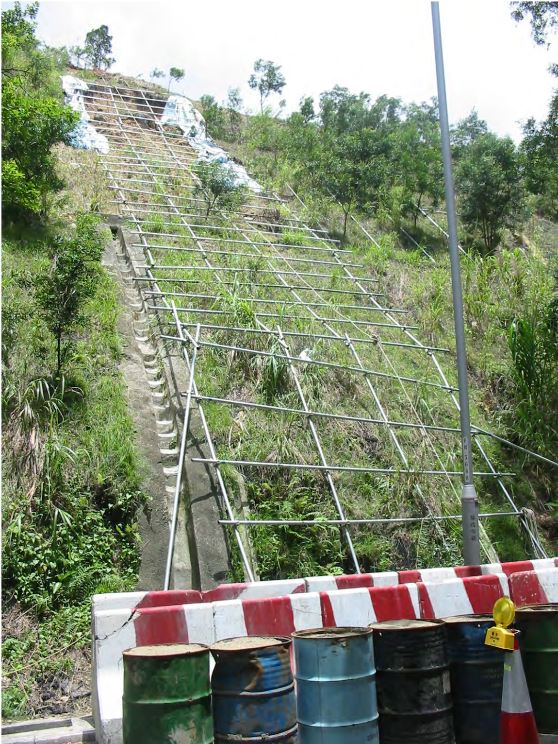
Plate 1 - General View of the 5 May 2003 Landslide on Slope No. 6NE-B/C8 (Photograph taken on 16 May 2003)
