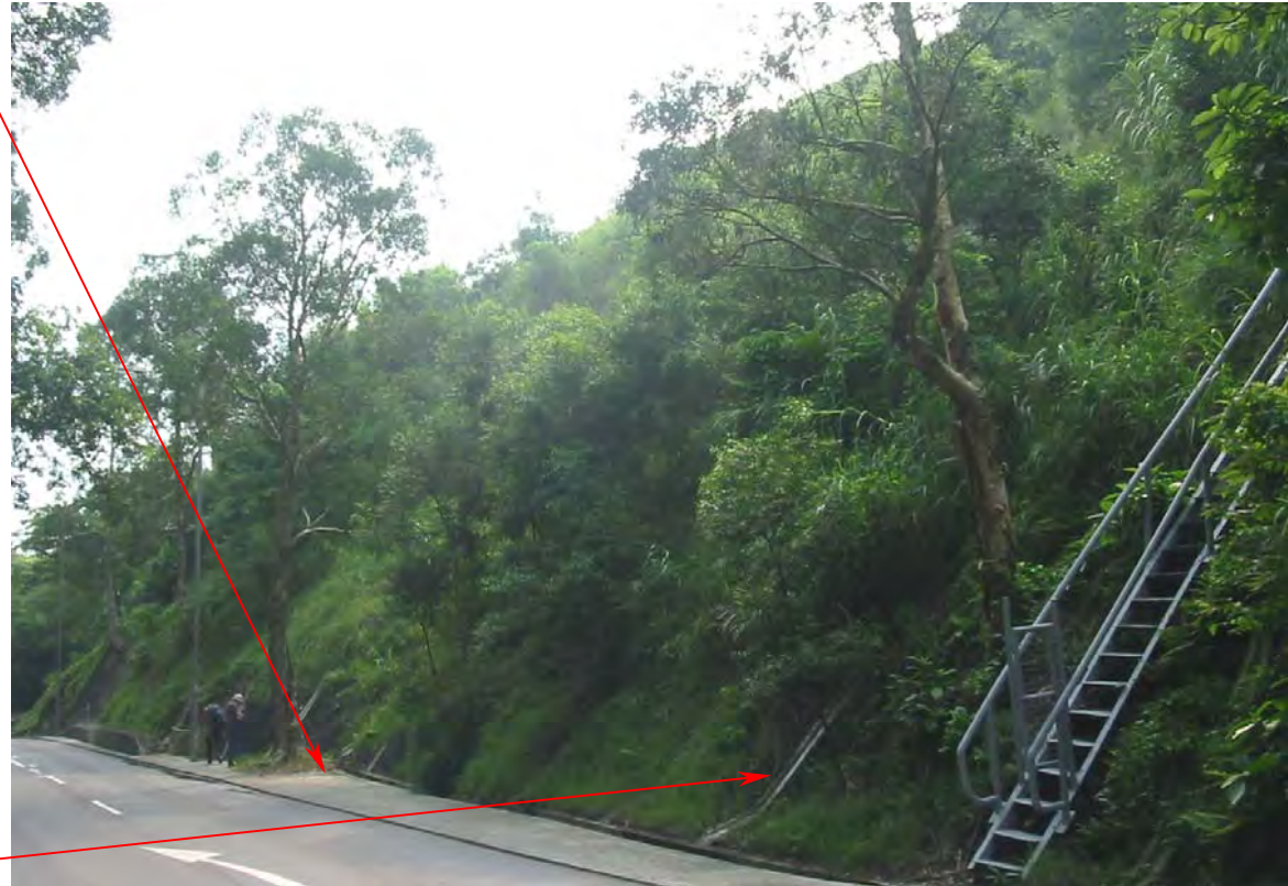
Plate 13 - View of Water Flowing from a Raking Drain and Seeping from the Interface between the Toe Surface Channel and the Pedestrian Pavement (Photograph taken on 6 August 2003)
