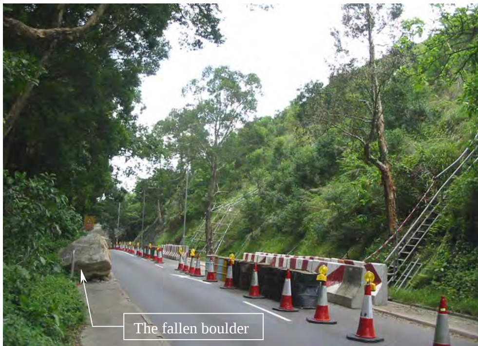
Plate 3 - General View of Slope No. 6NE-B/C8 and the Fallen Boulder (Photograph taken on 16 May 2003)
