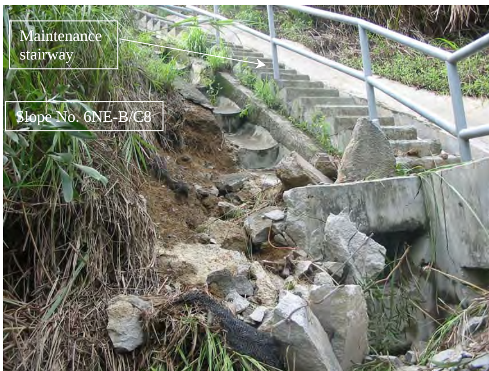
Plate A9 - View Showing a Catchpit Damaged by the Fallen Boulder (Photograph taken on 6 May 2003)
