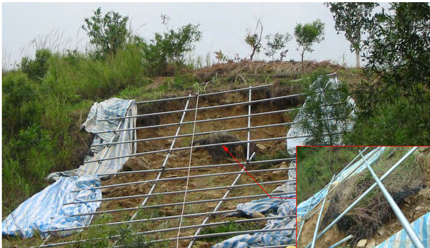
Plate 11 - Close-up View of the 5 May 2003 Landslide (Photograph taken on 16 May 2003)
