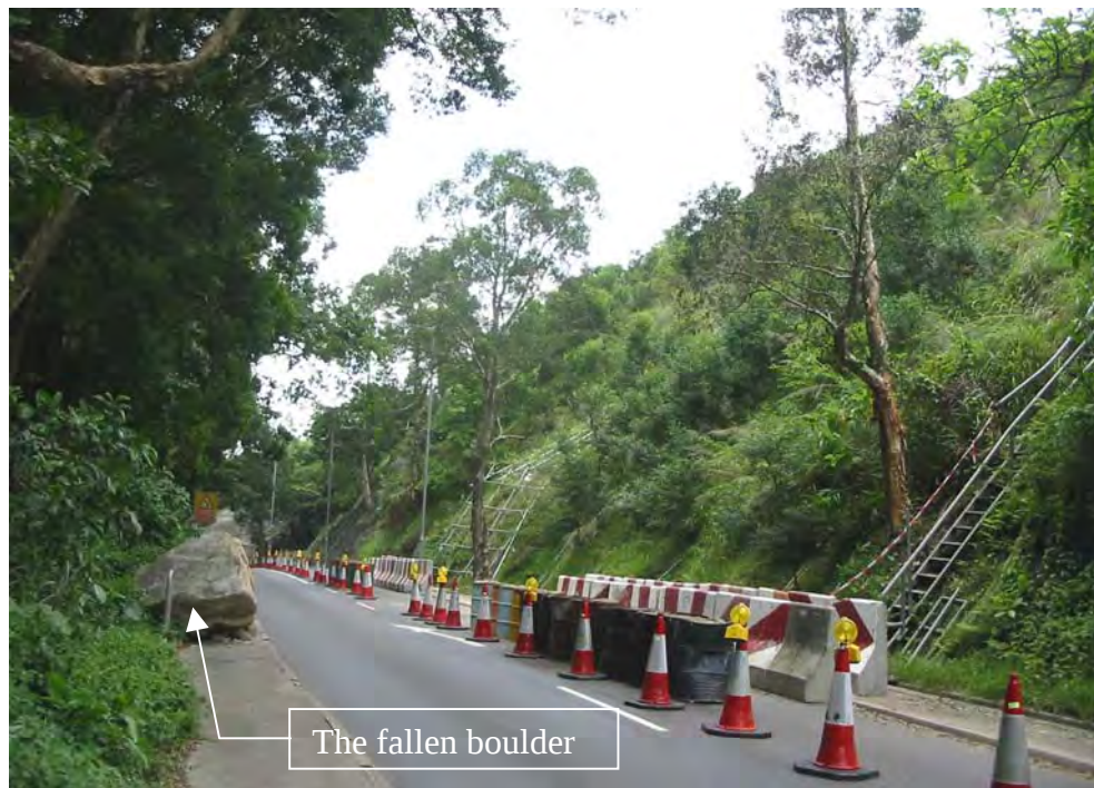
Plate A2 - General View of Slope No. 6NE-B/C8 and the Fallen Boulder (Photograph taken on 16 May 2003)
