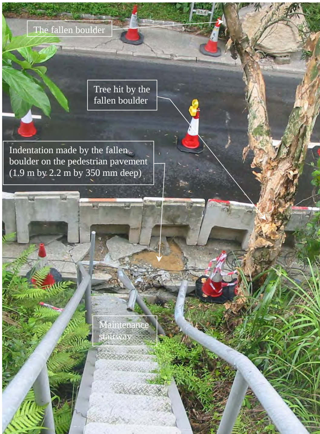
Plate A10 - View of the Maintenance Stairway and Pedestrian Pavement Damaged by the Fallen Boulder (Photograph taken on 6 May 2003)
