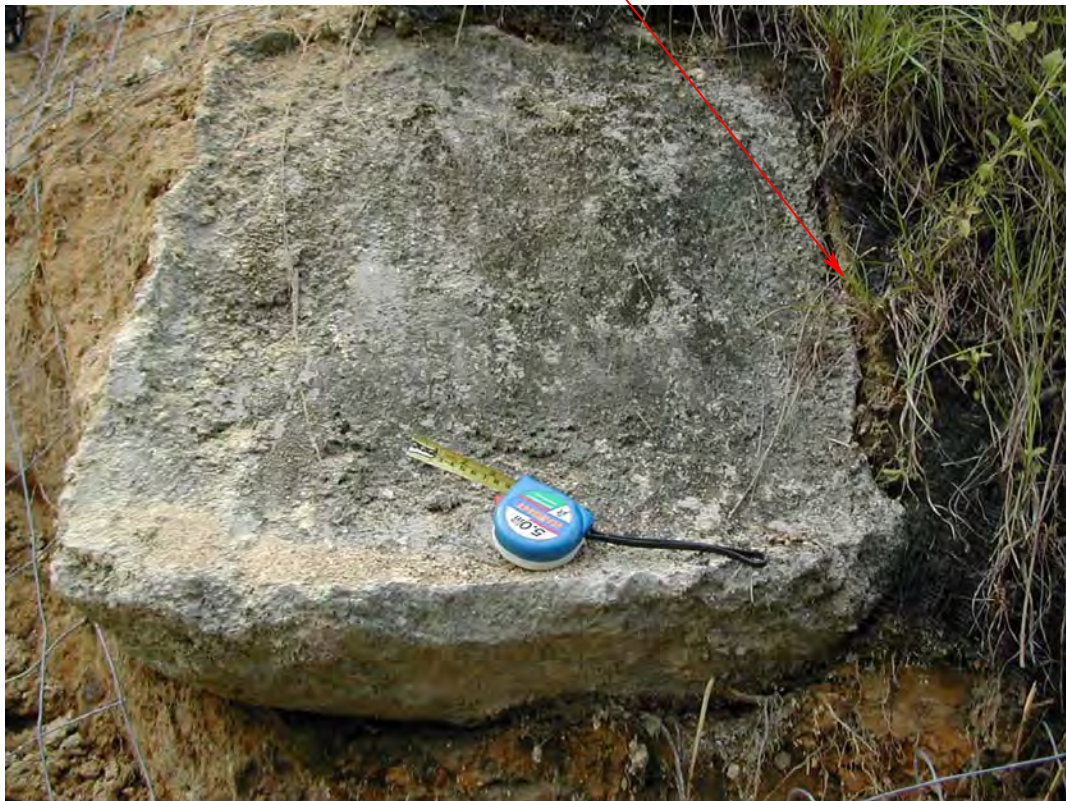
Plate 16 - Close-up View of a Gap between a Soil Nail Head and the Slope at the 13 June 2003 Landslide Site (Photograph taken on 19 June 2003)
