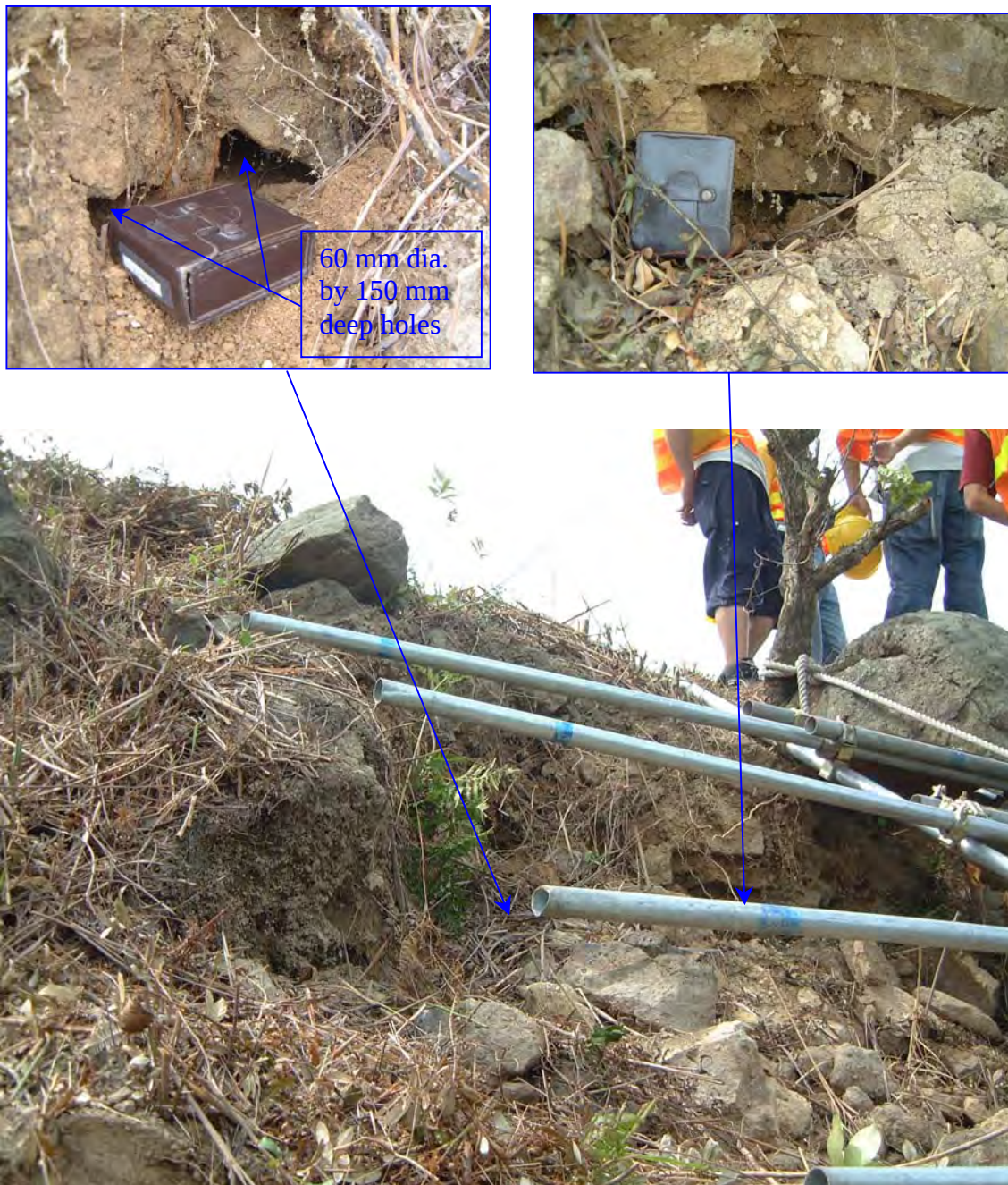
Plate A6 - Close-up View of the Source of the 5 May 2003 Boulder Fall after Vegetation Clearance (Photograph taken on 16 May 2003)
