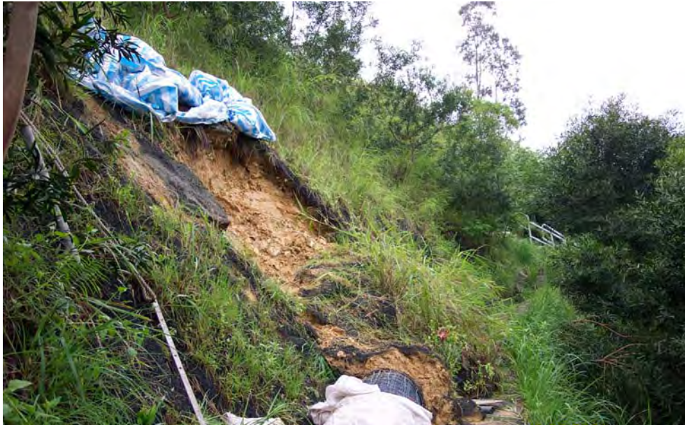
Plate 2 - View of the 13 June 2003 Landslide on Slope No. 6NE-B/C8 (Photograph taken on 14 June 2003)
