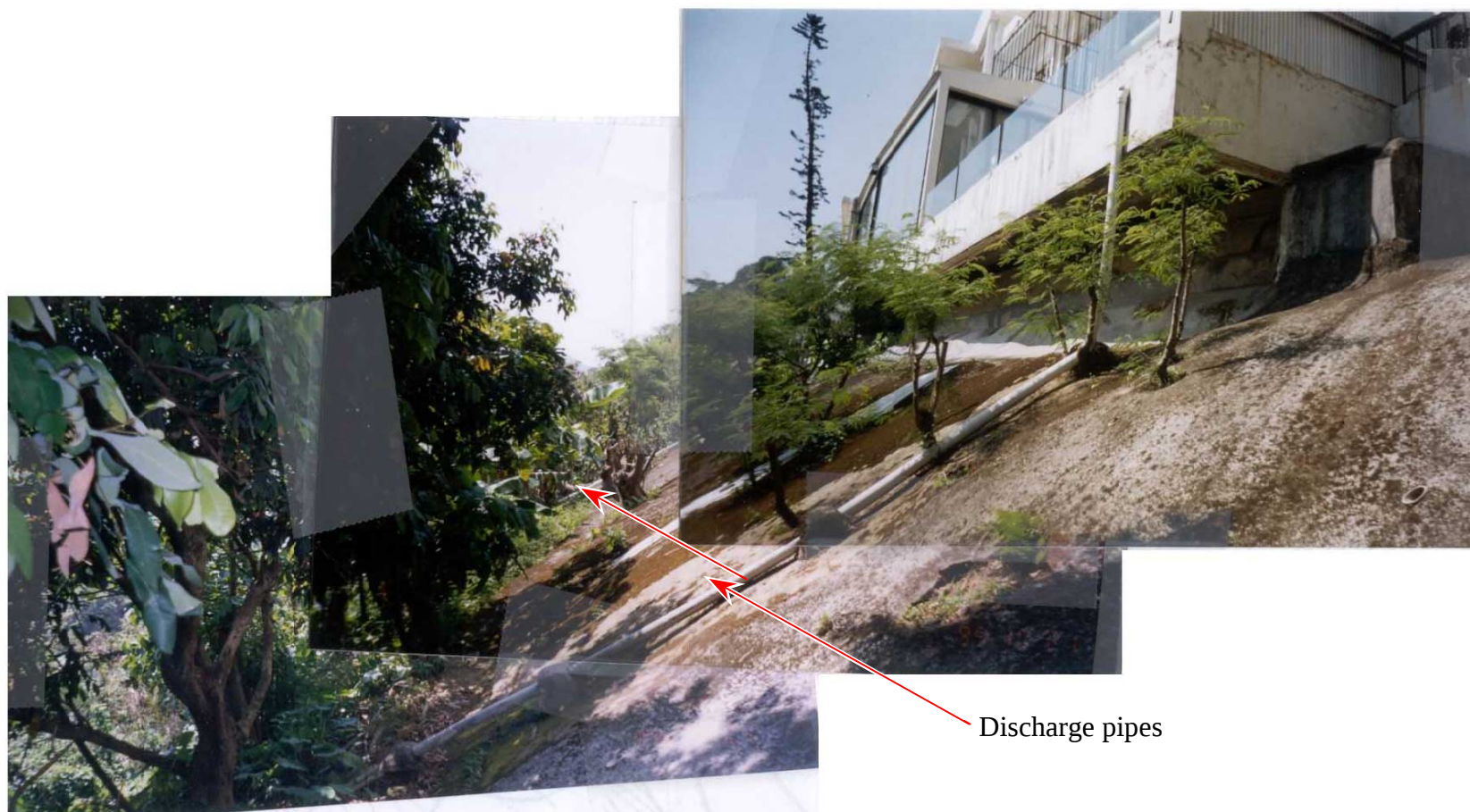
Plate 11 - Discharge Pipes from Platform of Albert Villa Discharged Directly to Hillside (Photograph Taken on 21 October 1999)
