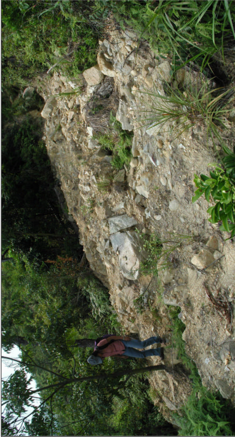
Plate 36 - View of Debris Lobe Below Landslide C between Chainages 45 and 60 (Photograph taken on 18 September 2000)
