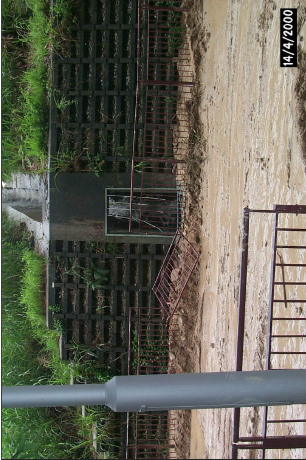
Plate 6 - View of the Alluvial Outwash Debris and Damaged Pedestrian Railing Below Drainage Line DC3 (Photograph taken by MCA on 14 April 2000)
