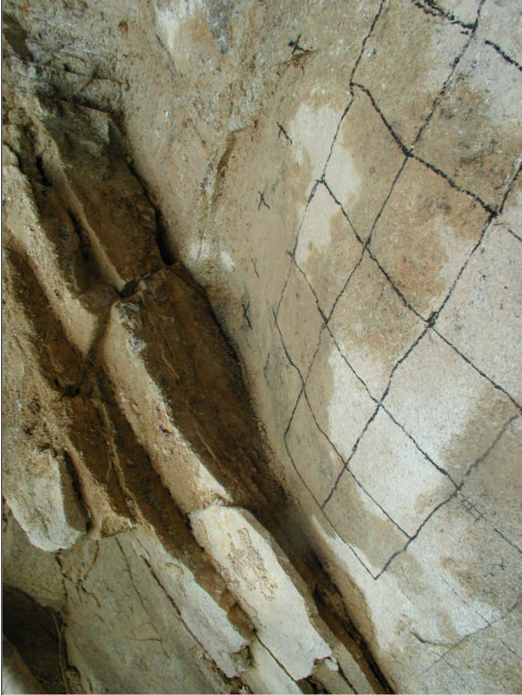
Plate 23 - Detail of Minor Seepage from Sheetting Joint Exposed on the Floor of Landslide B (Photograph taken on 28 October 2000)
