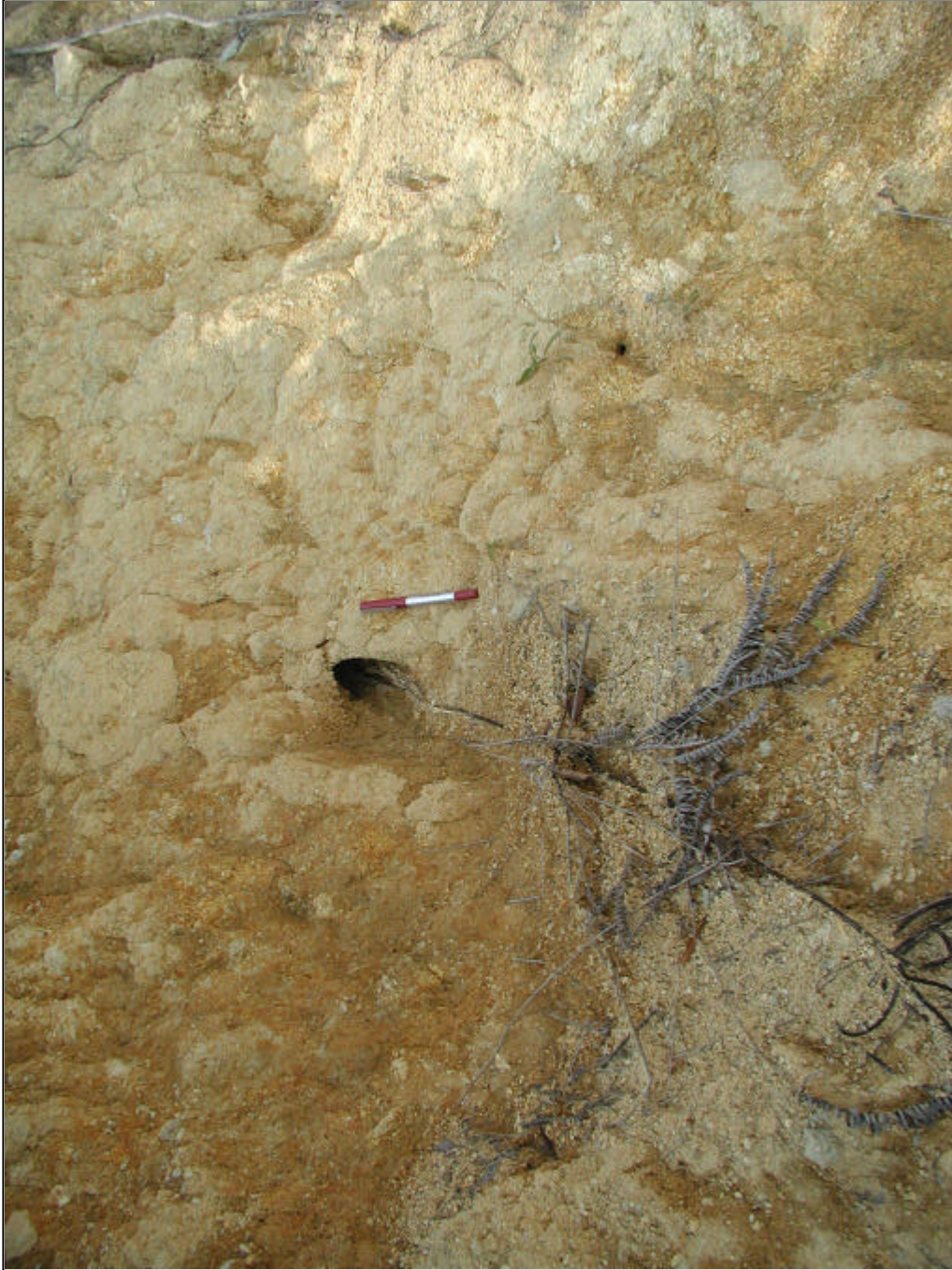
Plate 20 - Erosion Pipe Located on the Western Flank of Landslide B (Photograph taken on 24 October 2000)
