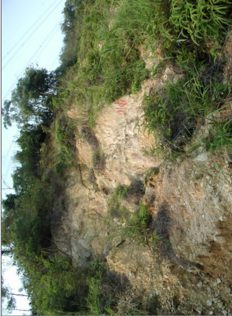
Plate 39 - General View of Landslide C3 (Photograph taken on 24 October 2000)
