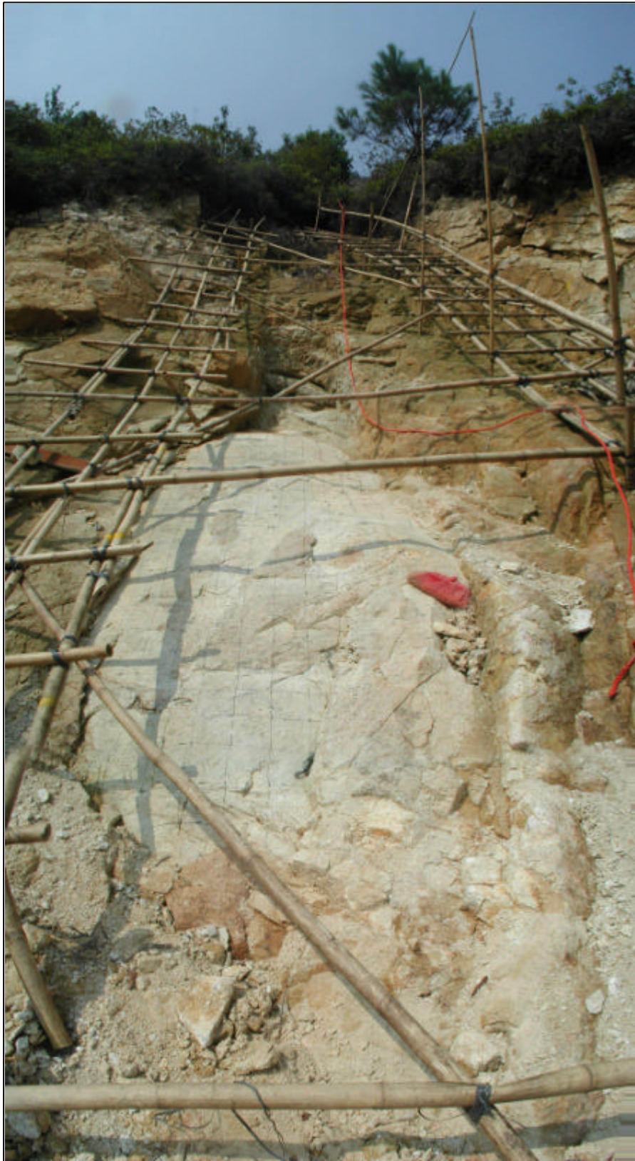
Plate 8 - View of the Floor of Landslide B (Photograph taken on 24 October 2000)
