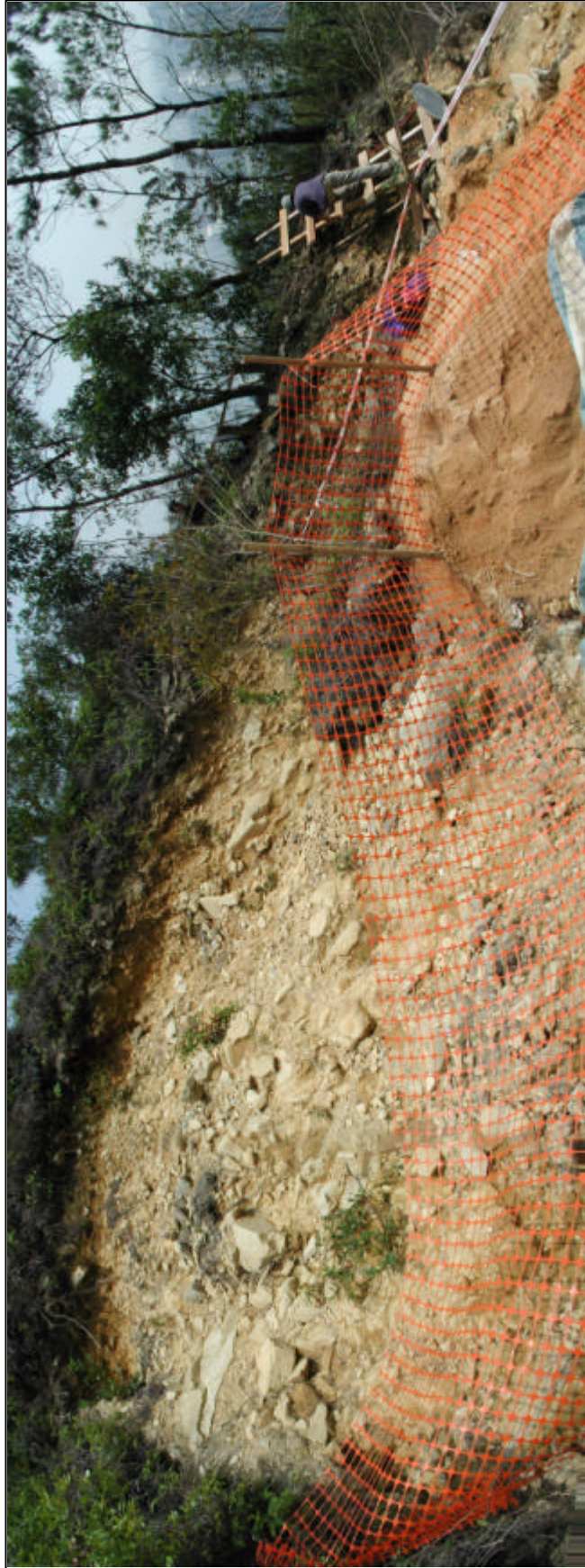
Plate 24 - Main Scarp of Landslide B1 (Photograph taken on 24 October 2000)
