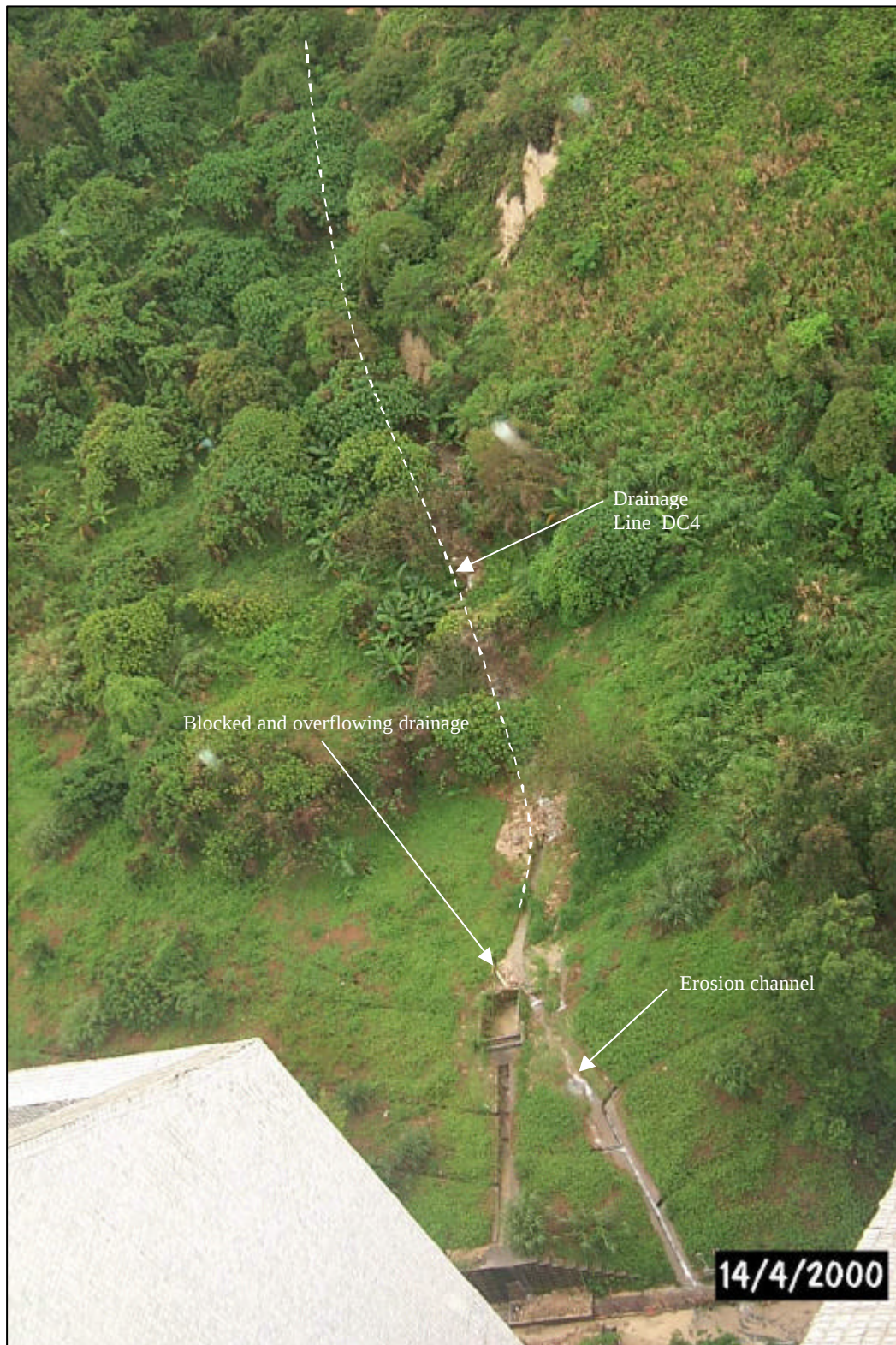
Plate 5 - View of the Blocked and Overflowing Slope Drainage Below the Source Area Landslide C (Photograph taken by MCA on 14 April 2000)
