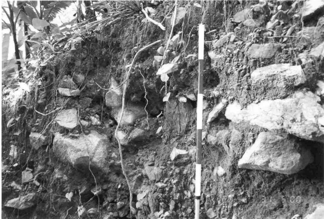
Plate A6 – View of Loose/Voided Colluvium Exposed in the Flank of the Drainage Line at about Chainage 120 m
