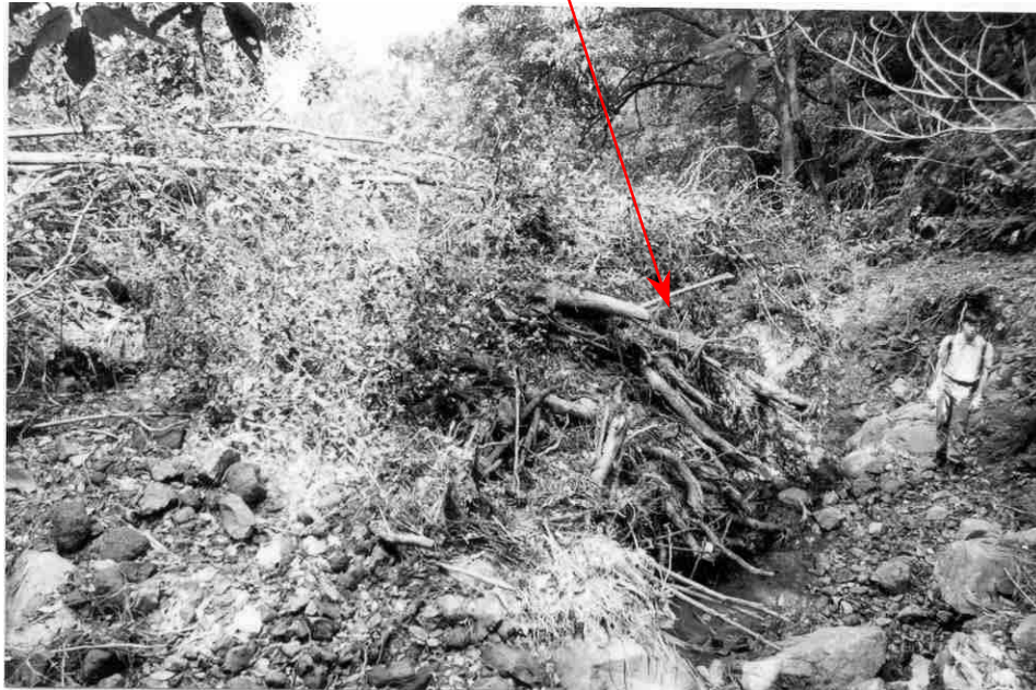
Plate A4 – View Looking Downslope of Localised Accumulation of Debris at Chainage 210 m
