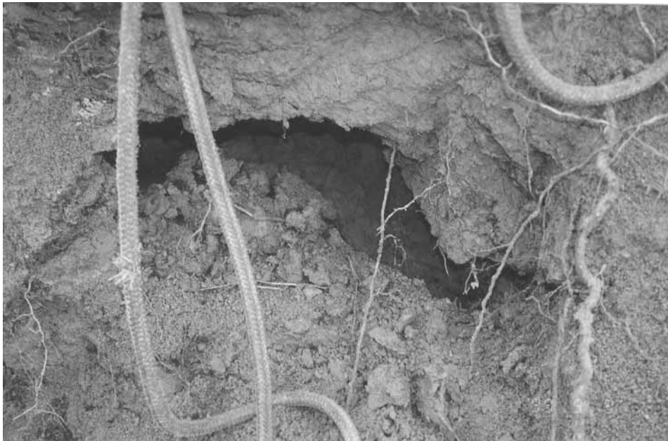
Plate 10 – Soil Pipe Exposed behind the Main Scarp Following Trimming (Photograph Taken on 9 September 1999. See Figure 11 for Location)
