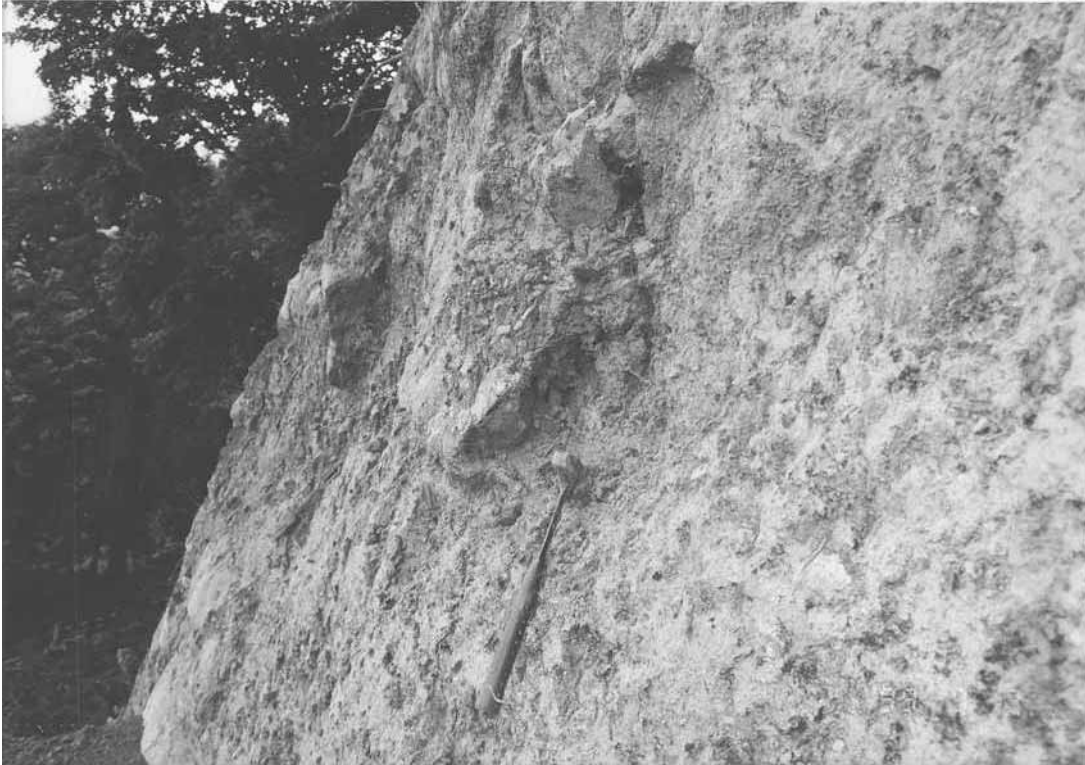
Plate 13 – Previous Tension Crack/Joint Infilling Exposed along Release Planes on Eastern Flank of the Scar (Photograph Taken on 2 September 1999. See Figure 11 for Location)
