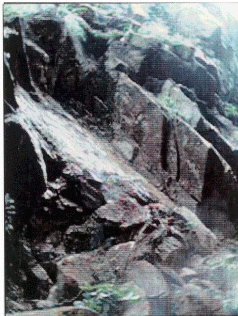
Plate 2 - View to Southeast Showing the Failure Scar and Sliding Surface of Incident No. MW97/5/6 (Photograph Taken on 8 May 1997)
