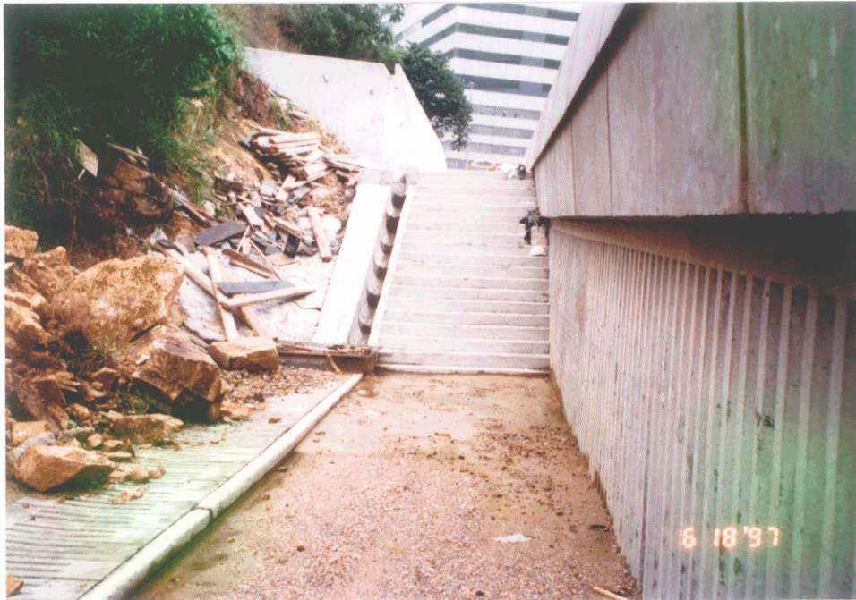
Plate 3 - View of Debris at Slope Toe from Incident No. MW97/6/21 (Photograph Taken on 18 June 1997)
