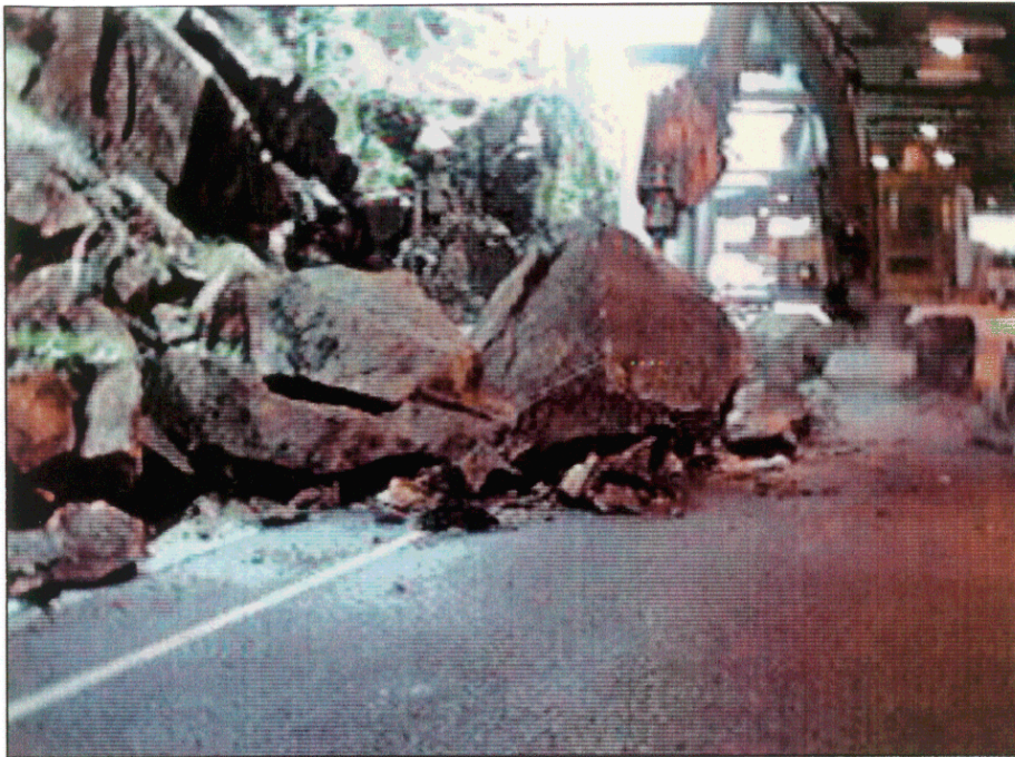
Plate 1 - View to Southeast of Landslide Debris on the Kowloon-bound Carriageway of Kwai Chung Road, Incident No. MW97/5/6 (Photograph Taken on 8 May 1997)
