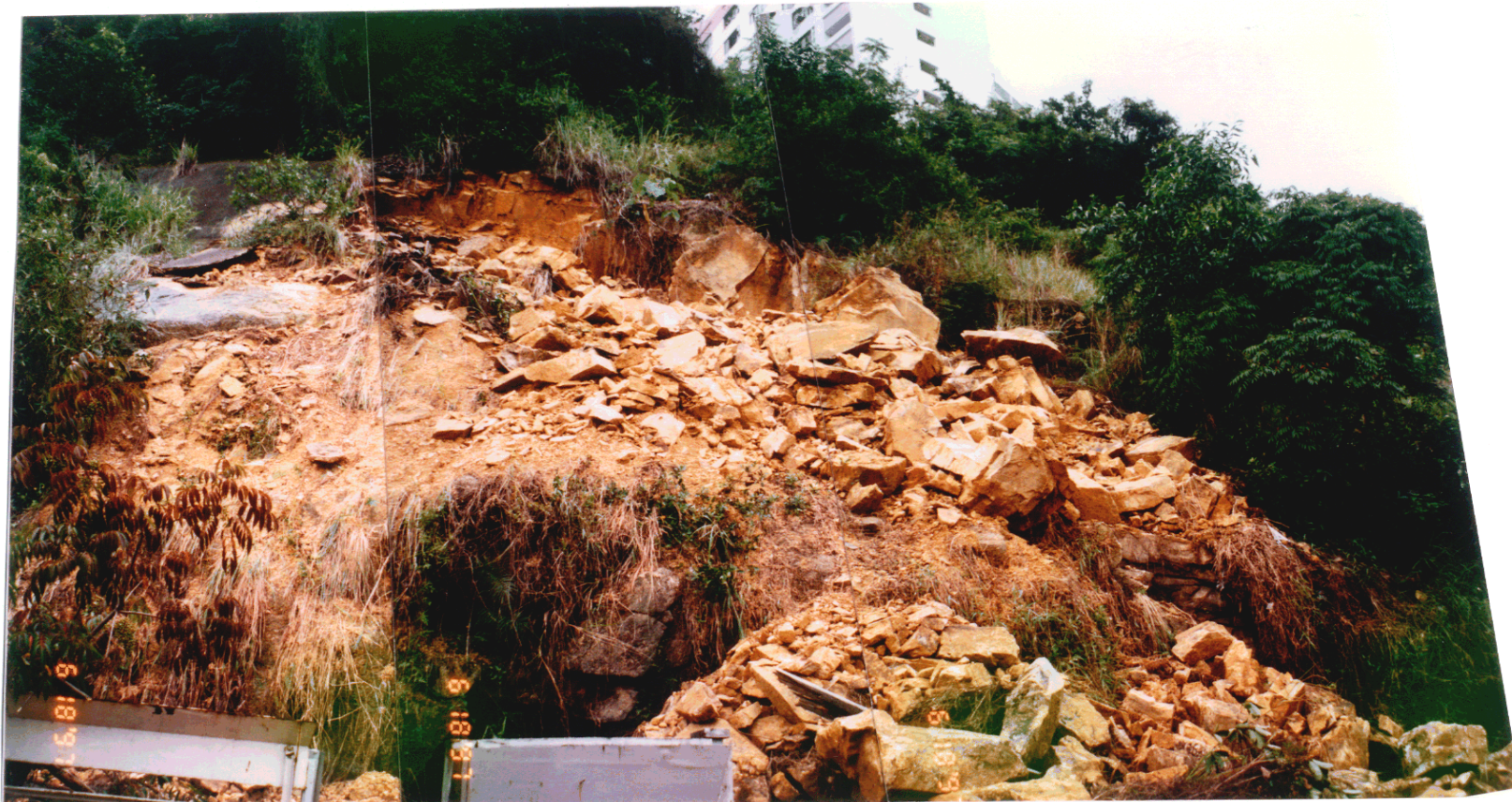
Plate 5 - Detailed View of Incident No. MW97/6/21 (Photograph Taken on 18 June 1997)
