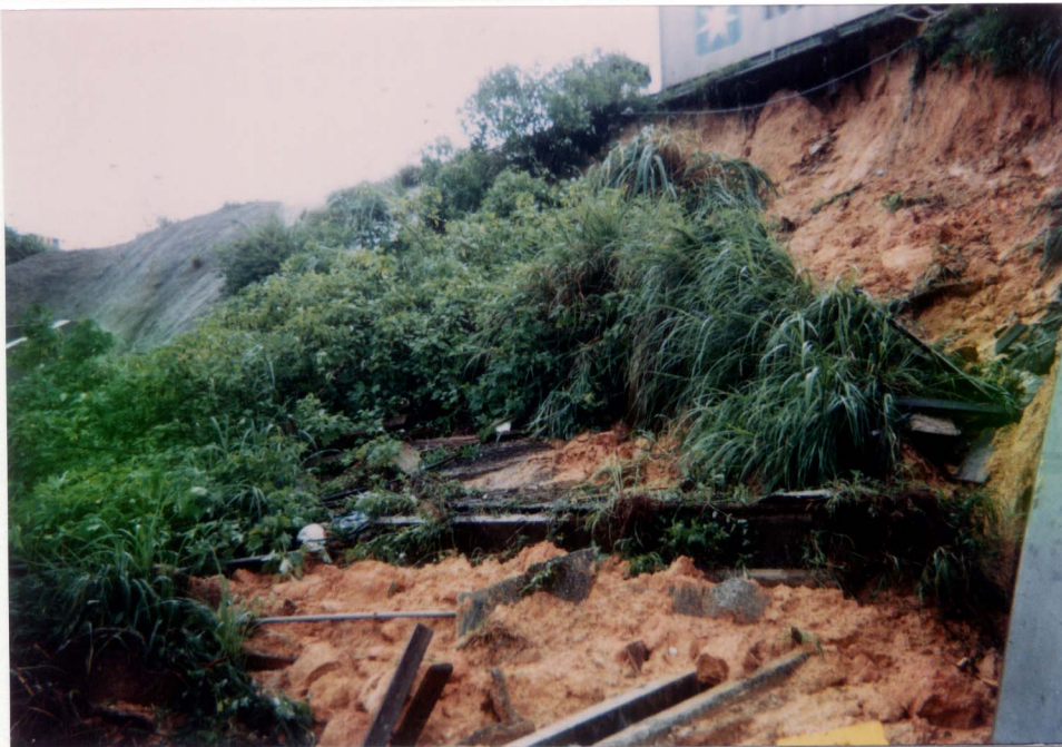
Plate 3 - View of the Eastern Flank of the Landslide (Photograph Taken on 2 July 1997. Note the Sections of Broken U-channel in the Debris)
