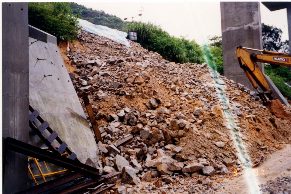
Plate 9 - Close-up of the Urgent Repair Works Showing the Main Scarp Infilled with Rockfill (Photograph Taken on 3 July 1997)
