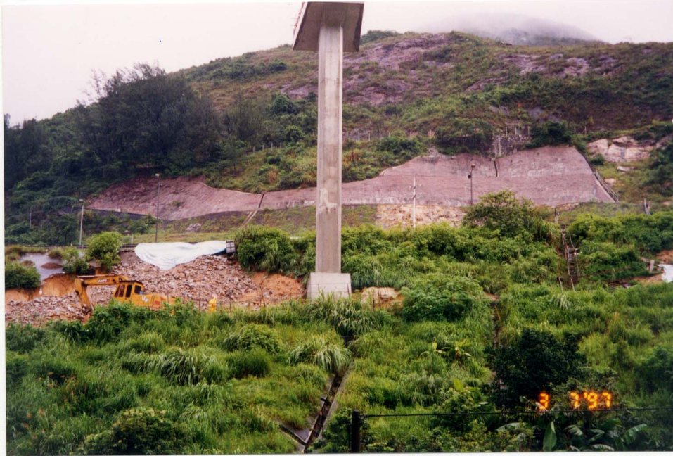
Plate 8 - View Showing the Urgent Repair Works (Photograph Taken on 3 July 1997. Note the Vegetation Covering the Slope to the East of the Landslide and Chunam Covering the Slope to the West of the Landslide)
