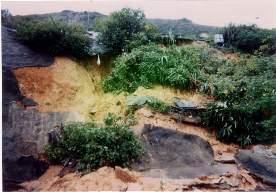
Plate 4 - View to the Western Flank of the Landslide (Photograph Taken on 2 July 1997. Note the Broken Chunam Surfacing in the Debris)
