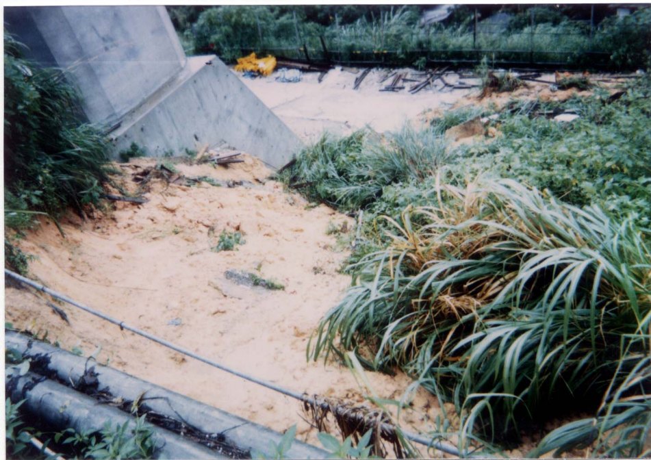
Plate 5 - View from the Crest of the Landslide (Photograph Taken on 2 July 1997. Note the Small Water Pipe and the Two Cable Conduits Exposed by the Landslide)
