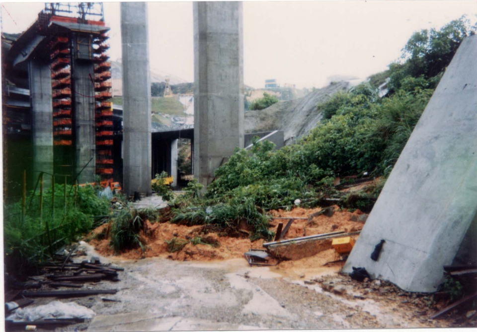
Plate 2 - View to the West Along the Access Road Which was Blocked with Landslide Debris (Photograph Taken on 2 July 1997. Note Bridge Pier D2/3 in the Foreground and Bridge Pier D2/2 in the Centre of the Photograph)
