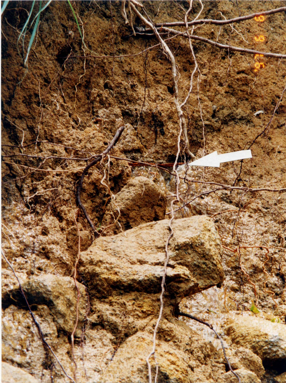
Plate 8 - An Erosion Pipe in the Main Scarp of Landslide B (Photograph Taken on 6 June 1997. Note the Arrow Points to Flowing Water Issuing from the Pipe in the Centre of the Photograph)
