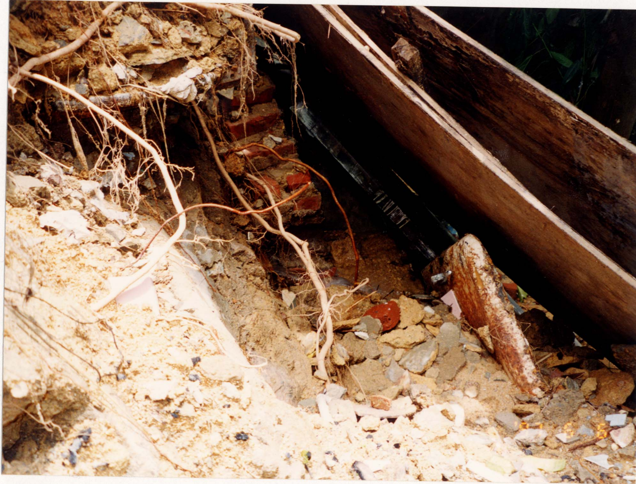
Plate 11 - View of the Thin Brick Retaining Wall Involved in Landslide C (Photograph Taken on 6 June 1997)
