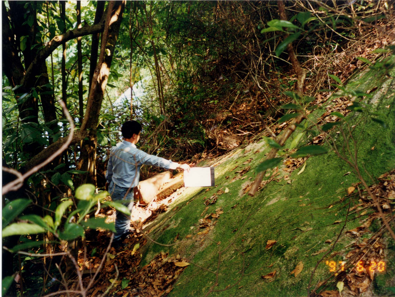
Plate 2 - A Sheeting Joint Rock Surface Above Landslide A (Photograph Taken on 20 June 1997)
