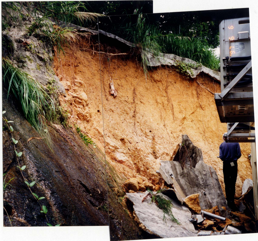
Plate 7 - View of Landslide B (Photograph Taken on 6 June 1997. Note the Water Flowing on the Steep Sheeting Joint Surface Below the Failed Soil Cut Slope)
