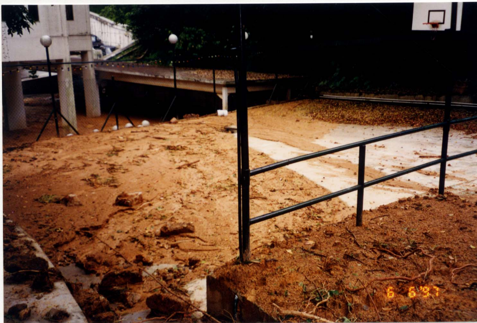
Plate 12 - View of Debris Run-out at Toe of Slope Following Incident No. MW97/6/23 (Photograph Taken on 6 June 1997)
