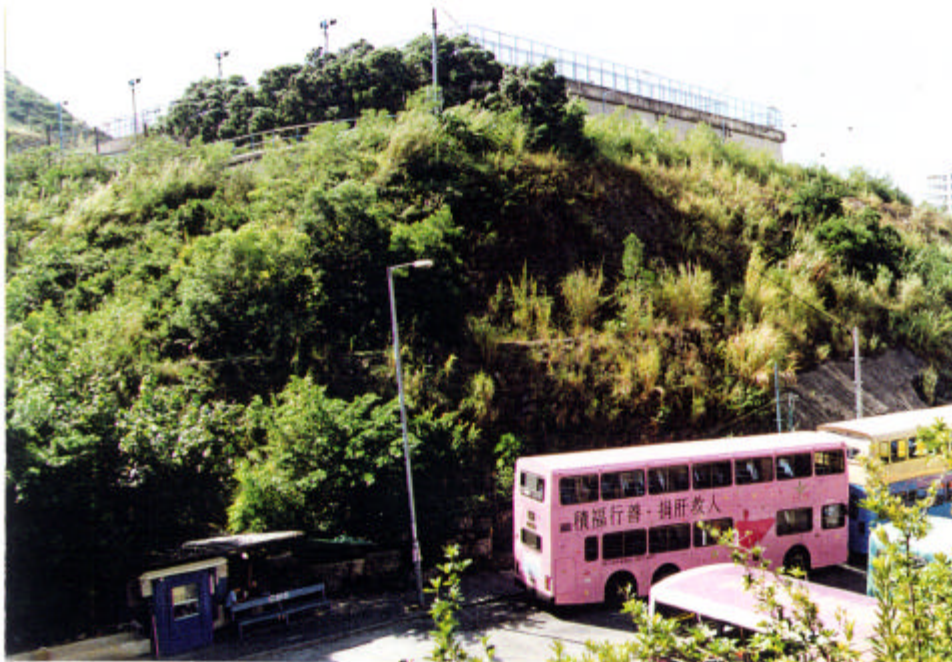
Plate 9 - Slope 15NW-B/C92 (834100E 811300N), by the Bus Terminus at Lei Tung Estate, in Decomposed Siliceous Fine Ash Tuff with Extensive Kaolinitic Clay Infills in Relict Joints within Grade IV/V Decomposed Bedrock. (Taken 12/11/96)
