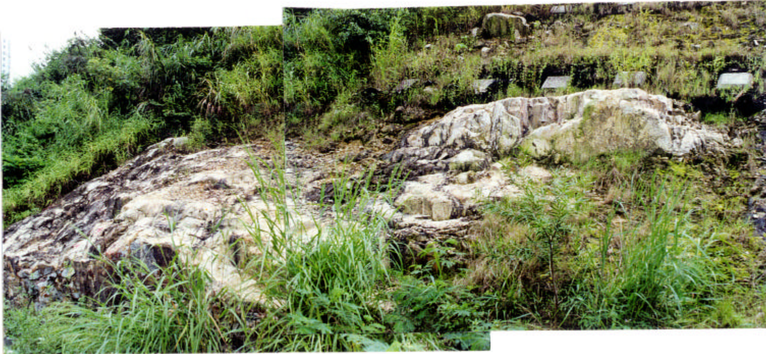
Plate 3 - Unregistered Slope (833550E 811500N) on Road Leading to Water Service Reservoir within Eutaxitic Fine Ash Vitric Tuff, Showing the Development of Subhorizontal and Inclined (Parallel to the Natural Slope) Stress Release Joints and Their Relationship to the Interface Between the PW90/100 and PW0/30 Rock Mass Weathering Zones. (Taken 1/10/96)
