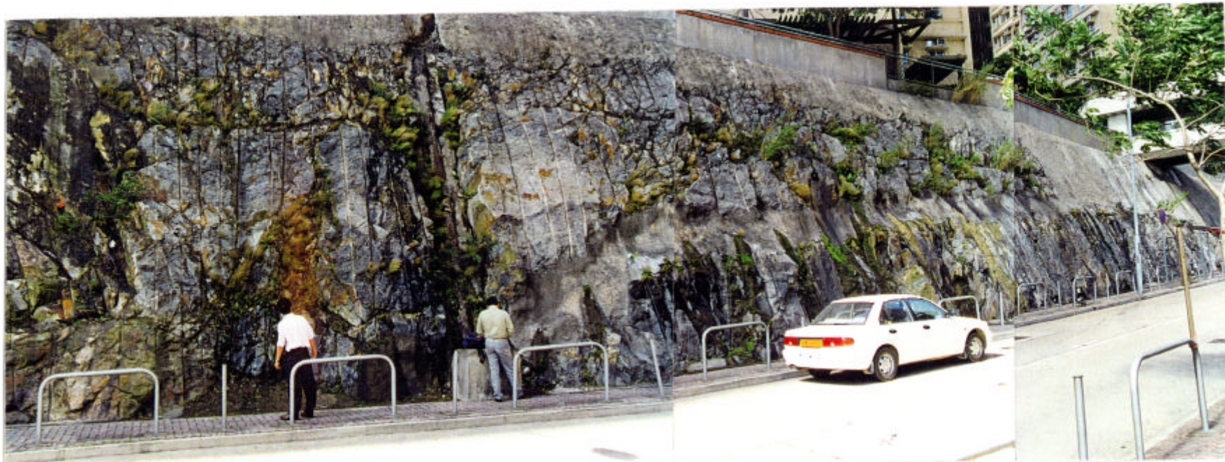
Plate 6 - Unregistered Slope 15NW-3B/S10 (834250E 811530N), in Lei Tung Estate Showing a Relatively Planar Weathered Seam (Largely Covered by Chunam) of Kaolinitic Clay, c.150 mm Thick, Dipping c.30-35° out of the Slope at about Mid-height within Grade II Tuff. Extensive Groundwater Seepage was Noted from the Seam during Site Inspection. (Taken 12/11/96)
