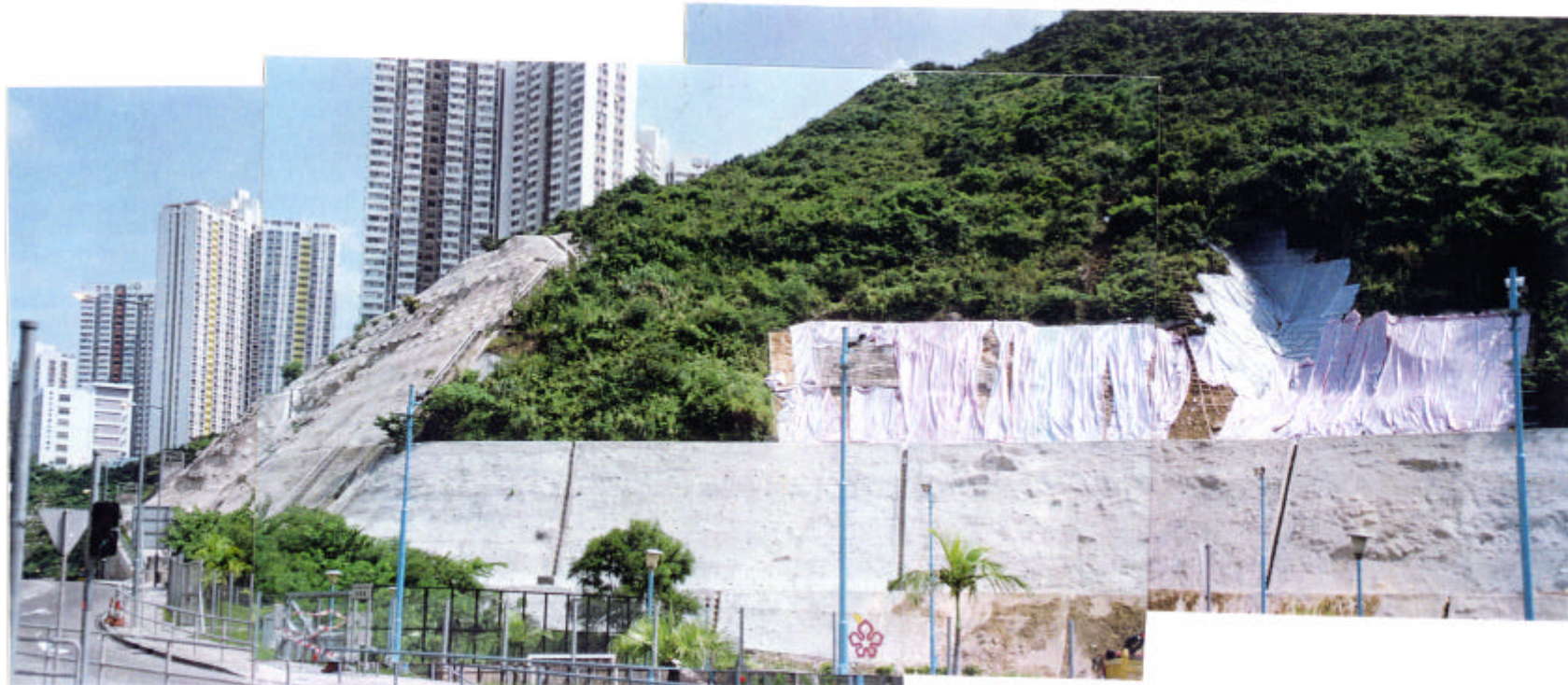
Plate 7 - Slope 15NW-A/C1, Corner of Ap Lei Chau Bridge Road and Lee Nam Road (833650E 811620N). Completely to Highly Decomposed Tuff with Many Relict Joints Infilled with Kaolinitic Clay. Six Landslide Incidents Have Occurred in This Slope Between 1993 and 1996, the Most Recent (Right-Hand Side Covered by Sheeting) Occurred on 5/9/96. (Taken 1/10/96)
