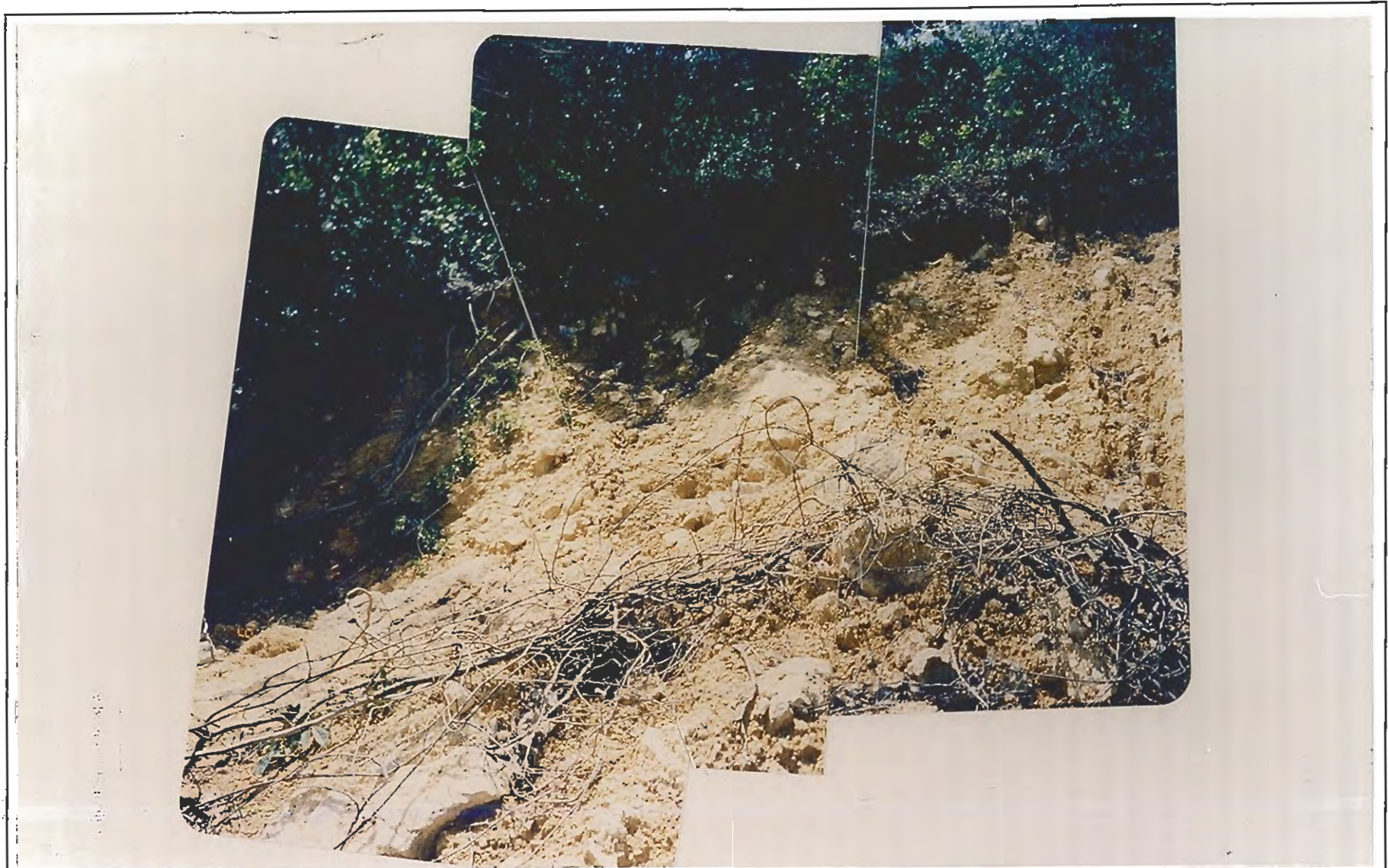
Plate B8.6 - Close-up of Main Scarp B8
