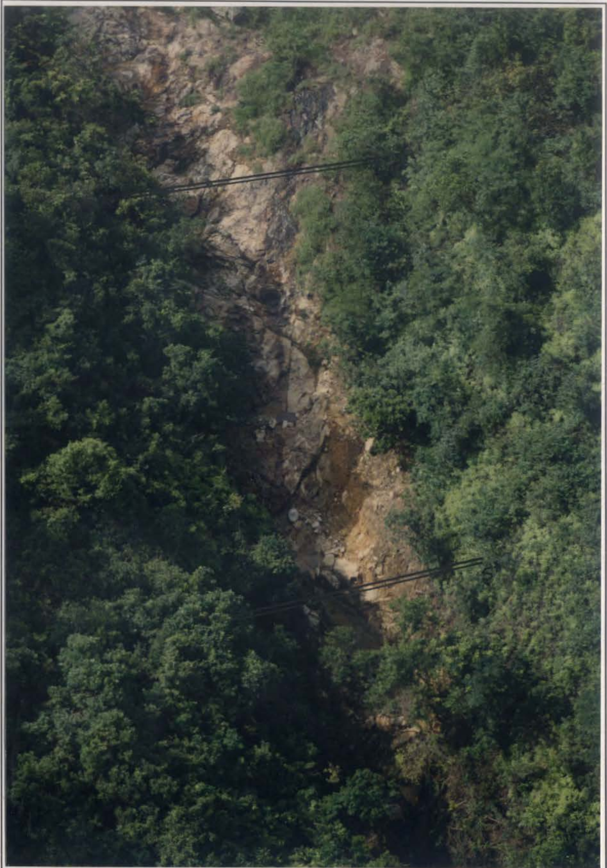
Plate B2.8 - Debris Trail (CH290 - CH320) of Landslide B2
