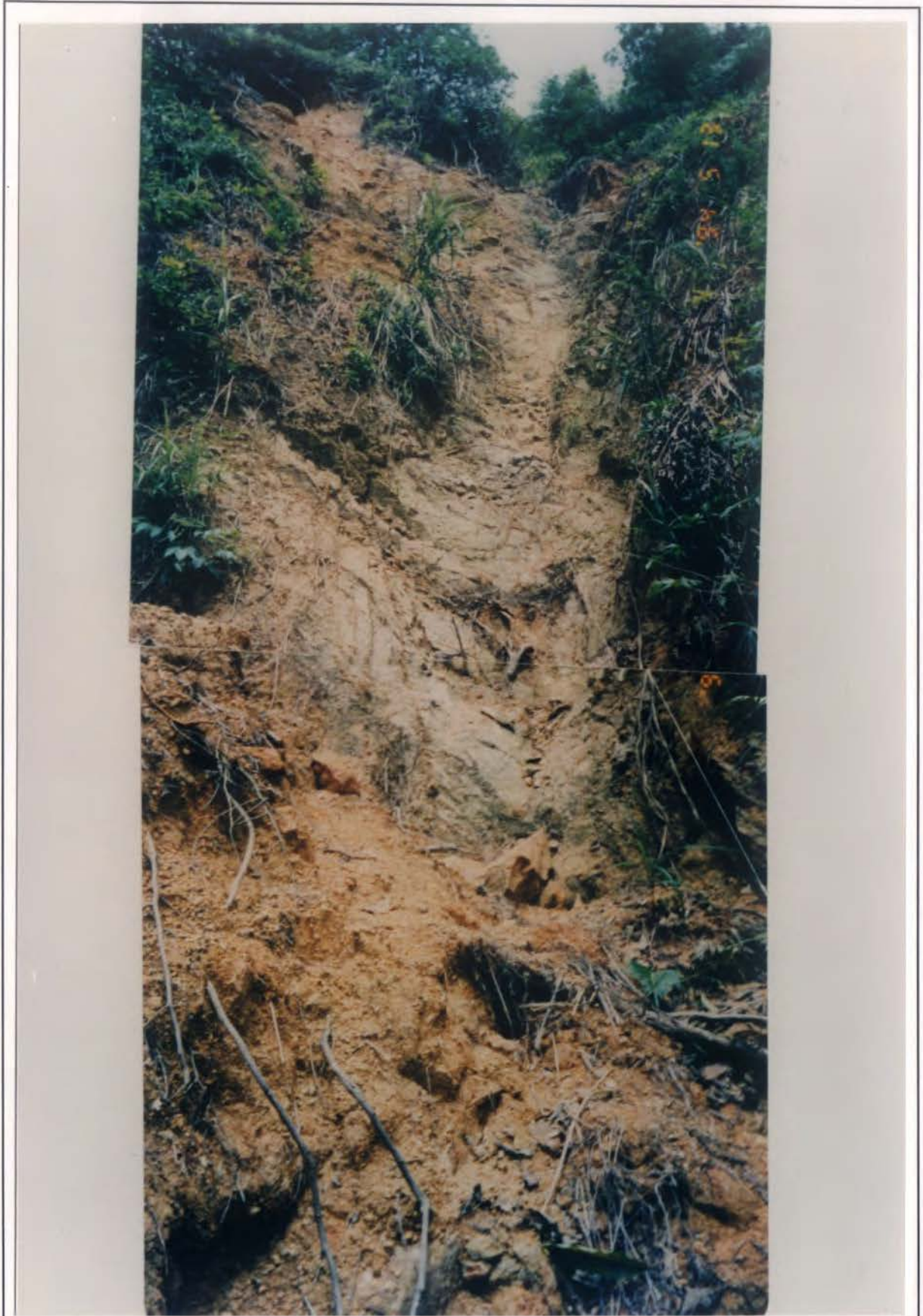
Plate B3.17 - Uphill View of Landslide B3D
