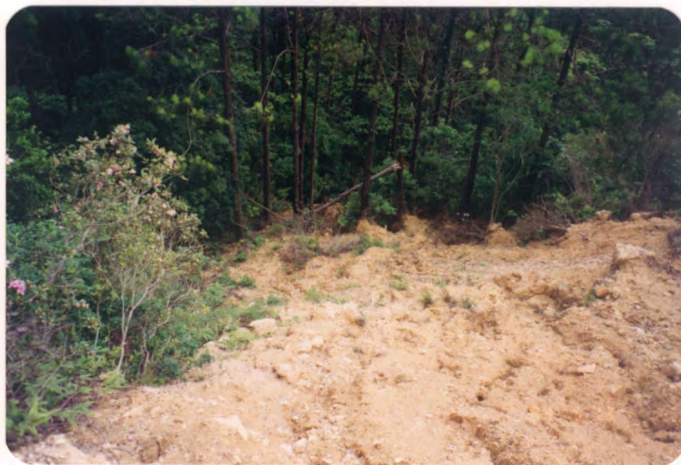
Plate B6.8 - Toe of Debris Trail of Landslide B6
