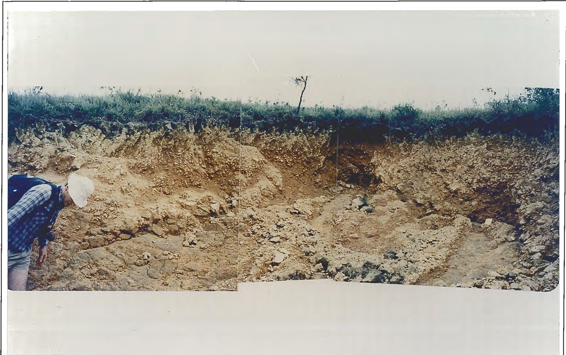
Plate C4 - Main Scarp of Landslide C1
