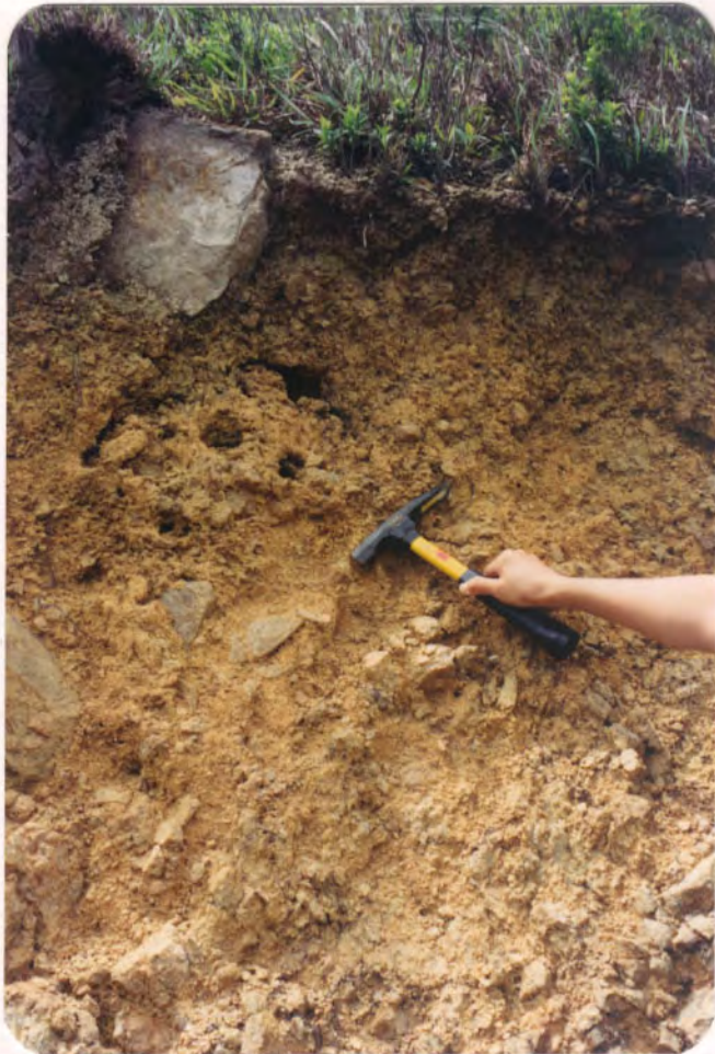
Plate B5.14 - Pipe Holes at Main Scarp B5B
