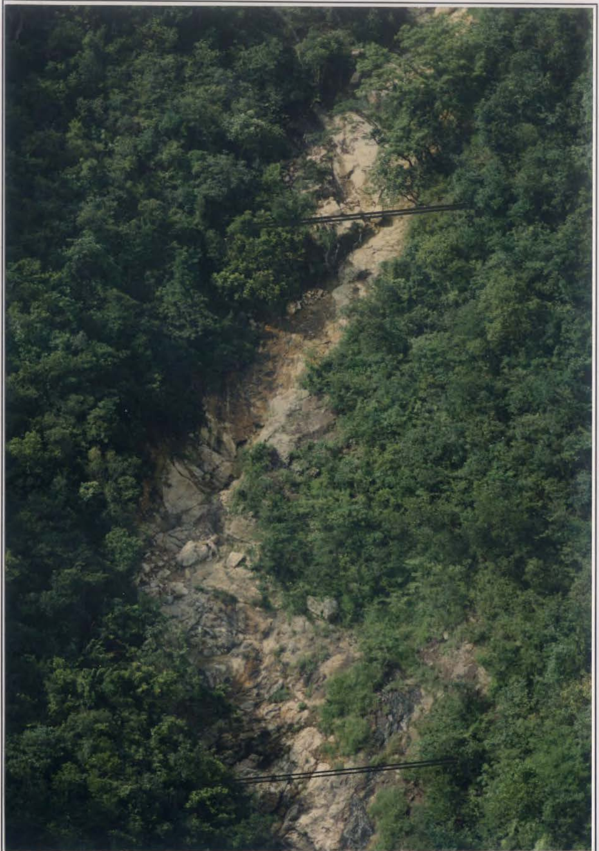
Plate B2.7 - Debris Trail (CH260 - CH290) of Landslide B2
