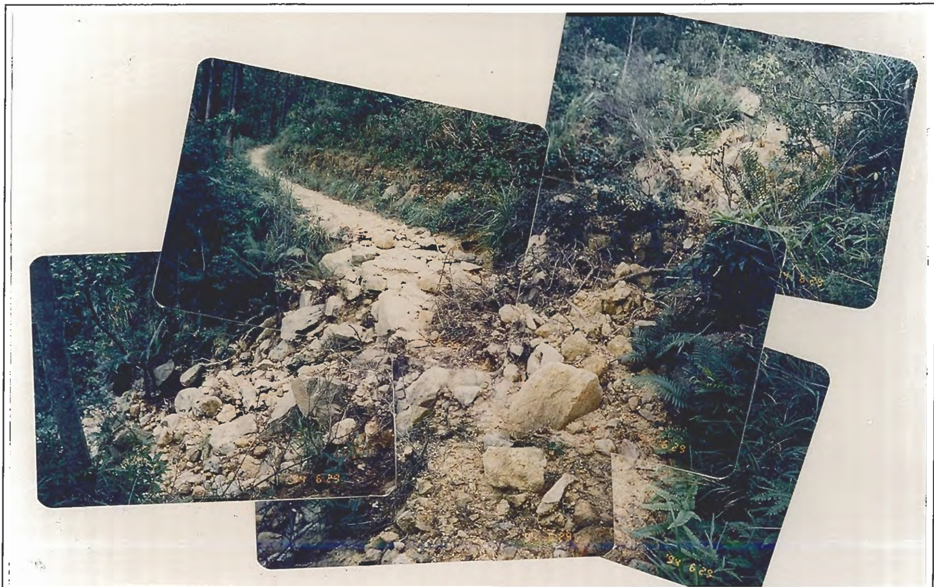
Plate B11.7 - Debris Trail of Landslide B11 at Footpath Level
