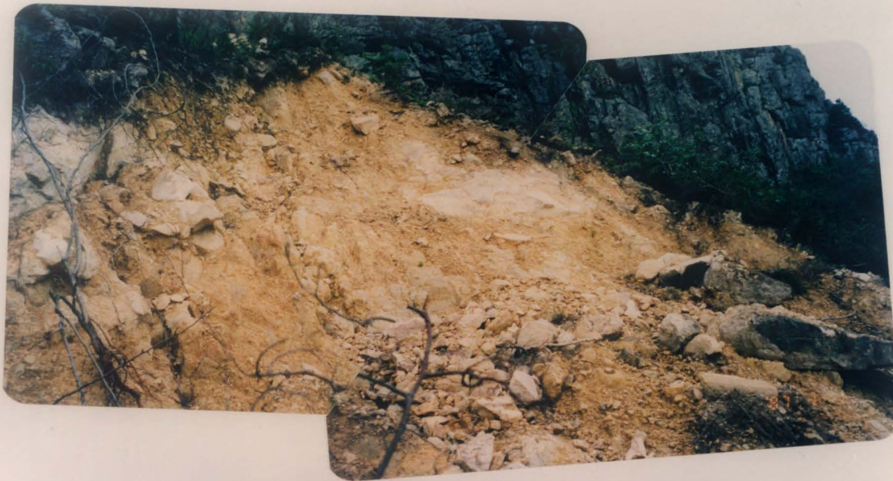
Plate B2.11 - Close-up of Main Scarp B2A
