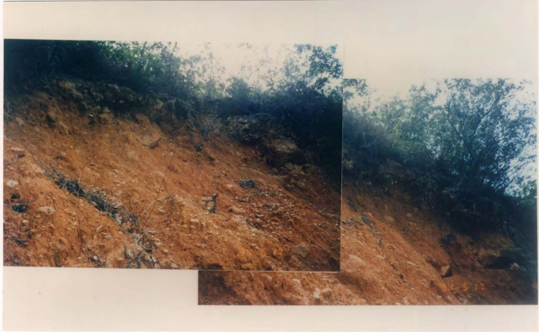
Plate B3.5 - Close-up of Main Scarp B3A
