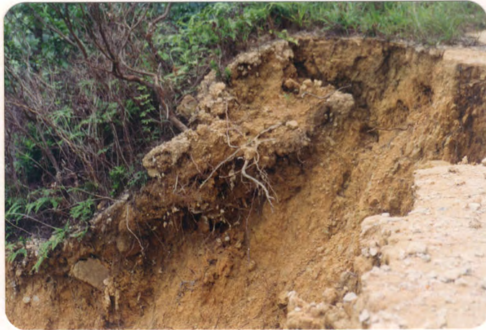
Plate B6.5 - Crown of Landslide B6
