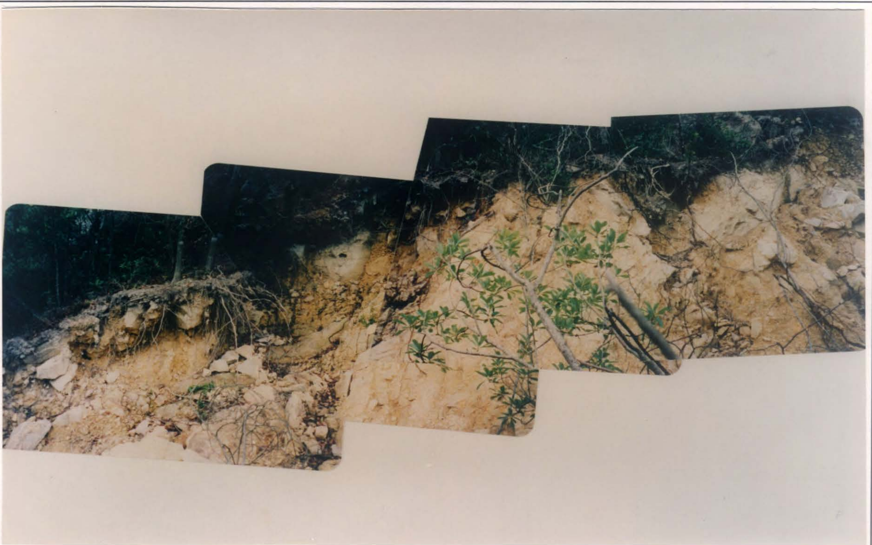
Plate B2.13 - Close-up of Main Scarp B2A
