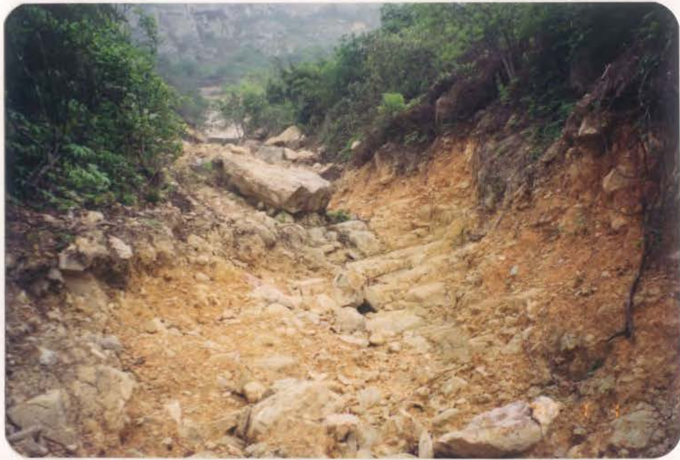
Plate B2.26 - Downhill View of Erosion Gully along Debris Trail of Landslide B2
