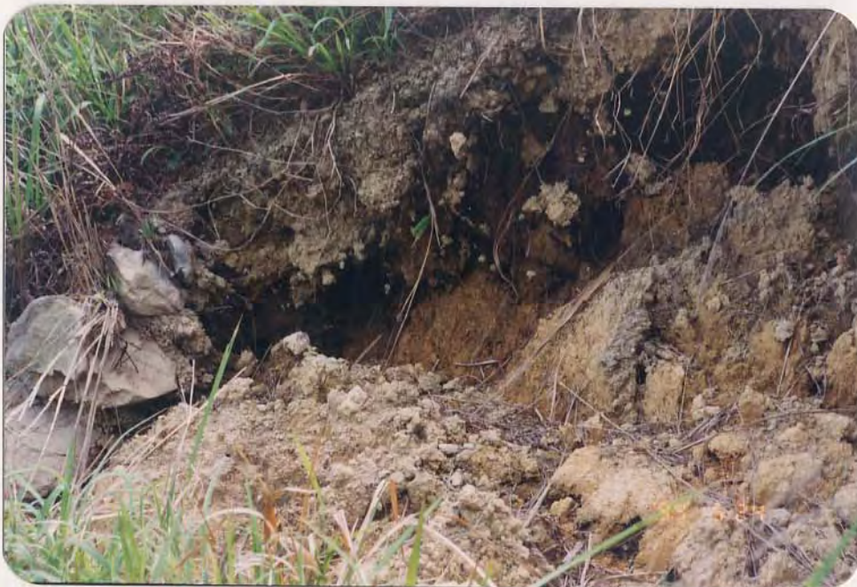
Plate A9.4 - Pipe Holes at Minor Landslide Adjacent to Footpath
