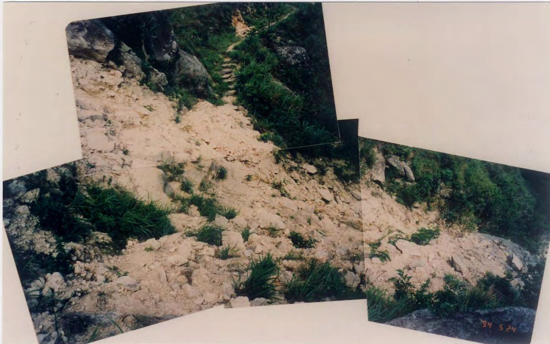
Plate A7.4 - View of Debris Trail of Landslide A7 at Footpath Level
