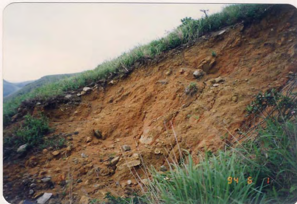
Plate A13.9 - Close-up of Crown of Landslide A13A
