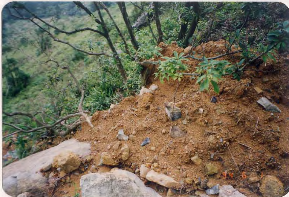
Plate A13.4 - Deposition of Debris along Debris Trail of Landslide A13A
