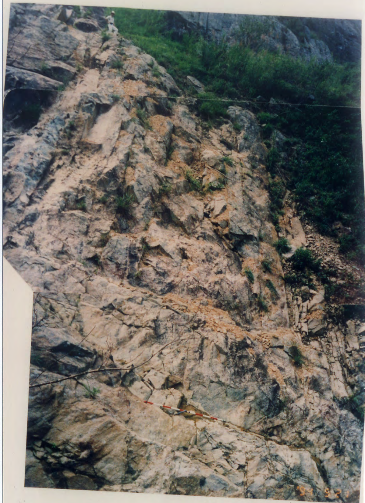
Plate A1.11 - View of Rock Cliff along Debris Trail of Landslide A1B
