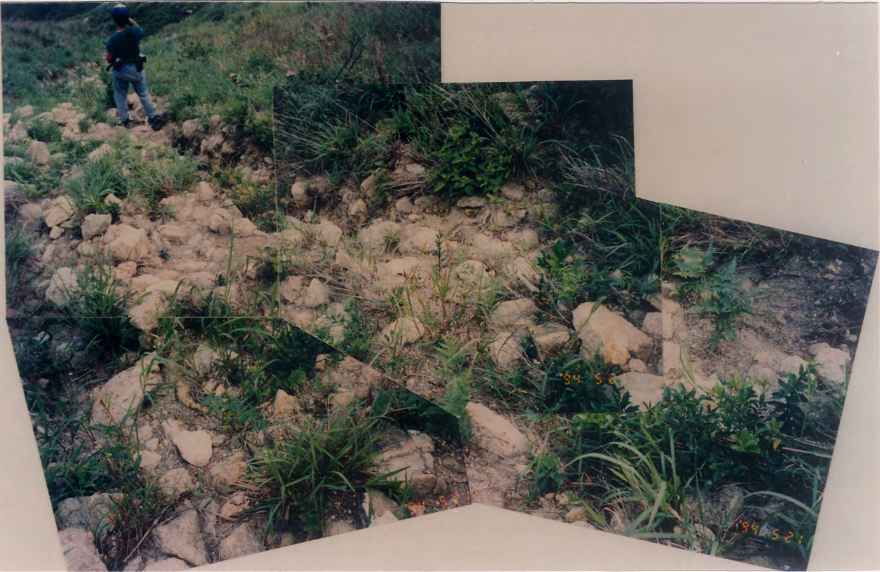
Plate A2.5 - Downhill View of Debris Trail of Landslide A2
