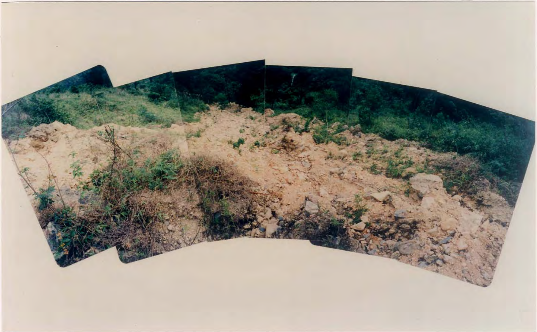
Plate A15.3 - Downhill View of Debris Trail of Landslide A15
