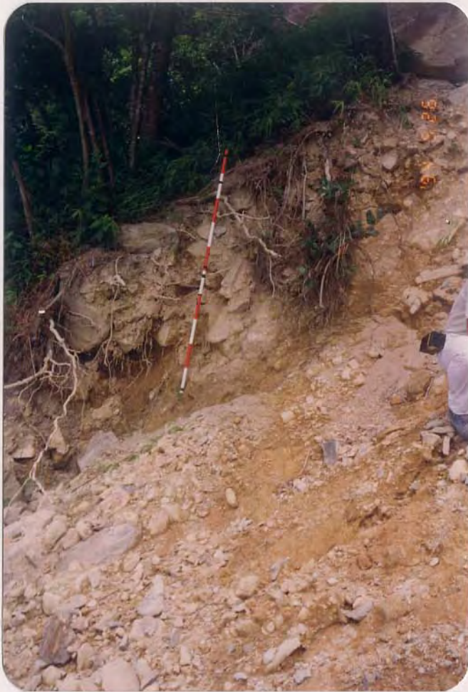
Plate A16.12 - Close-up of Soil Pipes in the Main Scarp of Landslide A16A
