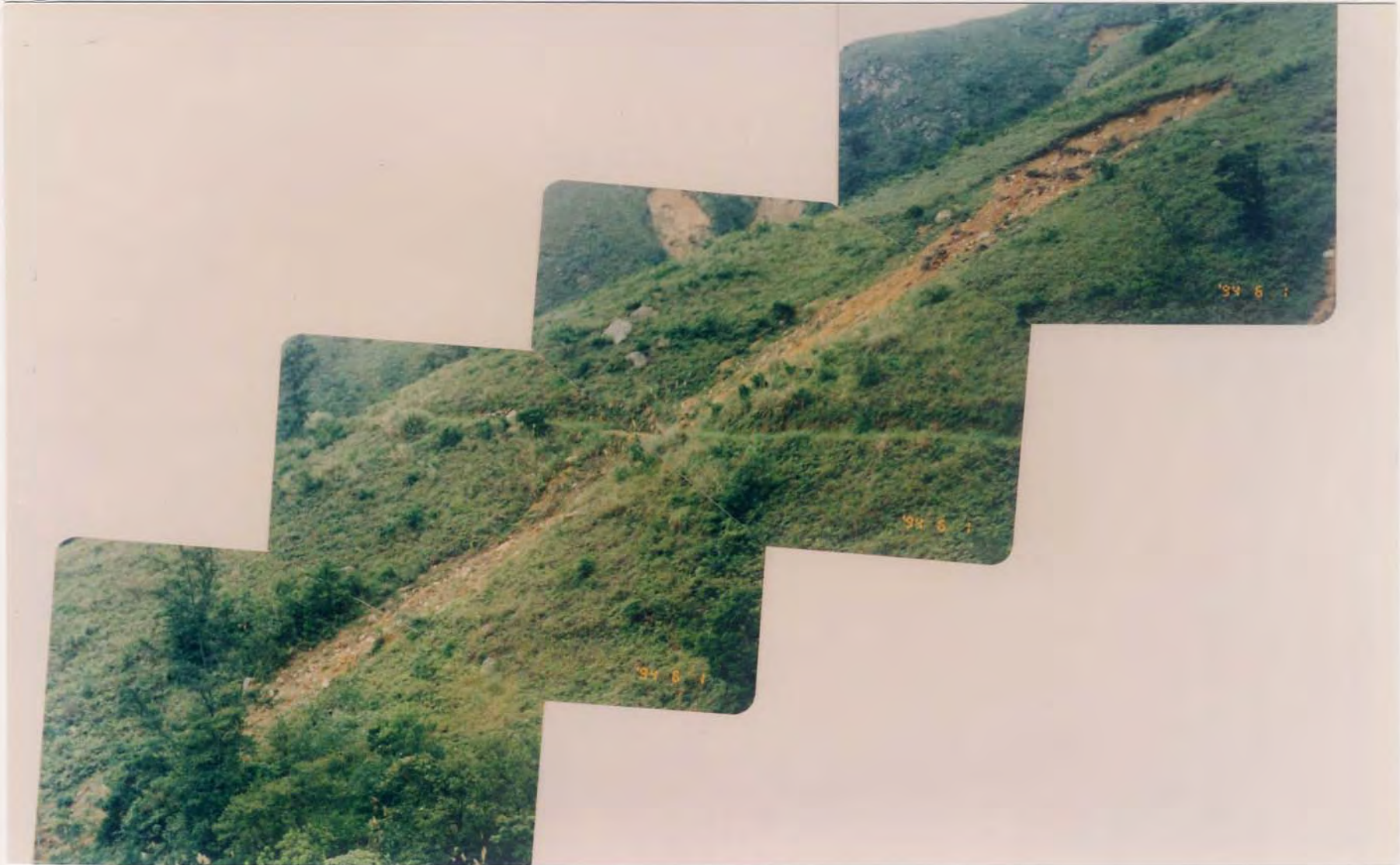
Plate A14.2 - Oblique View of Landslide A14
