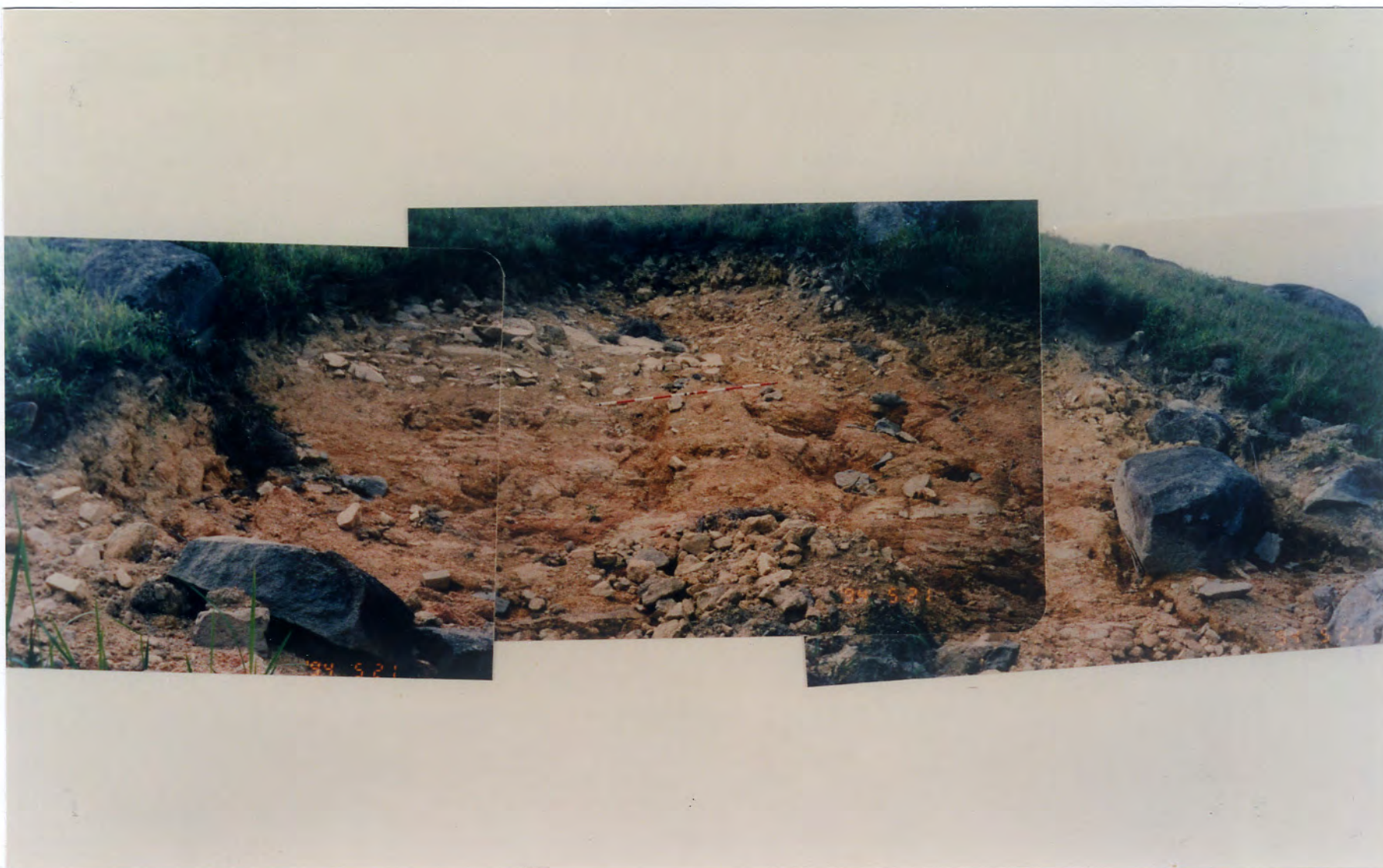
Plate A1.3 - Main Scarp of Landslide A1A
