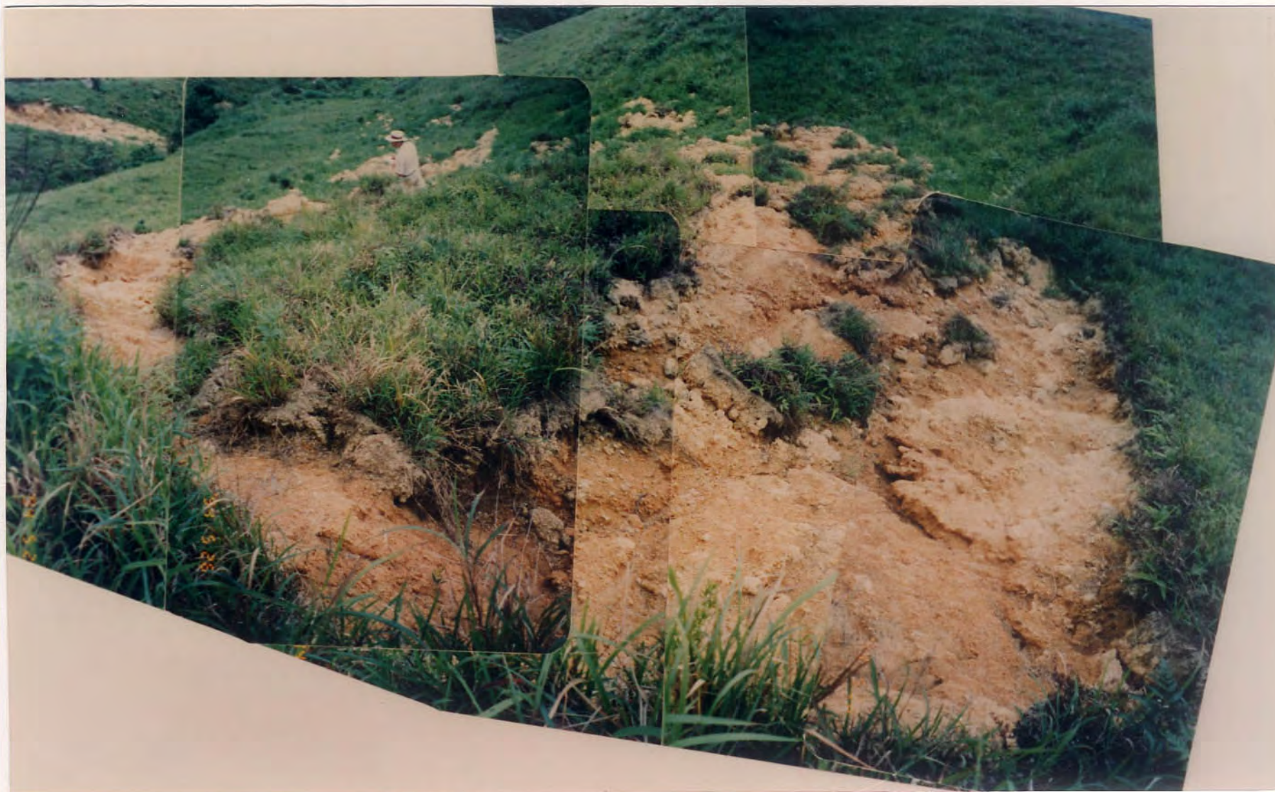
Plate A6.6 - Downhill View of Landslide Scarp A6
