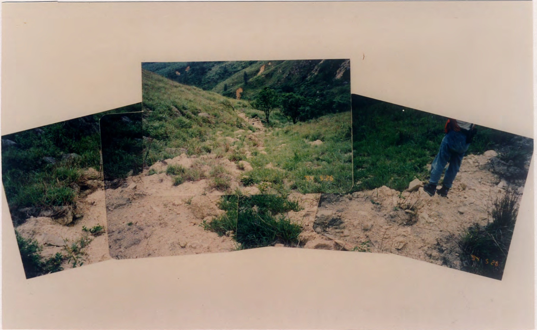
Plate A4.3 - Downhill View of Debris Trail from Landslide Scarp A4
