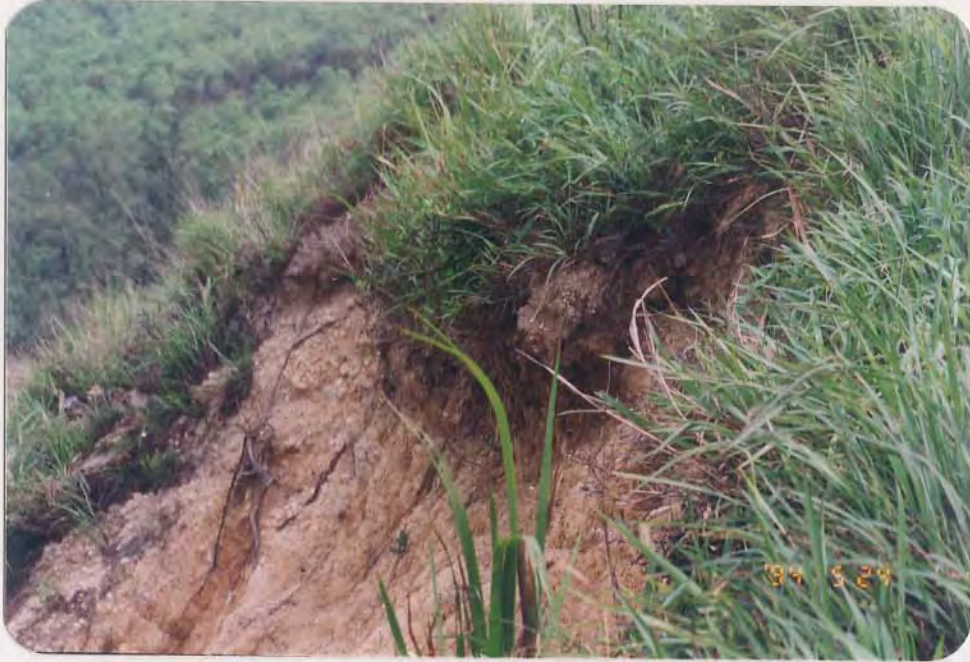
Plate A9.3 - Close-up of Minor Landslide Adjacent to Footpath
