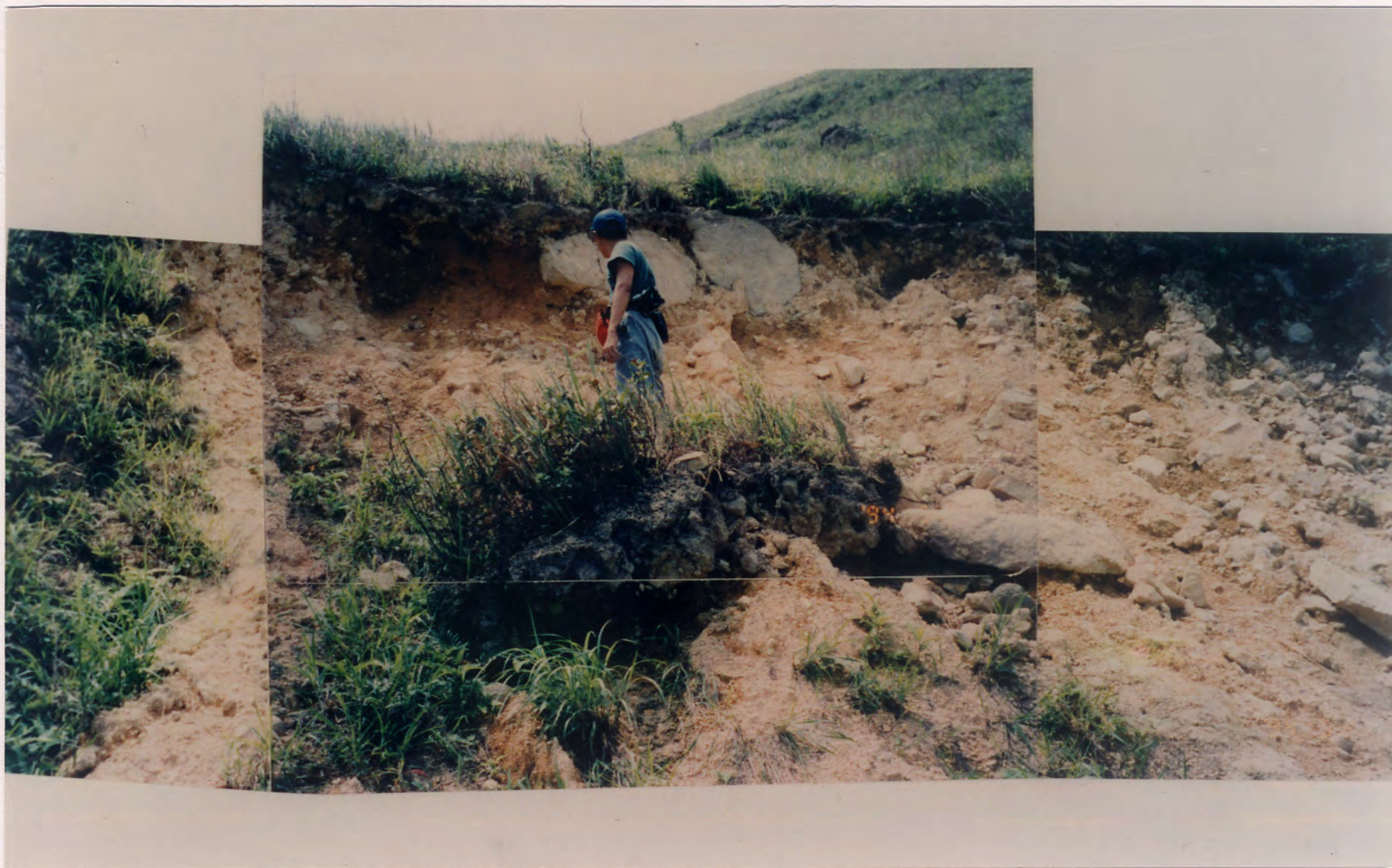
Plate A3.5 - Close-up of Main Scarp of Landslide A3
