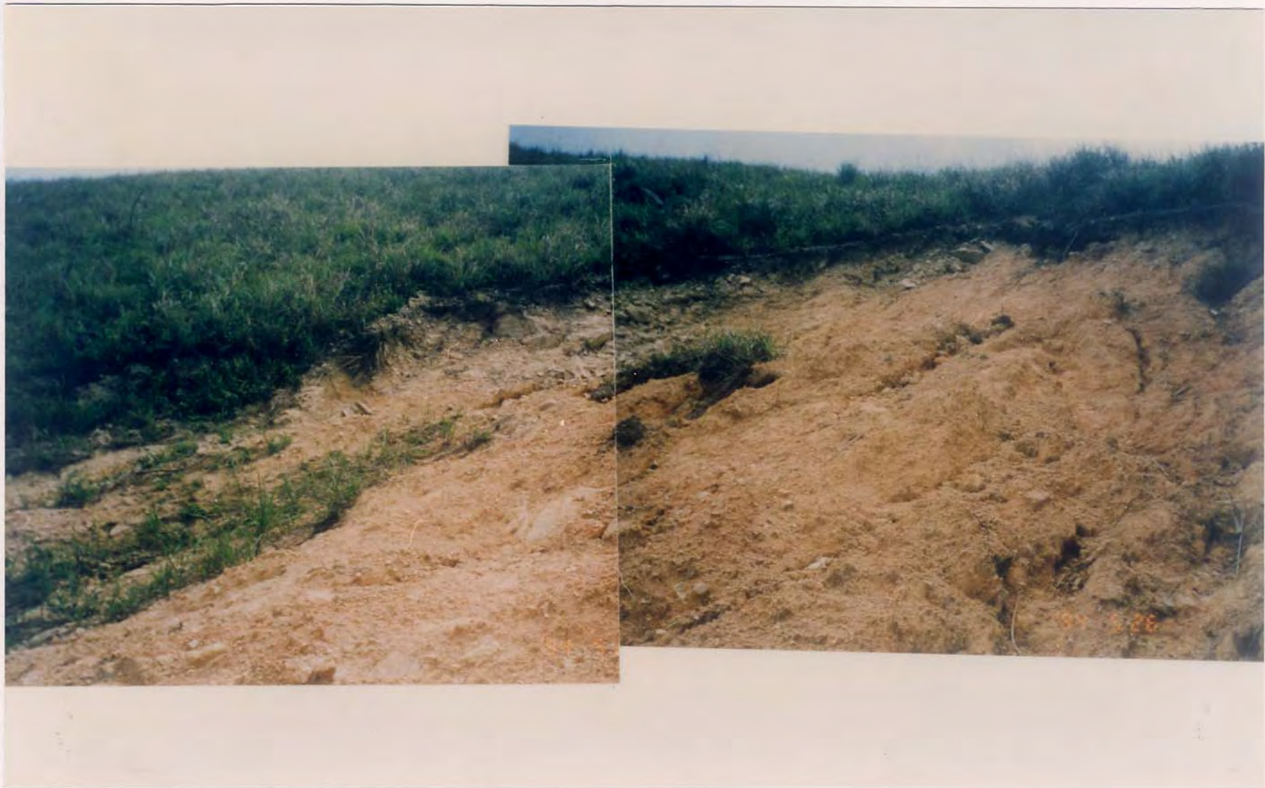
Plate A16.9 - Close-up of Landslide Scarp A16B
