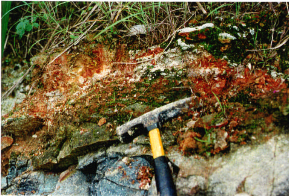
Plate 7 - Close-up of Exposure Shown in Plate 6, Showing Kaolinitic Clay Development along the Outward-dipping, Planar PW0/30 and PW90/100 Rock Mass Weathering Zone Interface (843478 813884), Slope 11SE-D/C187, Northwest of Siu Sai Wan Estate (Taken 24/7/96)
