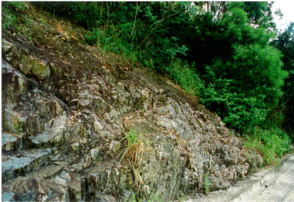
Plate 8 - General View of Outward-dipping, Planar PW0/30 and PW90/100 Rock Mass Weathering Zone Interface (843510 813932), Associated with Kaolinitic Clay Development, Slope 11SE-D/C187, Northwest of Siu Sai Wan Estate (Taken 24/7/96)
