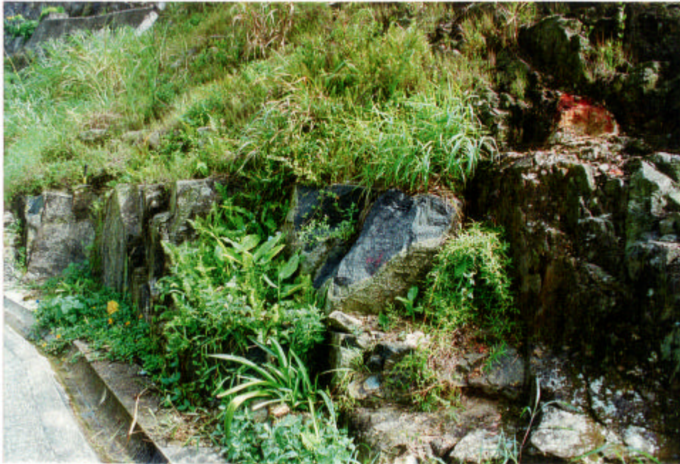
Plate 10 - General View To South, of the PW0/30 Zone Containing the Kaolinitic Clay-infilled Joint Shown in Plate 11, with Occasional, Large, Joint-bounded Cores Comprising Tuff, Predominantly of Weathering Grade II (Taken 24/7/96)
