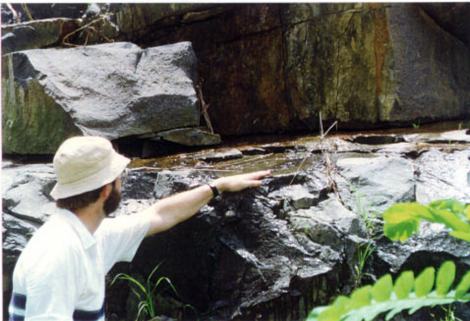
Plate 21 - Extensive Seepage from Shallowly-inclined Joint ( 84430 813690) Dipping Outward from Slope 11SE-D/C181, Southeast of Siu Sai Wan Estate (Taken 26/6/96)
