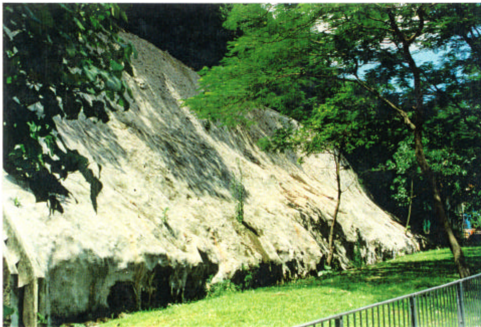
Plate 19 - Oblique View of Slope 11SE-D/C41, Looking Southwest, on the South Side of Fei Tsui Road, Showing Concavity in the Shotcreted Slope Approximately Coinciding with the Outward-dipping PW0/30 and PW90/100 Rock Mass Weathering Zone Interface. Eutaxitic Fabric also Dips Outward in Exposed Rock near the Slope Base (Taken 5/7/96)
