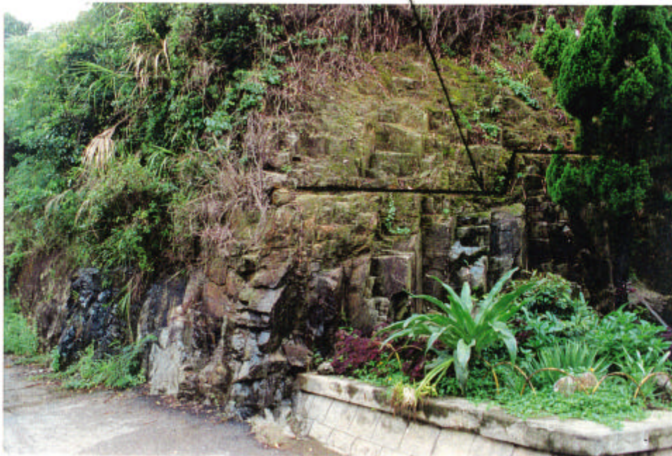
Plate 16 - A Wide, Weathered, Shallowly-inclined Joint in Slope 11SE-D/C98, West Side of Cape Collinson Road. The Joint Infill is of Completely Decomposed Tuff and Kaolinitic Clay. The Joint Locally Steps and Bifurcates across Subvertical Joints (Taken 15/7/96)
