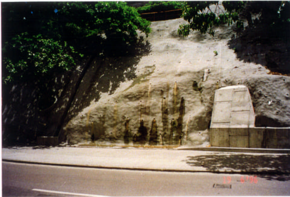
Plate 20 - Seepage from Weepholes in Shotcreted Slope 11SE-D/C17 on the Southeast Side of San Ha Street. Several Small Landslides (Map No.3) have Occurred along this Slope which is a Modification of the Pre-reclamation Cliff Line (Taken 19/6/96)
