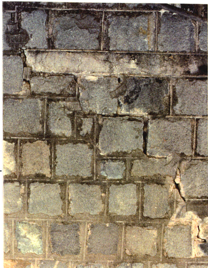
Plate 7.8 - Example of Crack Origin Diagnosis - Retaining Wall at Hok Size Terrace (I)
